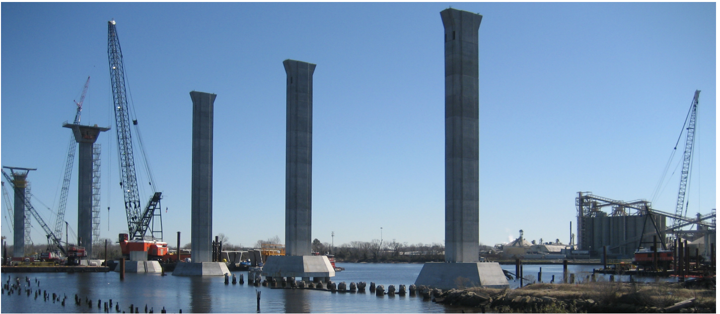
Figure 5. Construction of the South Norfolk Jordan Bridge at the Atlantic Wood Industries, Inc. site and across the Southern Branch of the Elizabeth River (Virginia).
