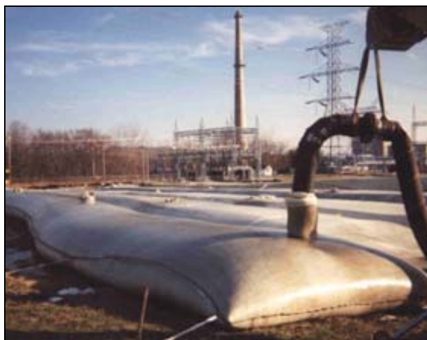
Figure 4-8. Geotextile Tube Filled with Dredged Sediment (Used with permission from Ellicott Division of Baltimore Dredges, LLC, Baltimore, MD 21230)
