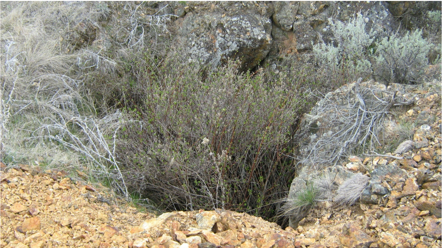
SMM Sealed Mine Workings Vent on Slope Above Adit from the South
