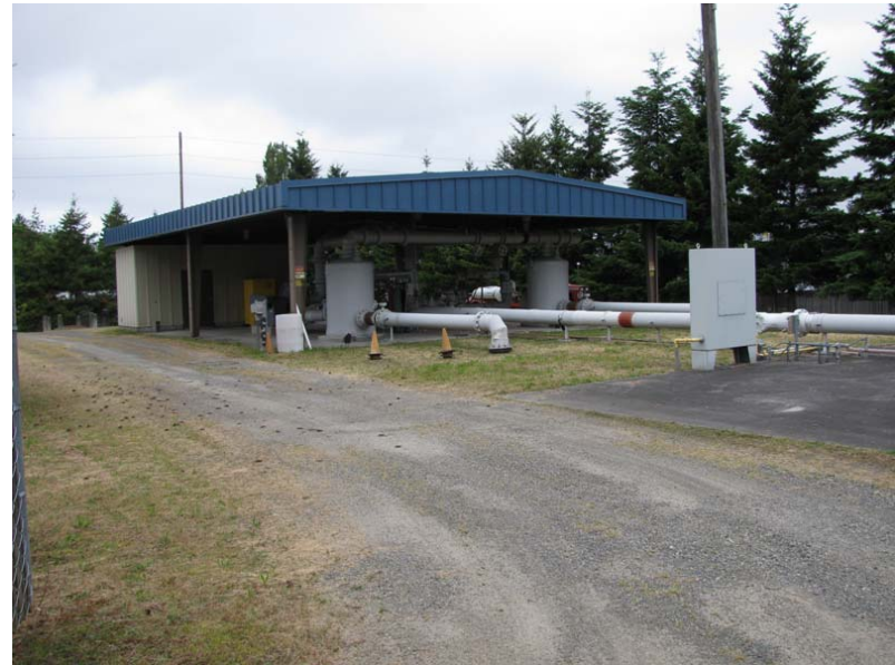
Gas extraction system mechanical room.
