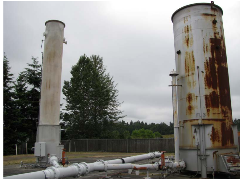
Gas extraction system flares. Current flare on left, backup flare on right.
