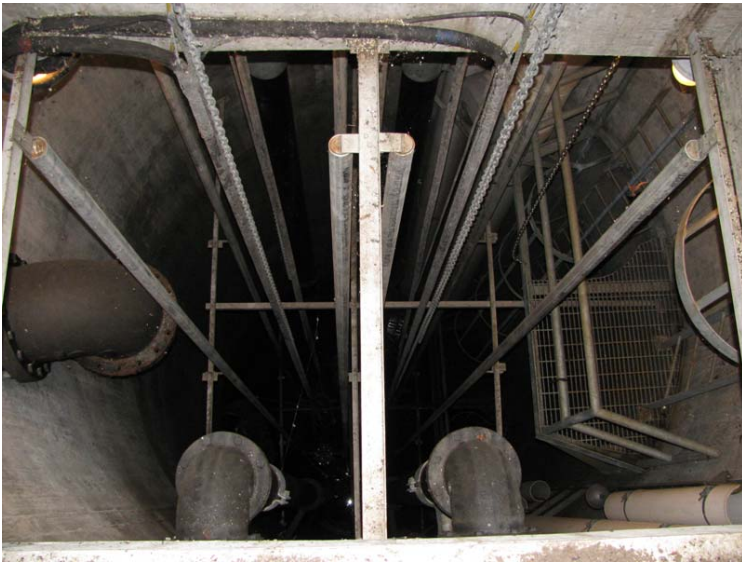
Linda Heights Park storm water diversion pumps.
