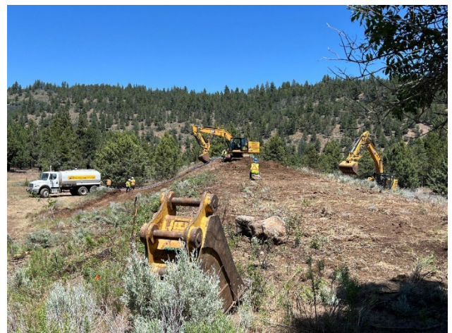
Figure 4: Time-critical removal action within the Rifle Range 300-yard firing line (OU2-RR-BB2) in 2024.
