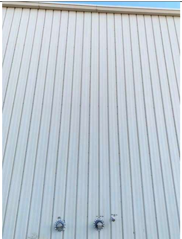
Leaking gutter with location of leak and drip path
