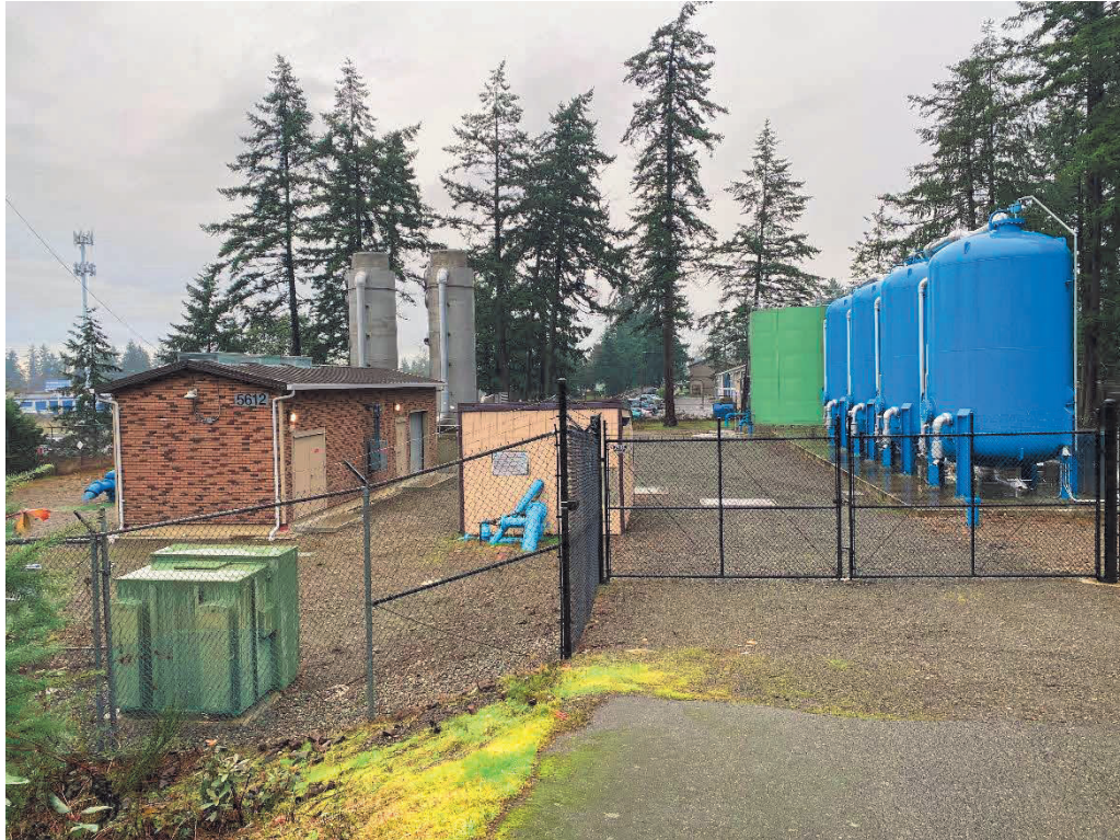
Lakewood Water District treatment facility
