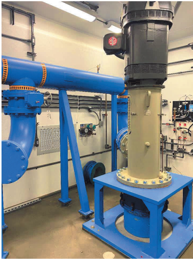
Treatment plant interior
