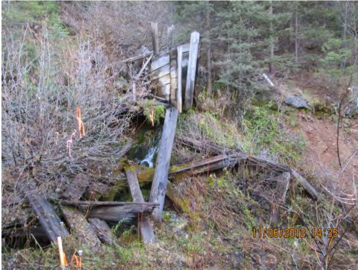
Figure 11A. Photo of the Bailey Tunnel Adit (YP-AS-2) from the Surface Water Quality Baseline Study, Appendix G, November 2012 Site Photos, page 14. Photo caption reads, “YP-AS-2, Bailey Tunnel outlet. Close-up looking south and upstream at seep source. November 2012.”
