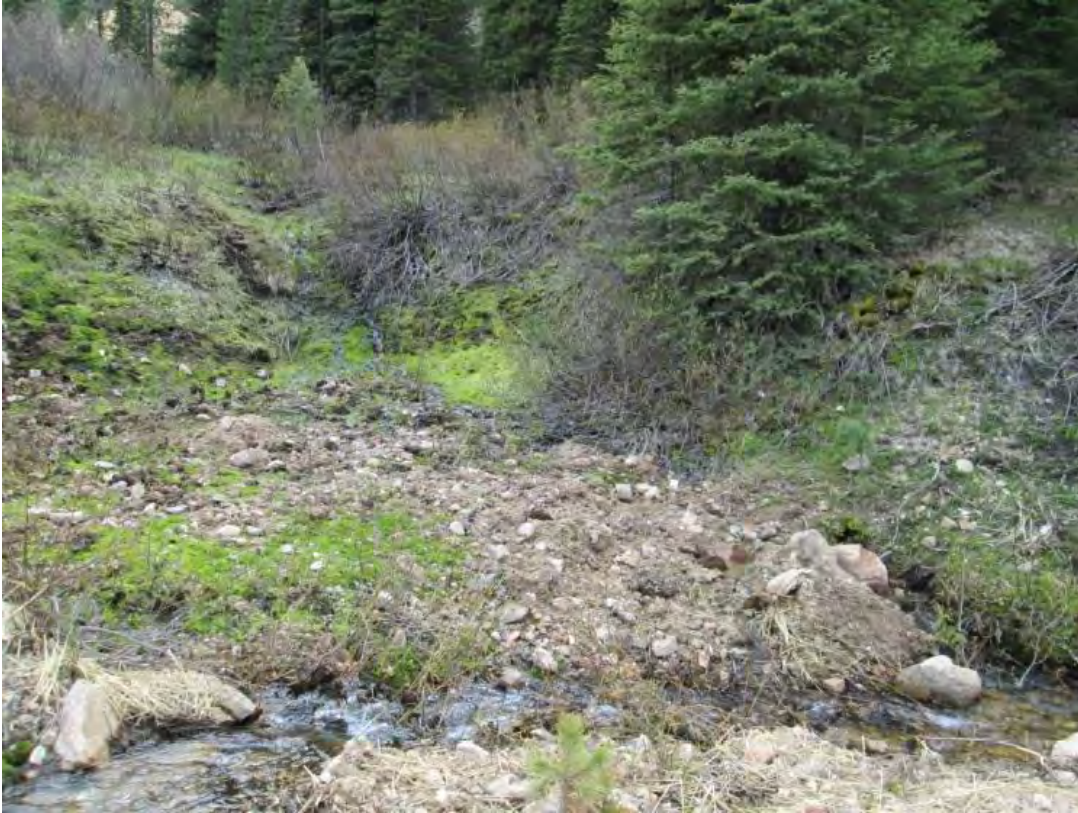
Figure 14D. Photo of the DMEA Wasterock Seep (YP-T-17) from the Surface Water Quality Baseline Study, Appendix G, May 2012 Site Photos, page 15. Photo caption reads, “YP-T-17, DMEA wasterock seep. Looking west and upstream, with DMEA wasterock dump visible in back left, and tributary at front, May 2012.”
