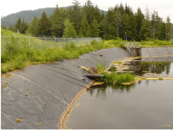
Photo 37. Geomembrane lined sediment lagoon at the KPC landfill. Note six foot chain link fence surrounding lagoon. Inlet pipe.
