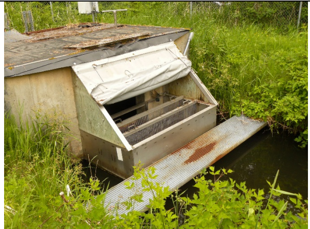
Photo 42. Outflow/ discharge point for landfill lagoon. APDES sample point of compliance.
