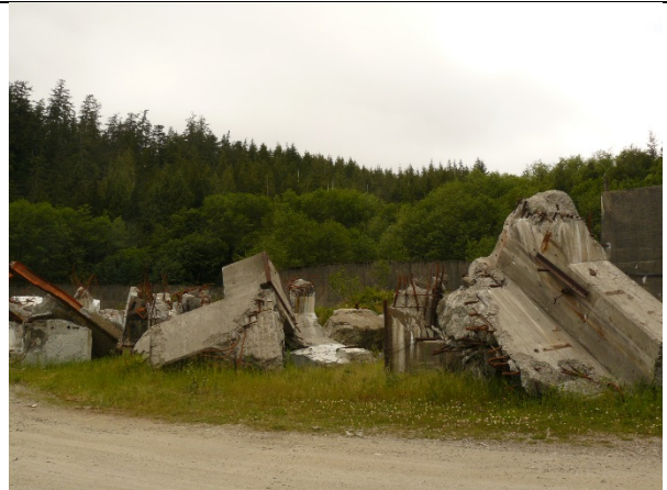
Photo 30. Former KPC Building rubble on site. Aeration basin secondary clarifiers in background.
