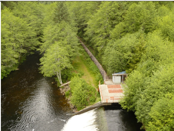
Photo 53. Wood pipeline carries water 3.1 miles to KPC mill site
