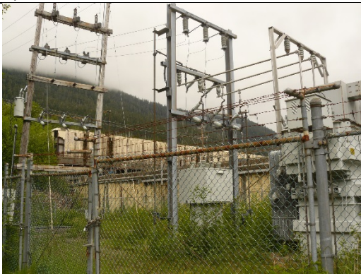
Photo 3. View of abandoned power substation, northeast of administration building. Yellow building in background is former KPC Filter Plant and can be seen from North Tongass Highway.
