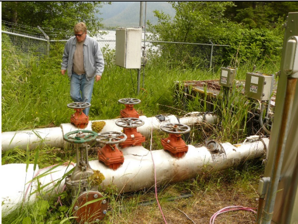
Photo 41. Flow pumps for KPC landfill lagoon.
