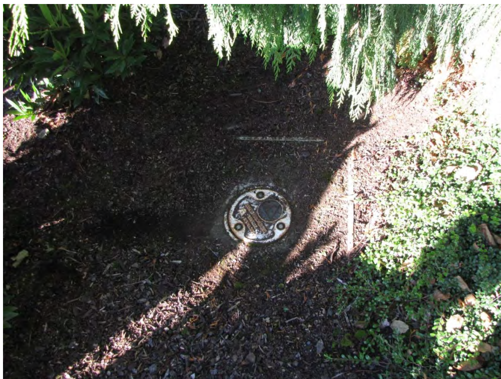
Photo 4. Monitoring well RW97-18A.
