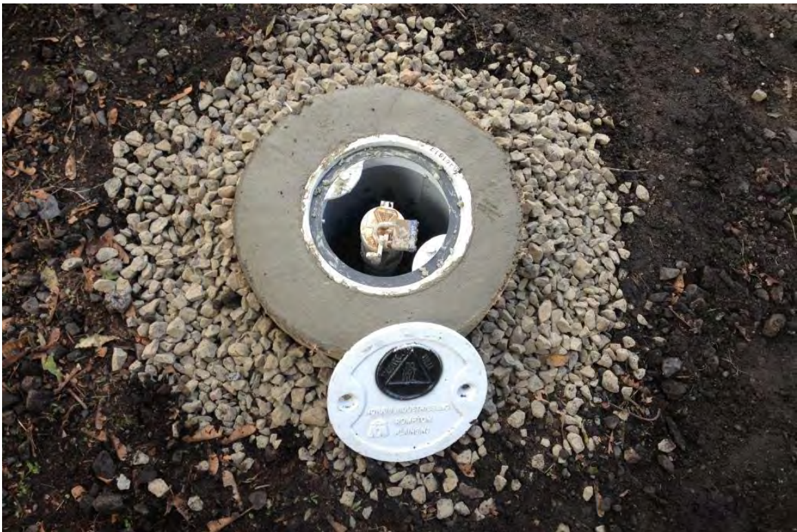
Photograph 9 - MW-58 well cluster repairs completed in 2013 without making modifications to the existing well casing heights.
