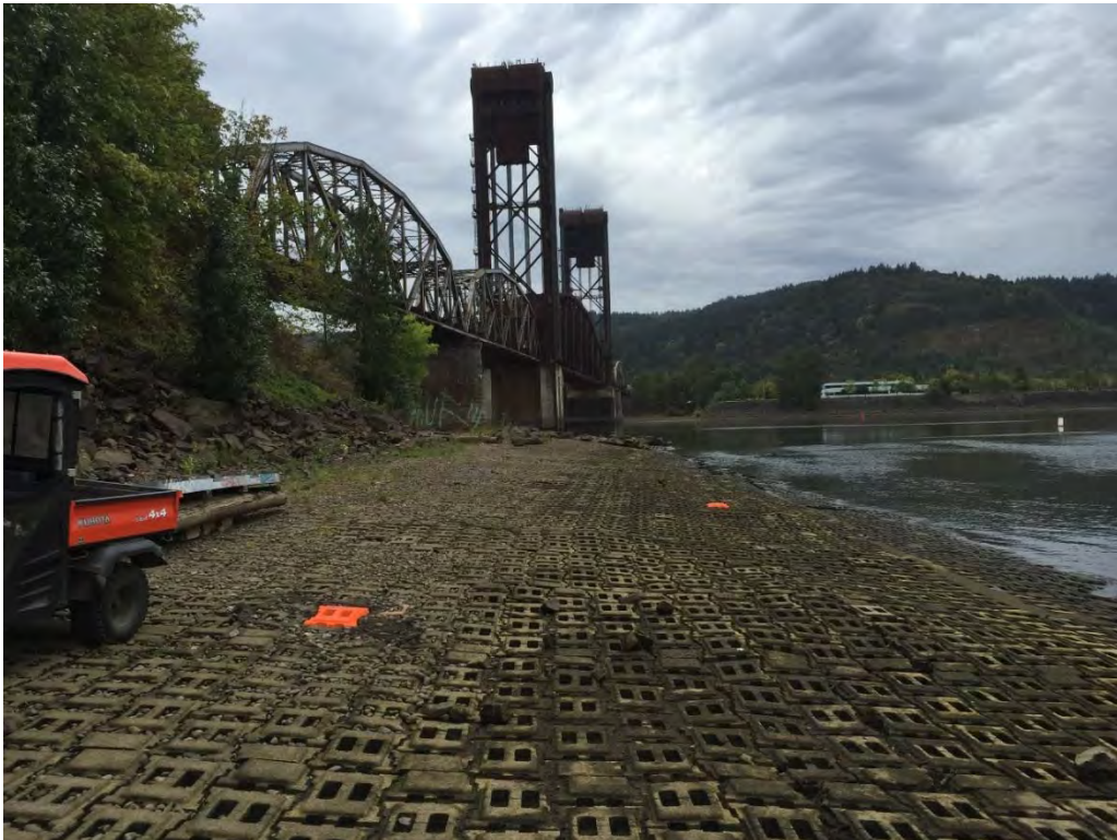
Photograph 5 – Willamette Cove sediment cap ACB blocks (bright orange) replaced following September 2015 organoclay sampling.
