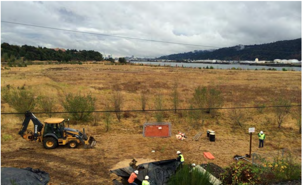
Photograph 8 - Overview of the Site during Northwest Natural gas line decommissioning in 2014. Photograph taken facing south.
