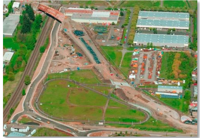
Figure 12. Completed Minuteman Way and ongoing construction of the Sunrise Corridor. (Source: ODOT)
