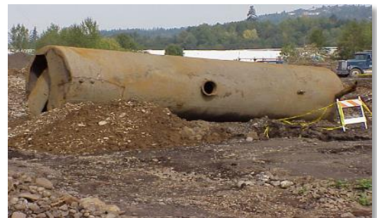
Figure 3. One of the two 10,000-gallon tanks on site prior to disposal in 2001.
