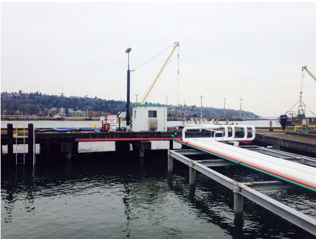
Photo 4. BP Terminal continuation of photo 2 showing on-loading and off-loading petroleum fuels piping and dock at West Waterway looking westward in distance is the north edge of West Seattle.
