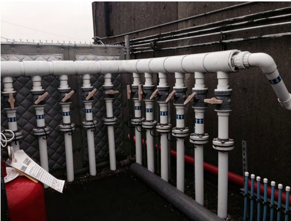
Photo 8. BP Terminal detail for the Soil Vapor Extraction Remediation System showing 11 individual well control valves and piping. Blue airlines to right were installed as a contingency in case additional remedial technologies, such as air sparging, would be needed to meet site cleanup objectives. This system is removing petroleum vapors from soil and groundwater for subsurface cleanup action.
