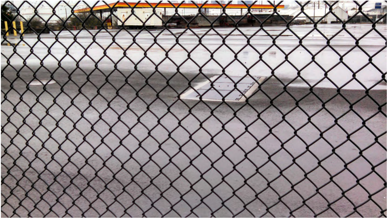
Photo 10. Stormwater treatment access vault
