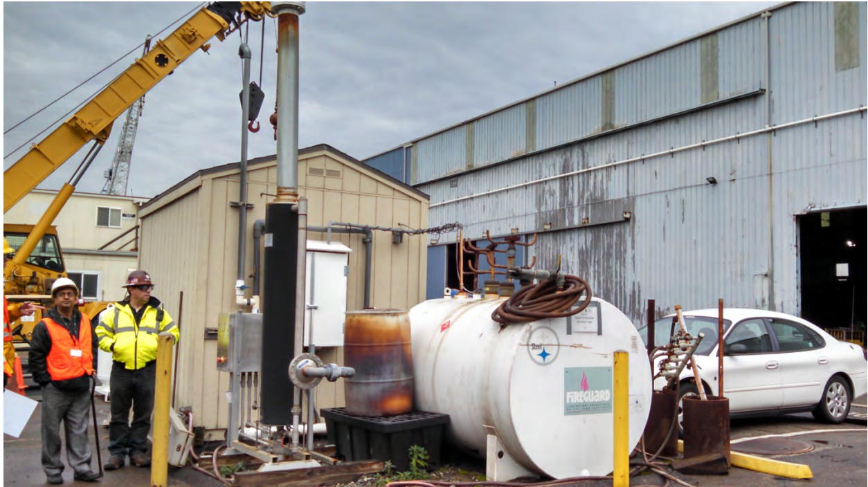
Photo 18. West LNAPL Shed LNAPL tank and catalytic oxidizer
