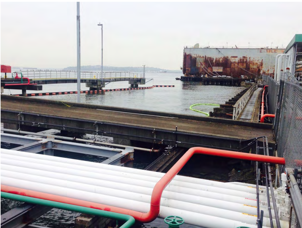
Photo 2. BP Terminal seawall parallel to loading rack on right, green boom to capture any sheen or floating product on West Waterway is a safety measure. Foreground is piping for on-loading and off-loading petroleum from barges or ships at West Waterway. Left is barge and ship dock with Elliott Bay is in background.
