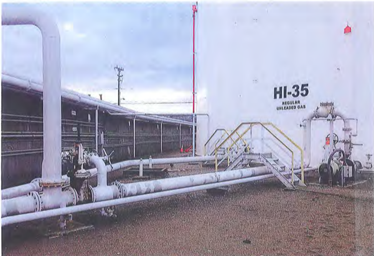
Photo 4. KMLT Above ground petroleum Storage Tank No 35 at E Yard with supply piping and valves.
