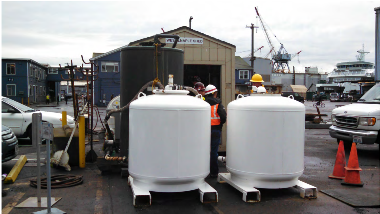
Photo 17. West LNAPL Shed carbon vessels
