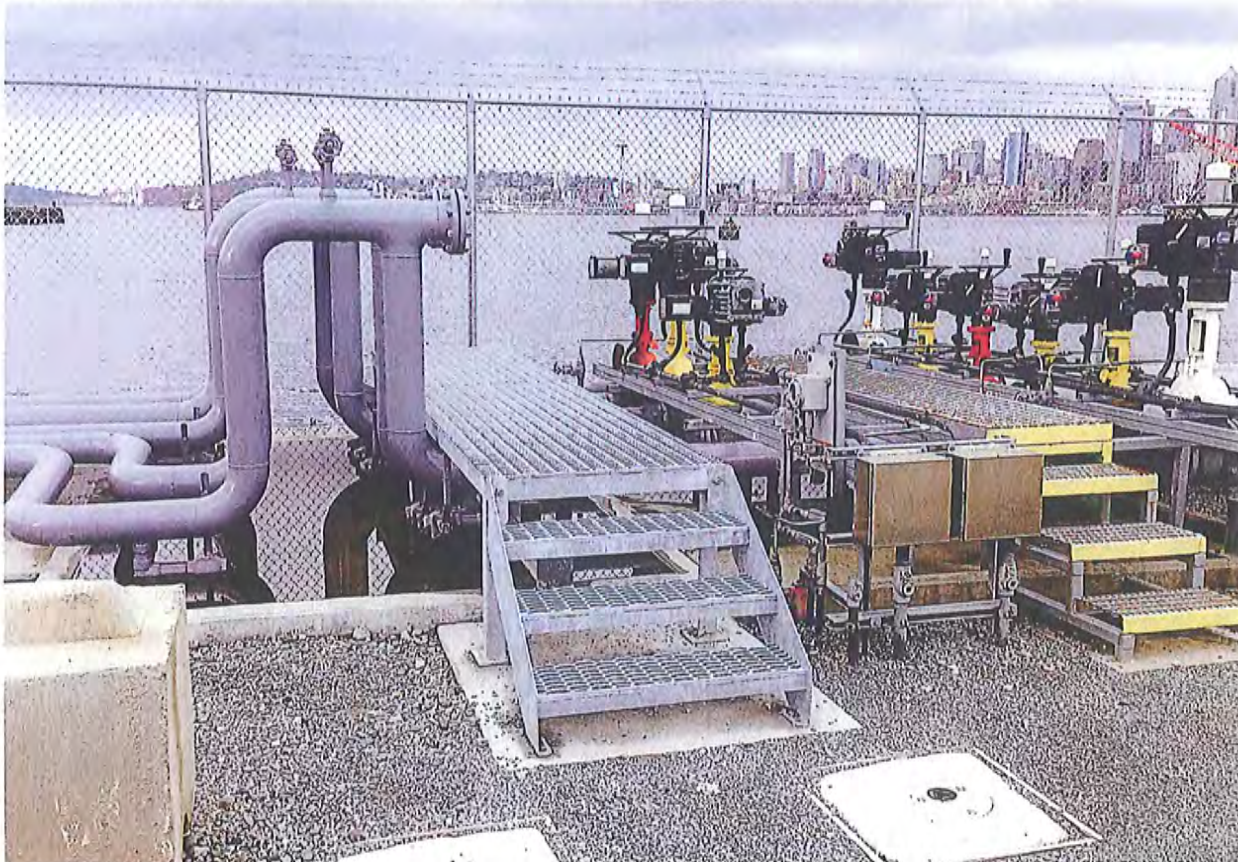
Photo 2. Shell Harbor Island Terminal Shoreline Manifold Area looking northeast across Elliott Bay to City of Seattle in background.
