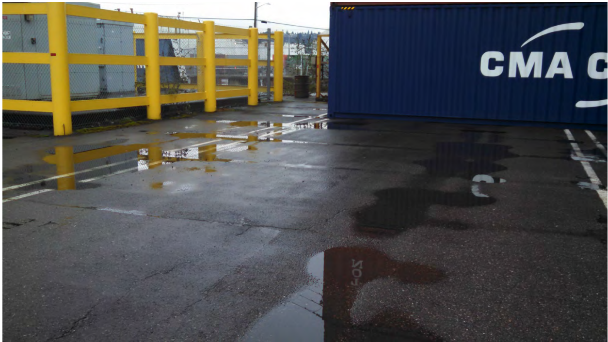
Photo 3. Capped area – standing water
