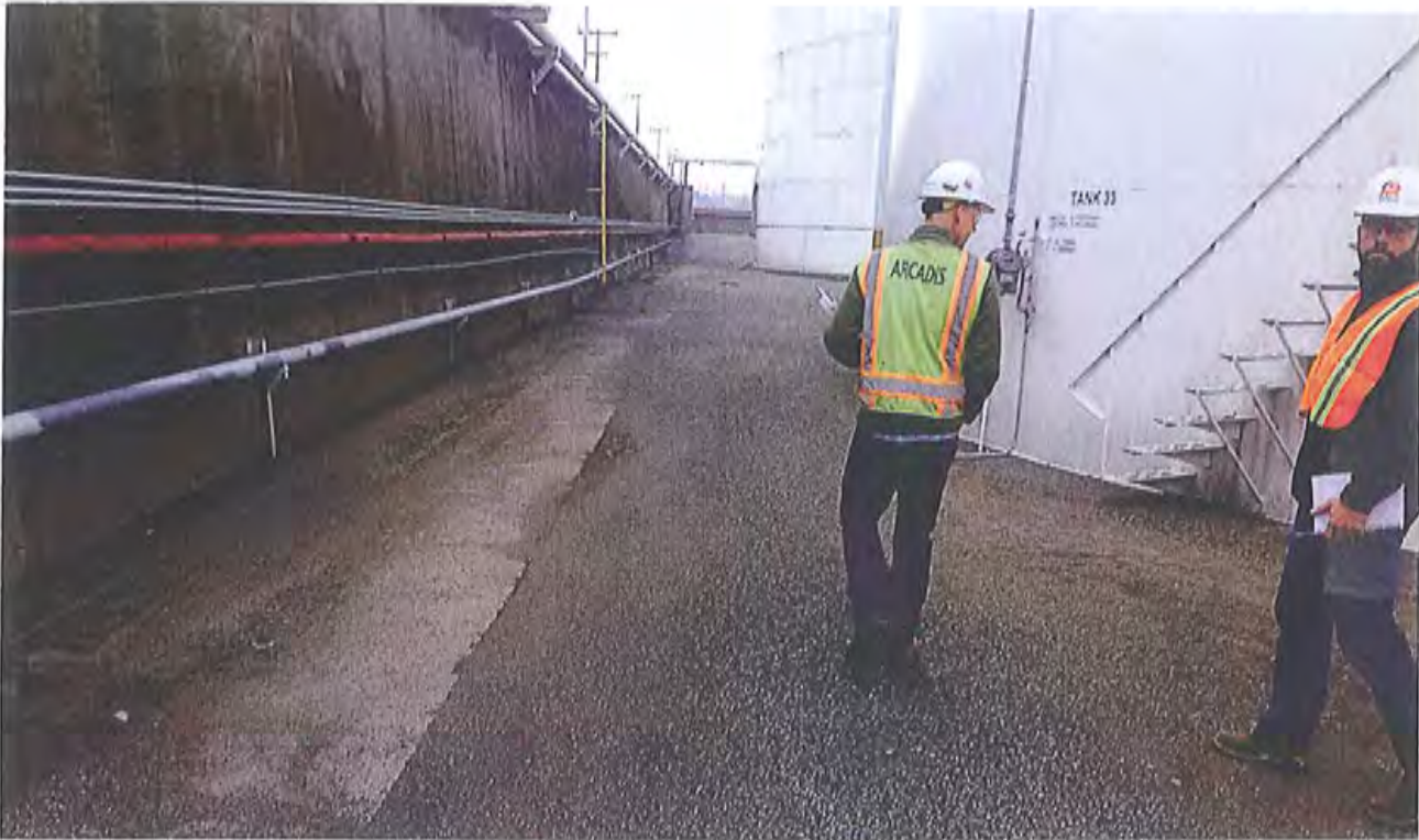
Photo 3. KMLT Above ground petroleum Storage Tank No. 33 at B Yard with containment wall and piping on left with two Arcadis consultants conducting the site inspection.
