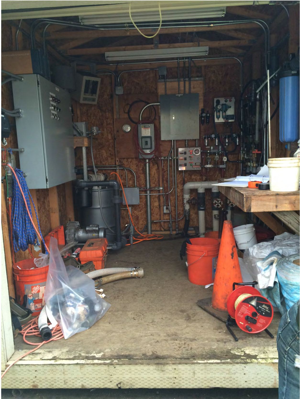
Photo 16. West LNAPL Shed controls
