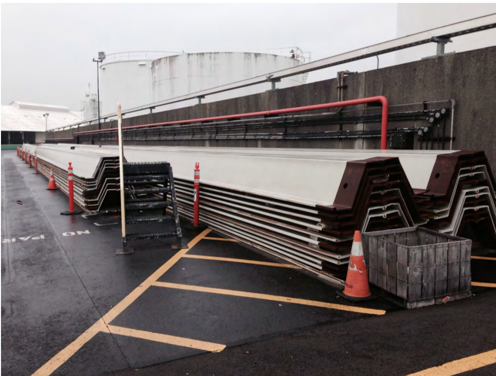
Photo 10. BP Terminal outside south wall for Plant 1 where new materials for new seawall are temporarily stored and waiting permit approval to replace West Waterway seawall and AST No. 9 and 13 in background.
