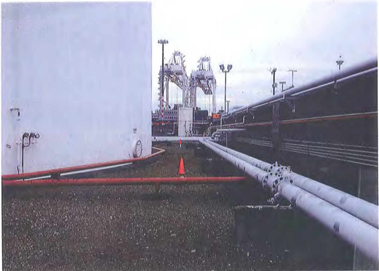
Photo 6. KMLT Above ground petroleum Storage Tank and supply piping with containment wall to right.
