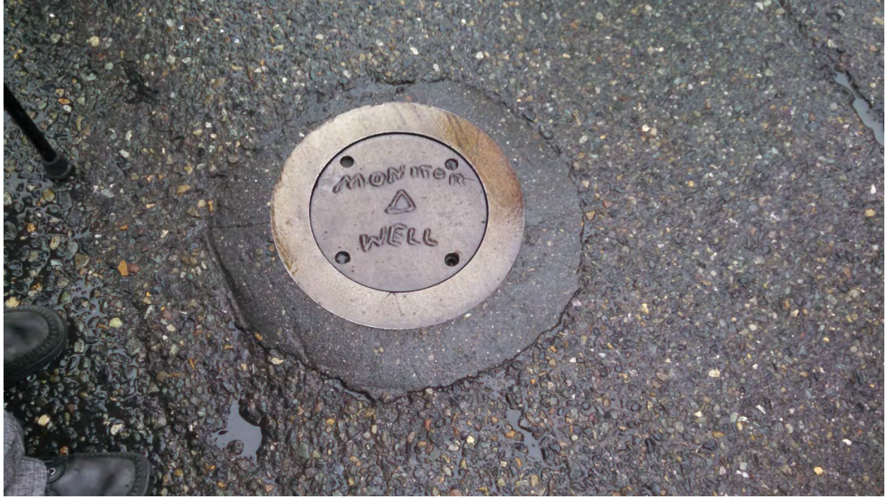
Photo 5. Monitoring well HI-3 (bolts missing)
