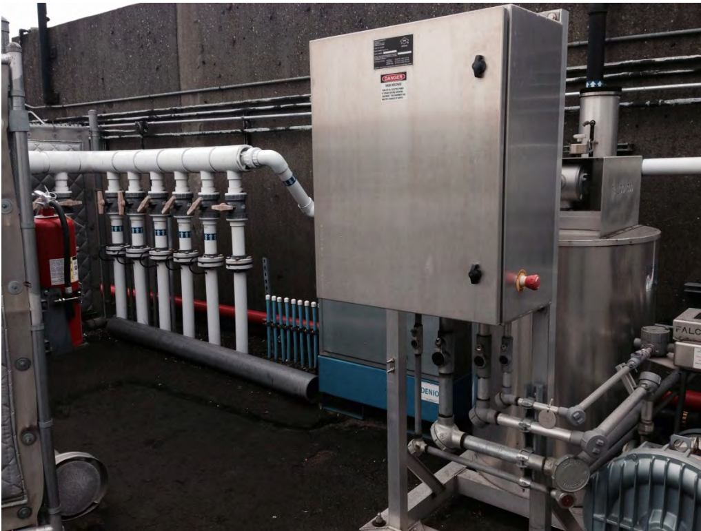
Photo7. BP Terminal Soil Vapor Extraction Remediation System equipment is shown with pumping station, vapor removal and stripping system and six individual well piping with control valves. This system is removing petroleum vapors from soil and groundwater for subsurface cleanup action.
