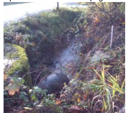
Photo 1 Belfair Valley Road 36 IN Culvert crosses the roadway at the Winner's Circle Bar and Grill
