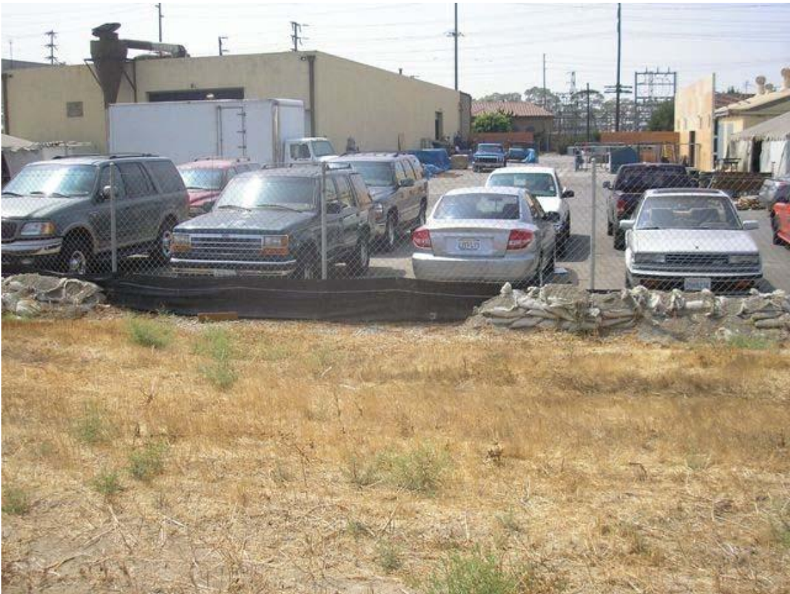
Photo 12: Storm Water Control – Sand Bags and Silt Fence, South Side of Site
