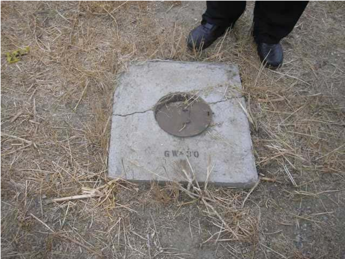
Photo 3: GW-30, Minor Surface Damage – Pad cracked, security lid damaged and unsecured
