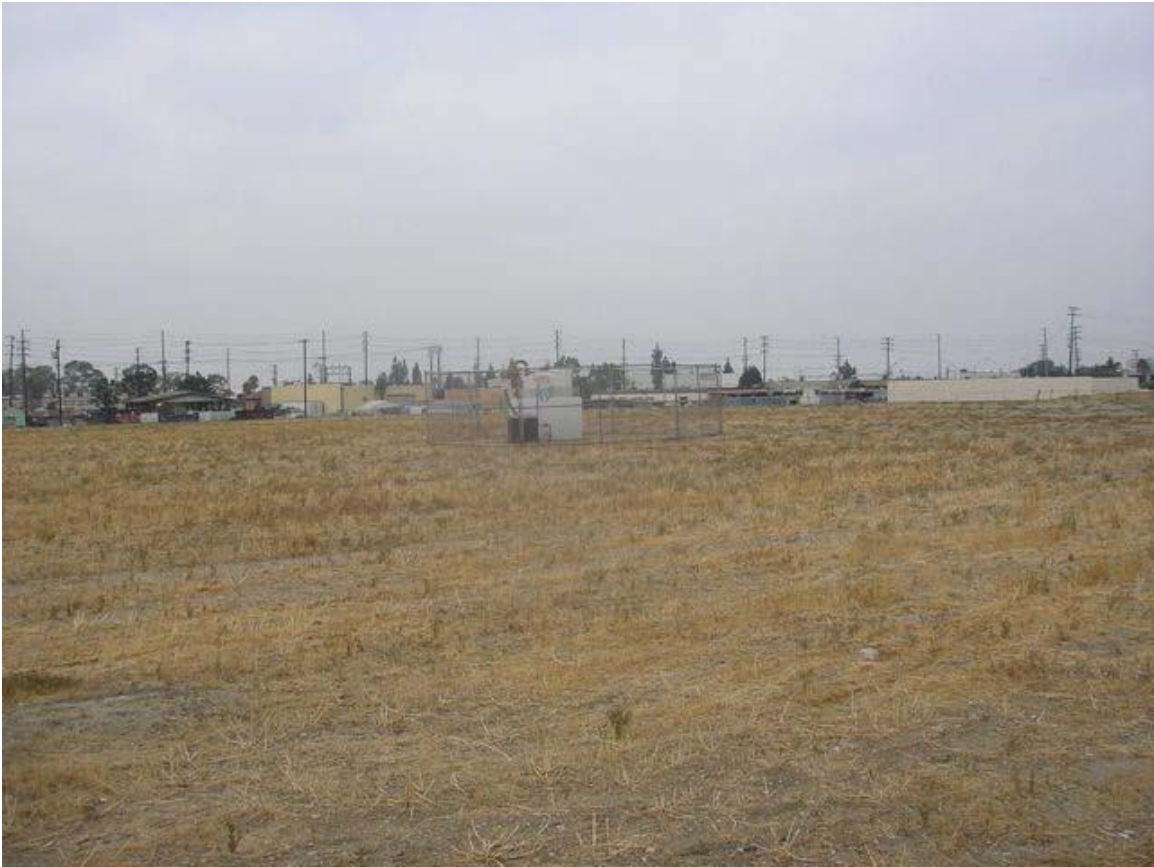
Photo 7: Leachate Collection Well, LC-2
