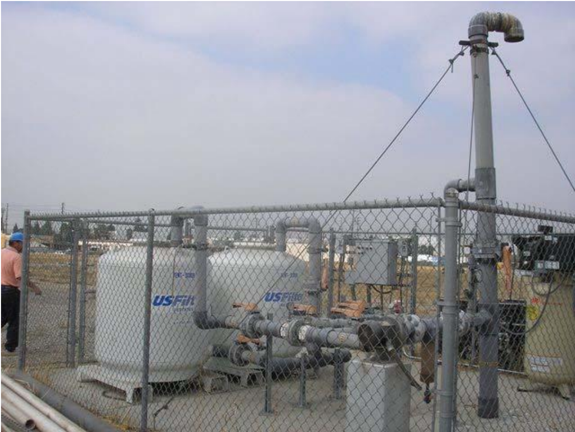
Photo 9: SVE System, Currently in Passive Operation
