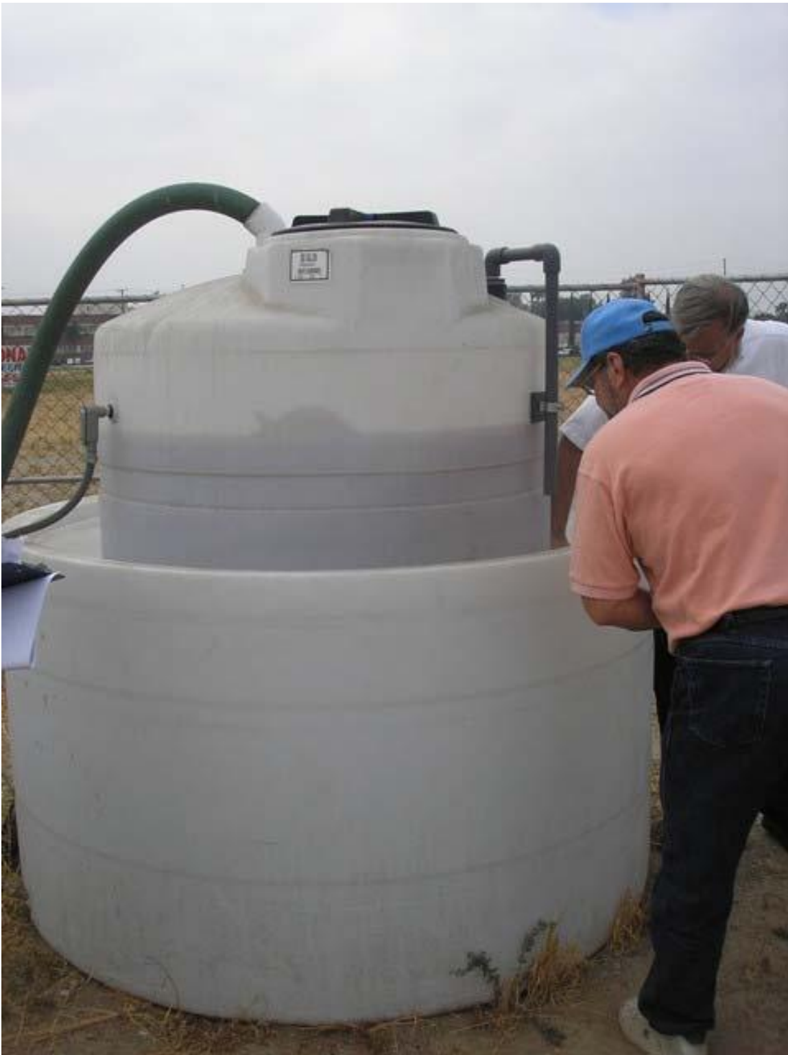
Photo 8: Examining Automated Leachate Collection System at LC-2
