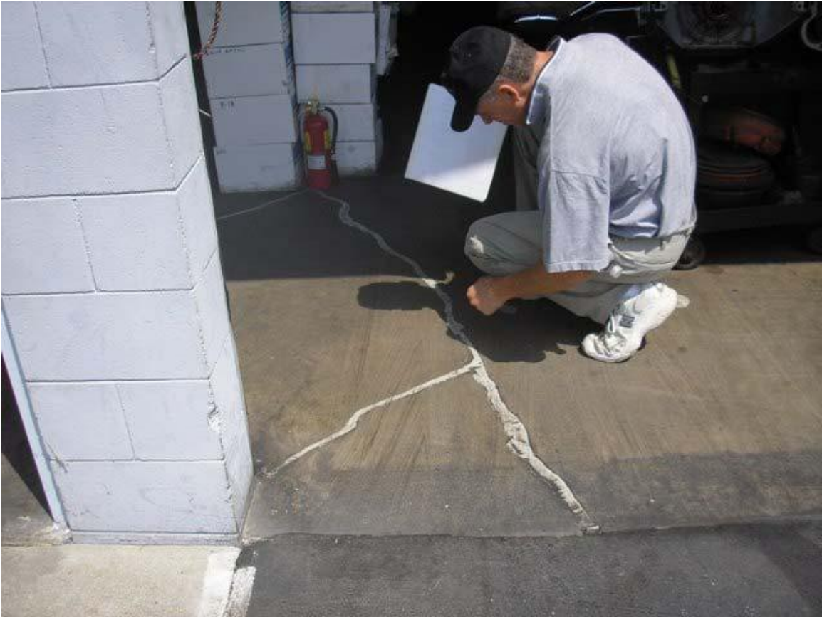
Photo 14: Sealed Cracks in Pavement at Small Business (“Four C’s Transmission”), South Side of Site
