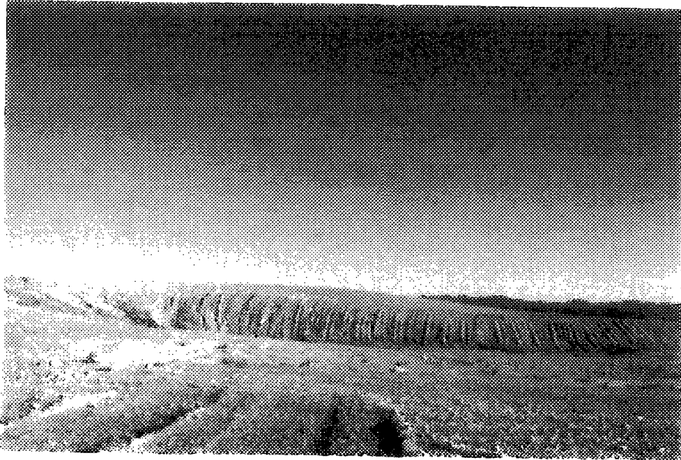
SW-24 LOOKING EAST SOUTHEAST AT EROSION ON FACE OF PRE-91 COVER IN SOUTHWEST CORNER
