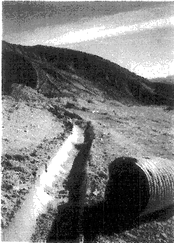
KB-7 LOOKING EAST SOUTHEAST ALONG EXISTING HALF-PIPES - bent, partially sedimented, poor joints, undermining at edges
