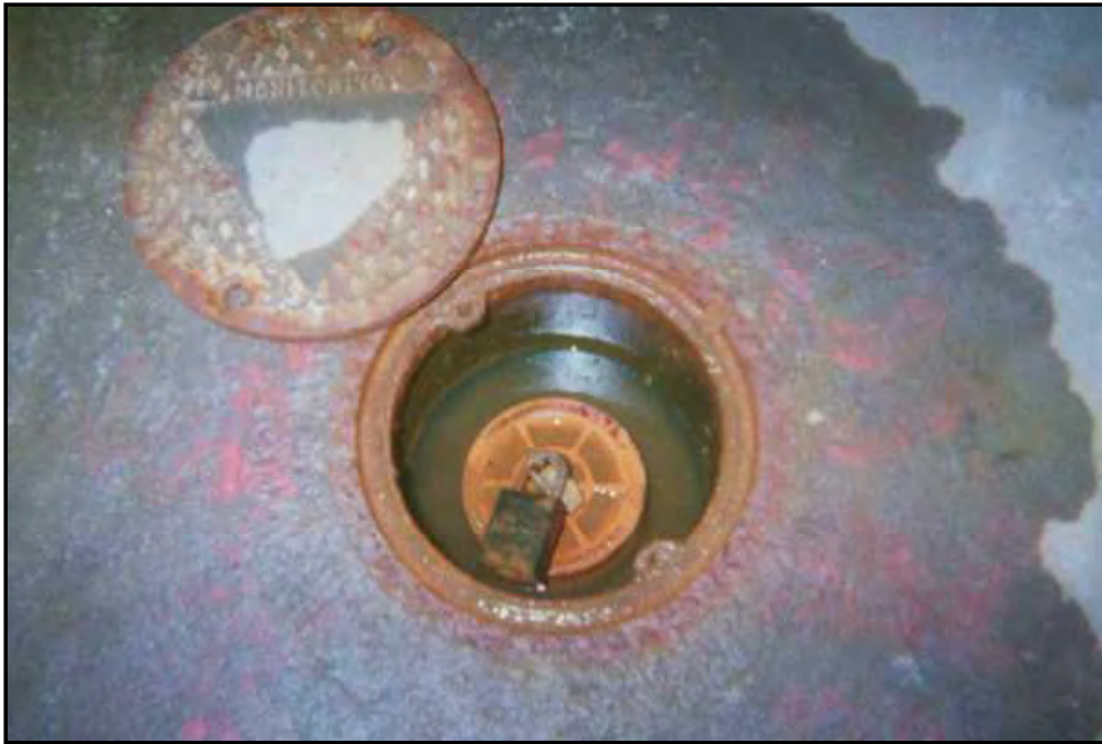
Photograph D-15. Well IR10MW59A; padlock on well and standing water in vault.
