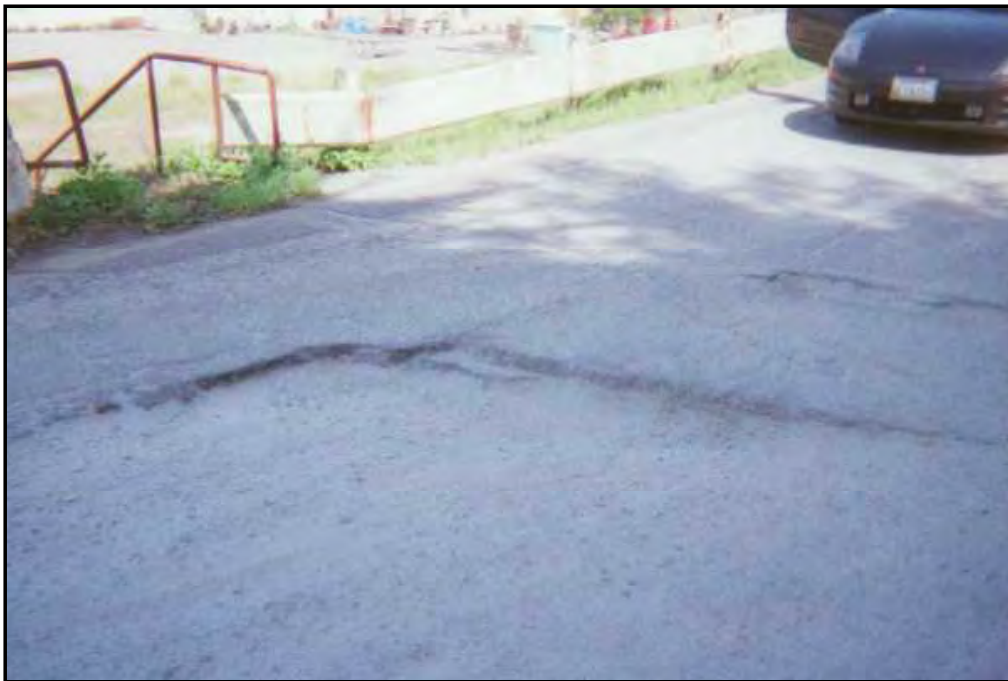
Photograph D-33. Large pothole in road on Parcel B near Building 104; extreme example of potholes observed throughout Parcel B roads.
