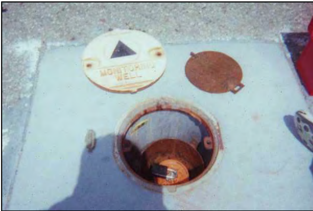
Photograph D-1. Well IR06MW42A; padlock on well and new concrete associated with vault.
