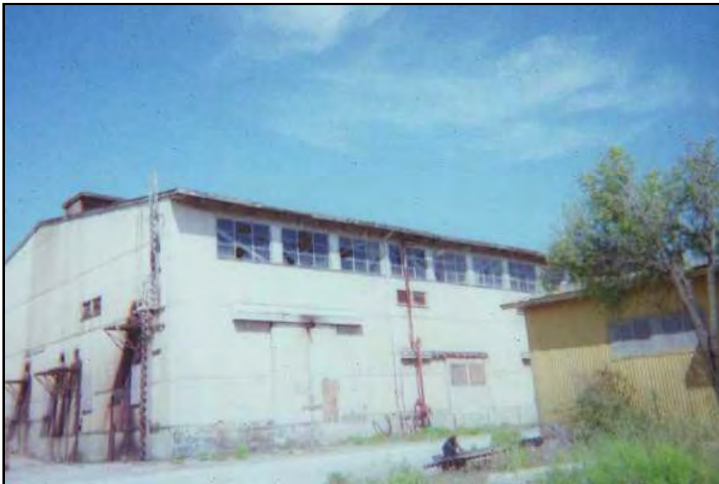
Photograph D-32. Broken windows on Building 123; representative of broken windows on abandoned buildings throughout Parcel B.
