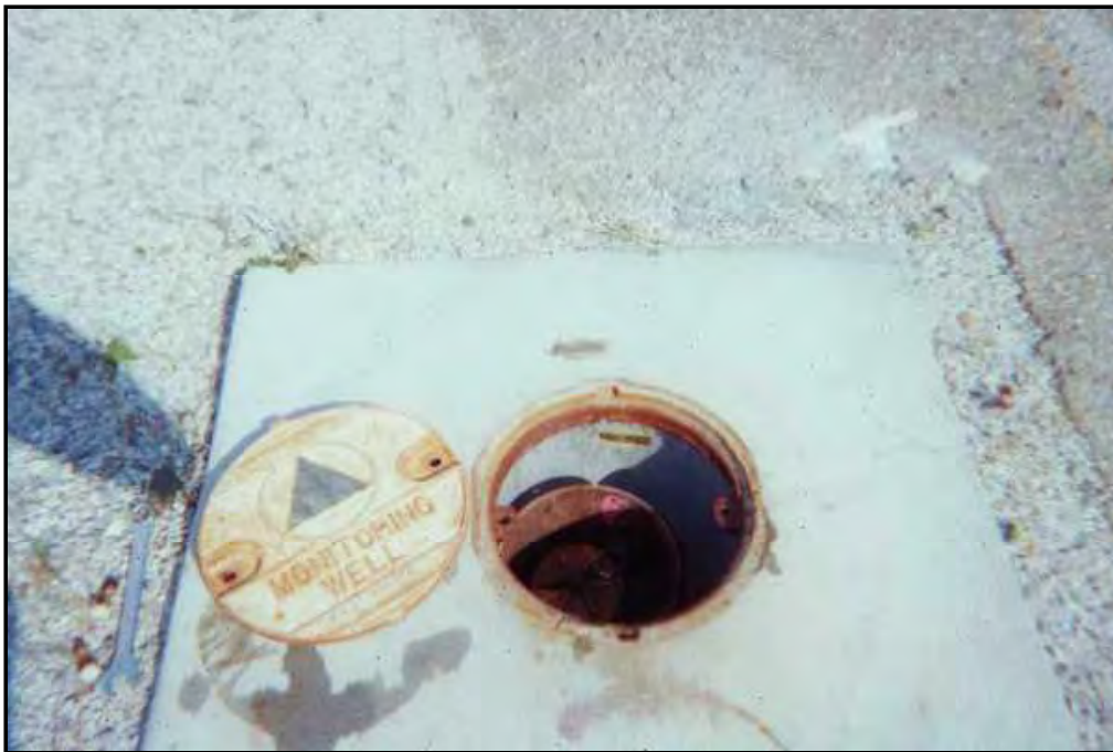
Photograph D-17. Well IR25MW17A; padlock on well and new concrete associated with vault.
