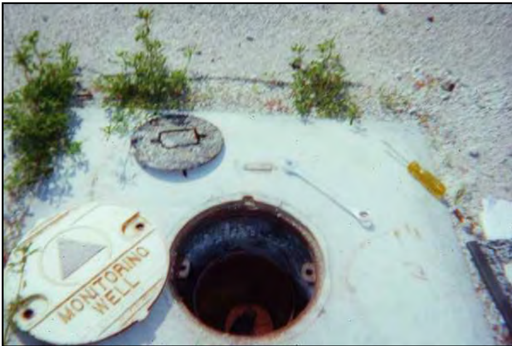
Photograph D-23. Well IR46MW37A; padlock on well and new concrete associated with vault.
