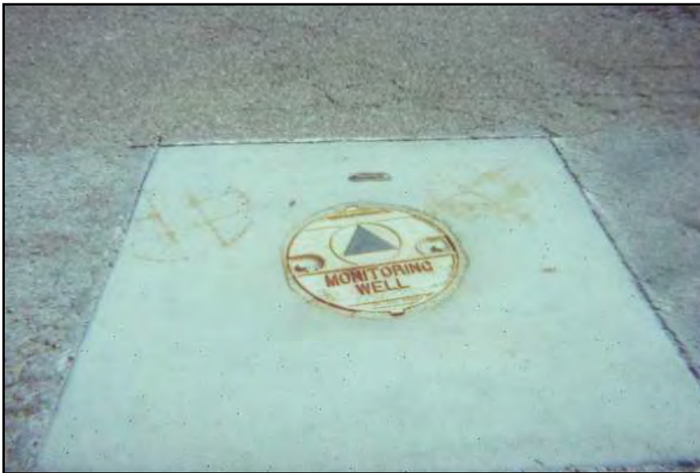
Photograph D-11. Well IR10MW14A; note new concrete associated with vault. Orientation: North Date: May 13, 2003
