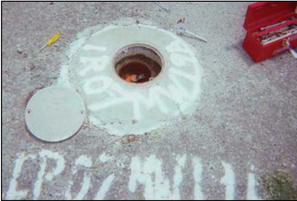
Photograph D-3. Well IR07MW19A; padlock on well and standing water with rust in vault.
