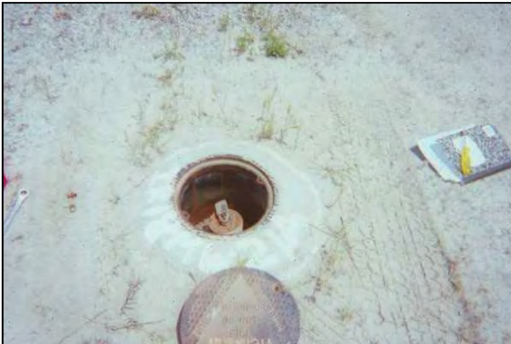
Photograph D-16. Well IR18MW21A; padlock on well and standing water in vault.
