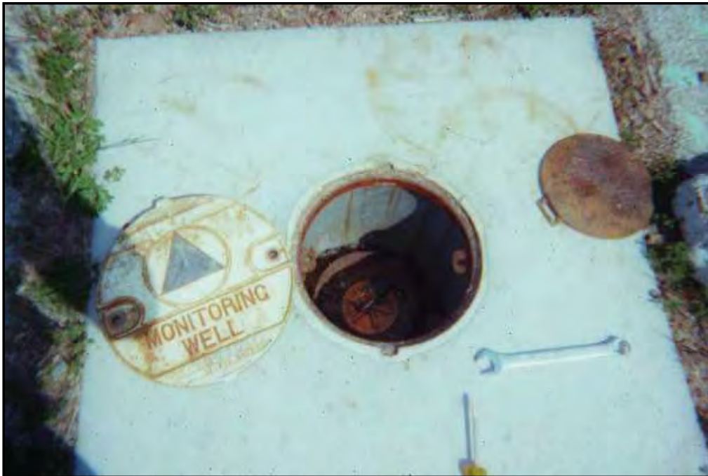
Photograph D-4. Well IR07MW20A1; padlock on well and new concrete associated with vault.
