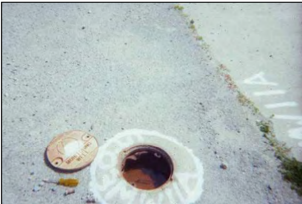
Photograph D-26. Well UT03MW11A; padlock on well and standing water in vault above wellhead.
