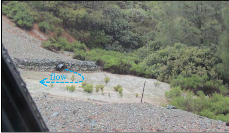
Photo 18. Ponding at Atlas Chanel B Energy Dissipater; volunteer vegetation present.
