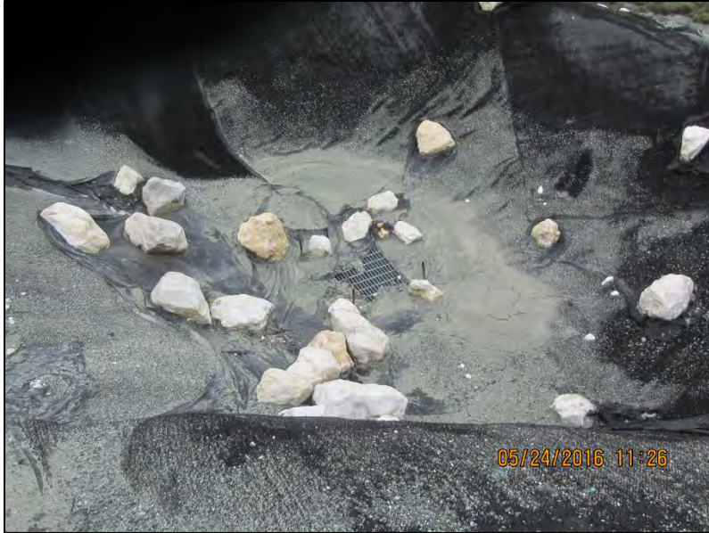
Photo 16. Sedimentation at Drainage Outlet near Atlas Sediment Storage Area.
