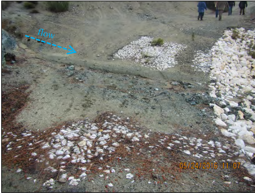
Photo 9. Drainage across Road to Atlas Rover Pit.
