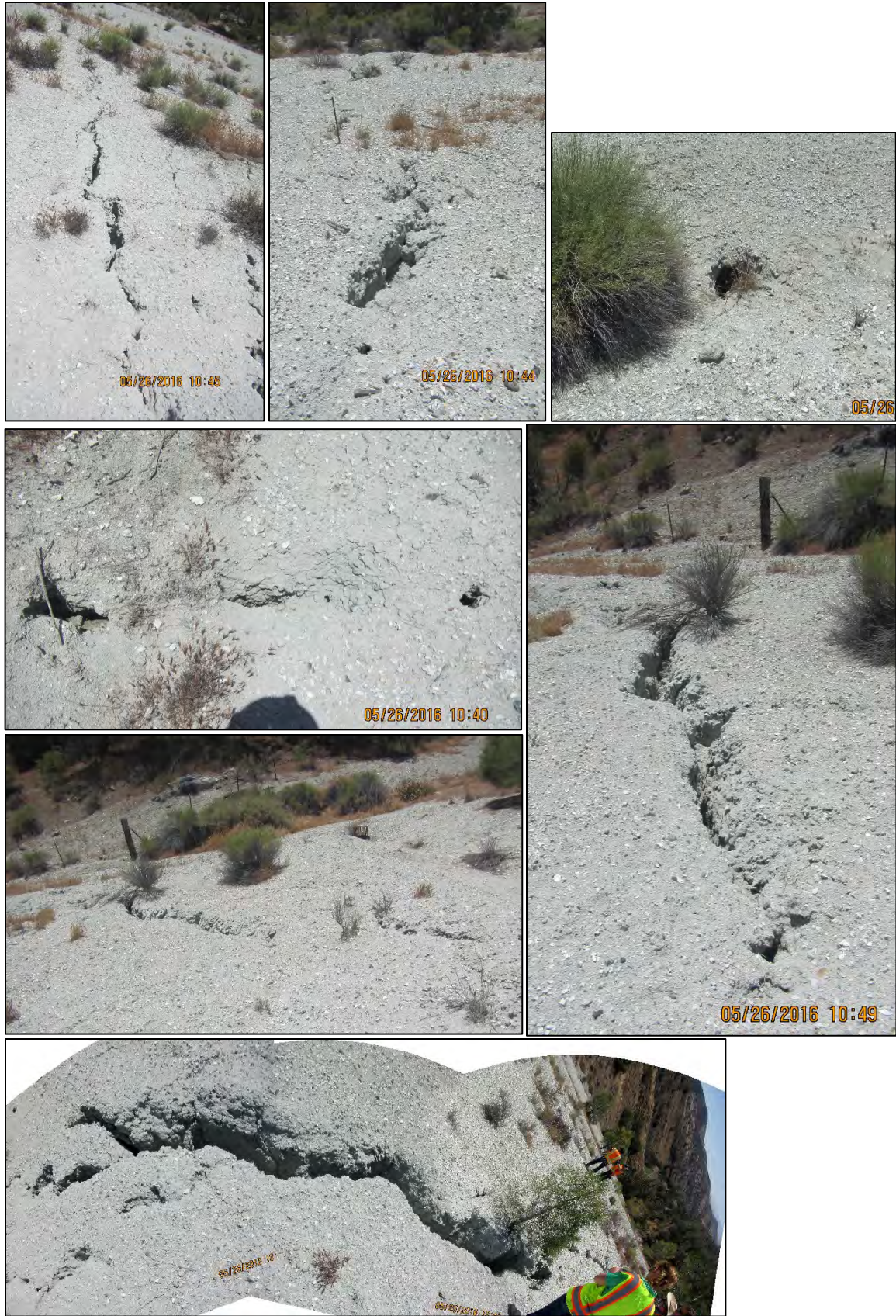
Photo 56. Cracks and Holes in the JMM Tailings Pile Slope
