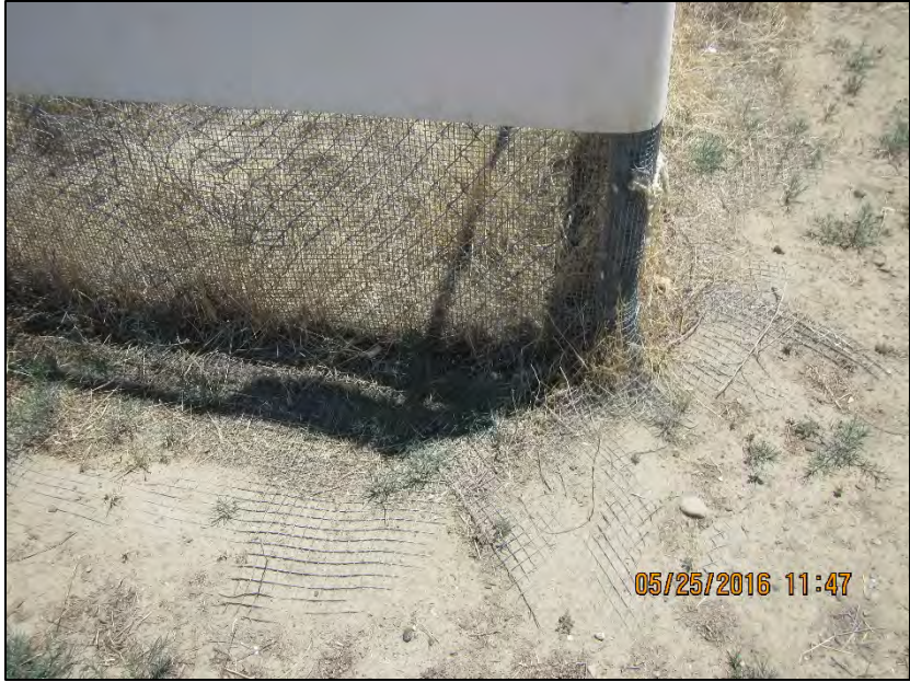
Photo 31. Newly Installed Chicken Wire Fencing to Exclude Rodents at City OU Landfill.
