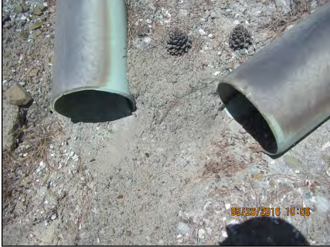
Photo 57. JMM Drainage System Outlet to Dissipation Pond
