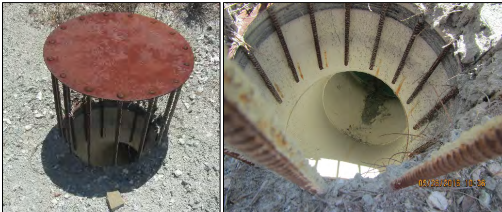
Photo 55. JMM Tailings Pile Drainage Collection Device
