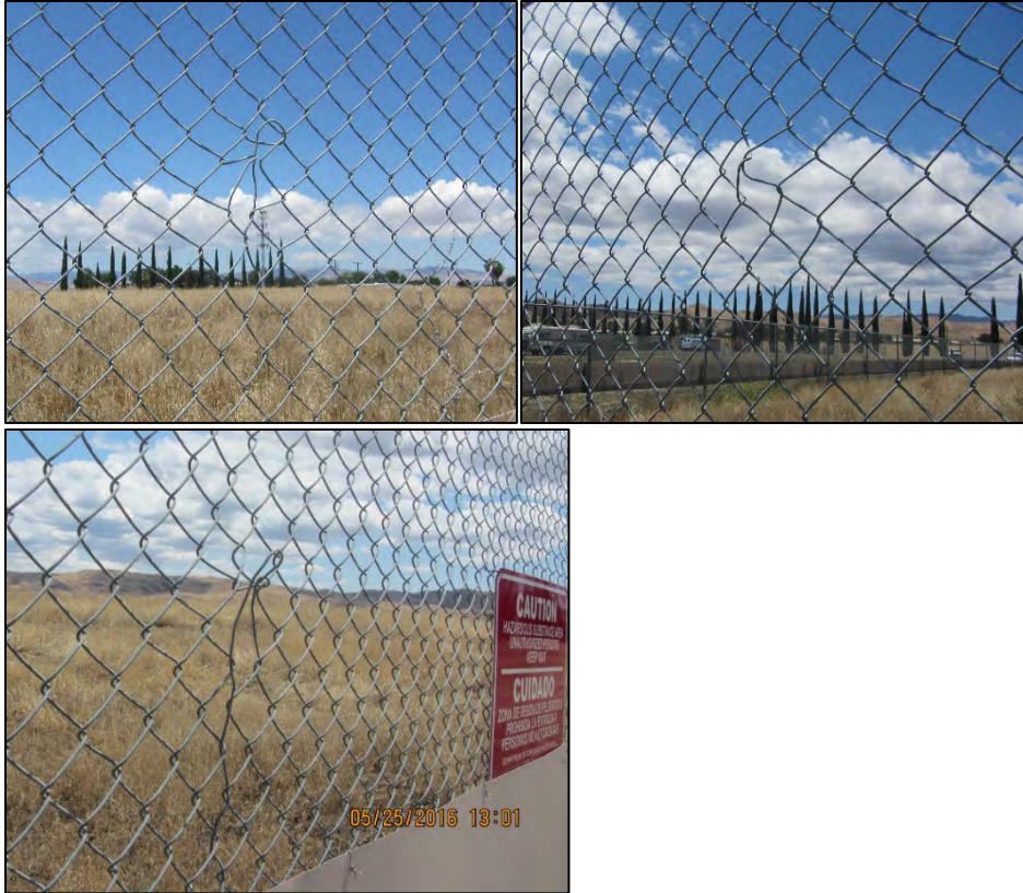
Photo 33. Minor Fencing Damage at City OU Landfill.
