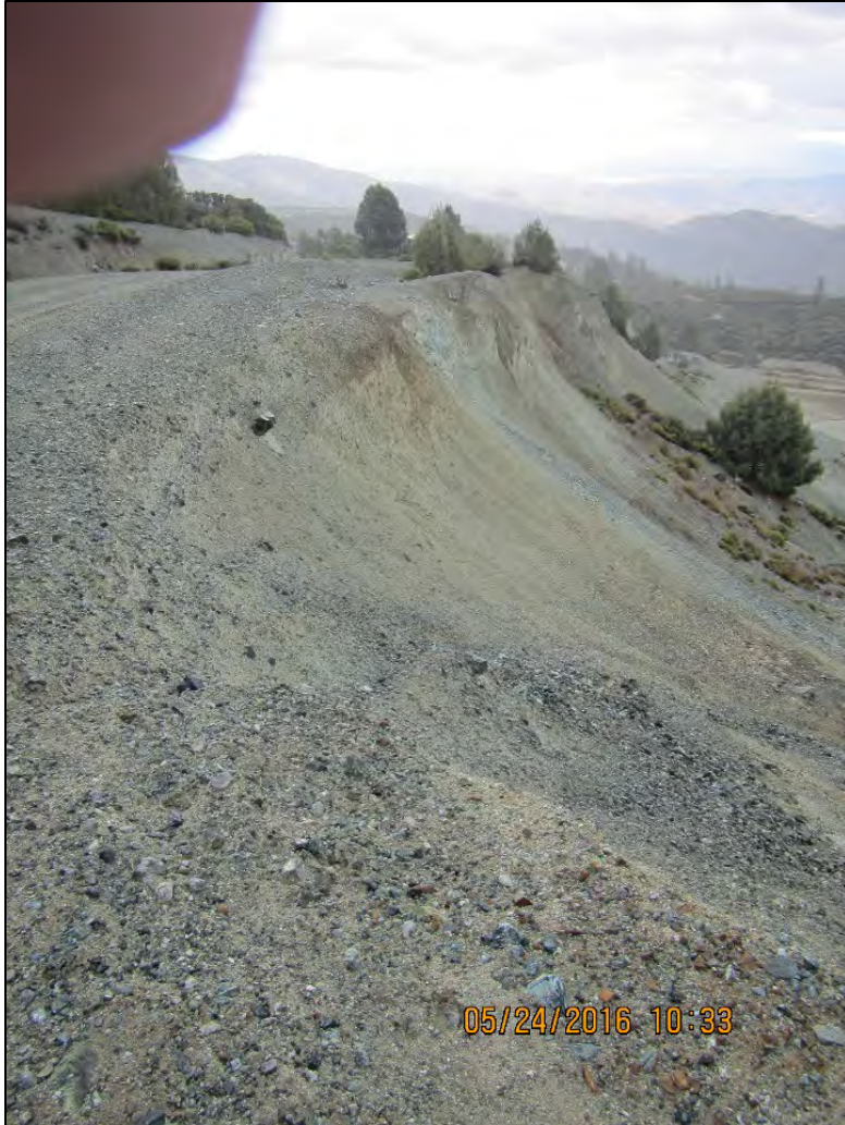
Photo 7. Past Erosion along Road to Atlas Pond A.
