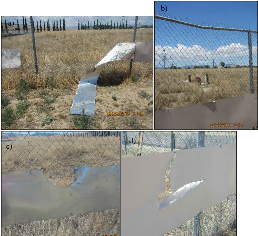
Photo 32. Damaged Sheet-metal Fencing at City OU Landfill; a) broken fencing, b) damaged fencing indicating potential attempted access, c) damaged fencing from intentional tearing, d) damaged fencing likely from accidental vehicle contact.
