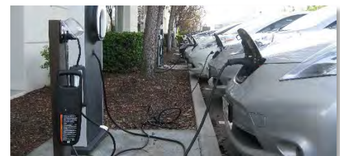
Figure 7. Electric vehicle charging stations in TiVo's parking lot.
