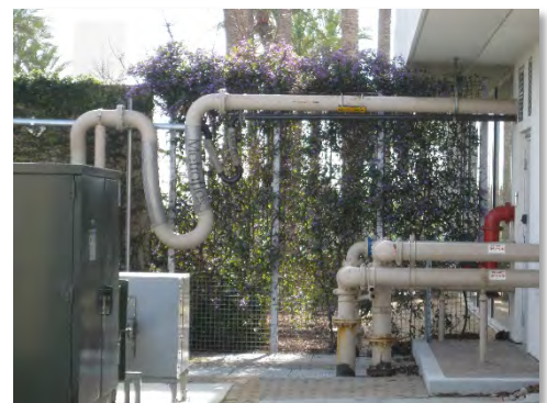
Figure 5. Flexible tubing at America Center helps to address landfill settlement at the site.
