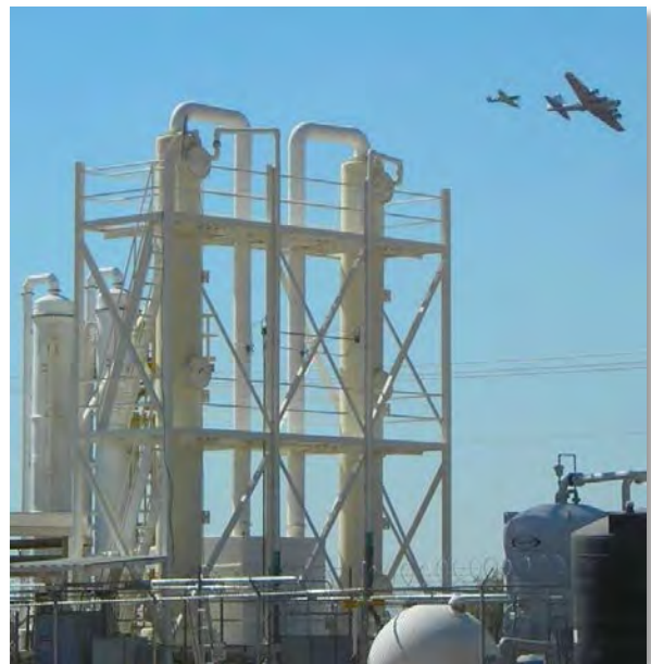
Figure 3. The main PGA-North groundwater treatment system.
