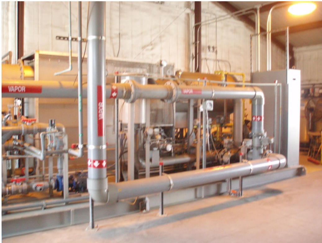
Photo 8: Flame Thermal Oxidizer view 2. May, 27 2010
