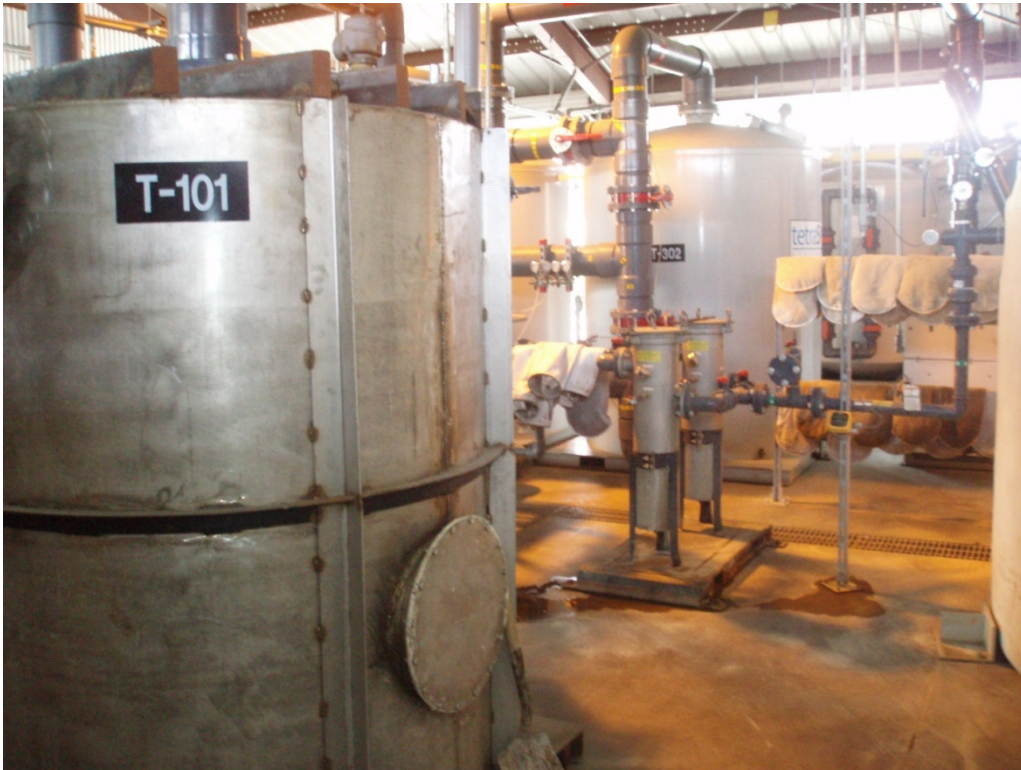
Photo 2: Knockout tank T-101 in foreground with Carbon tanks T-302 in background. May 27, 2010.
