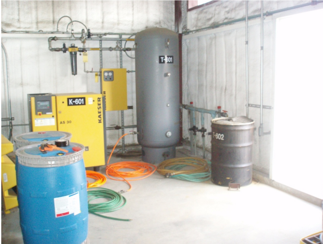
Photo 3: Compressed air tank. T-601. May 27, 2010
