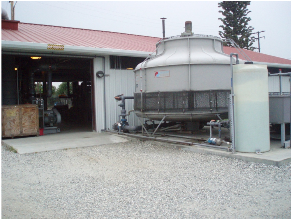
Photo 10: View of treatment plant facing southwest and vapor condenser. May 27, 2010.
