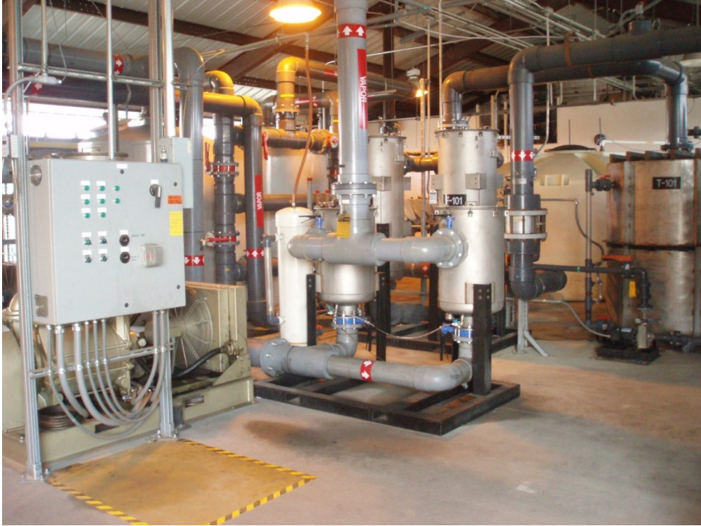
Photo 9: SP-104 and blower control panel. May 27, 2010
