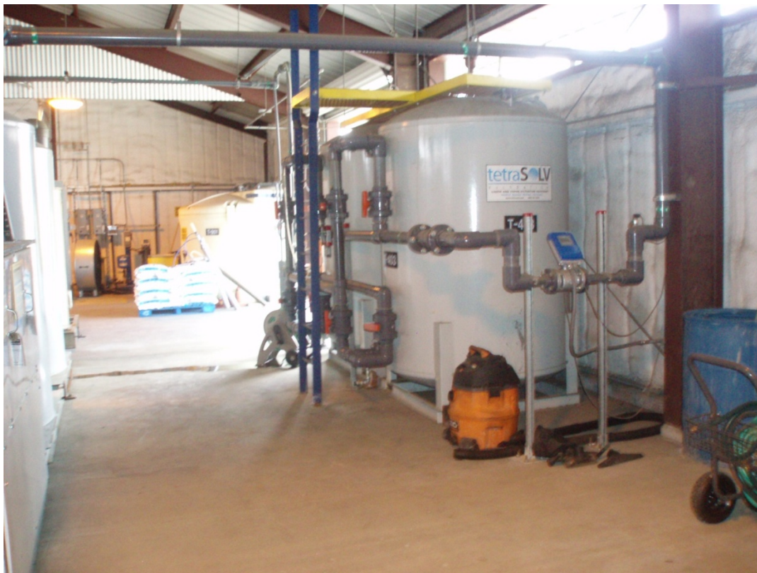
Photo 5: Liquid phase carbon adsorber tanks T-302, and SP-205 to SP-208. May 27, 2010.
