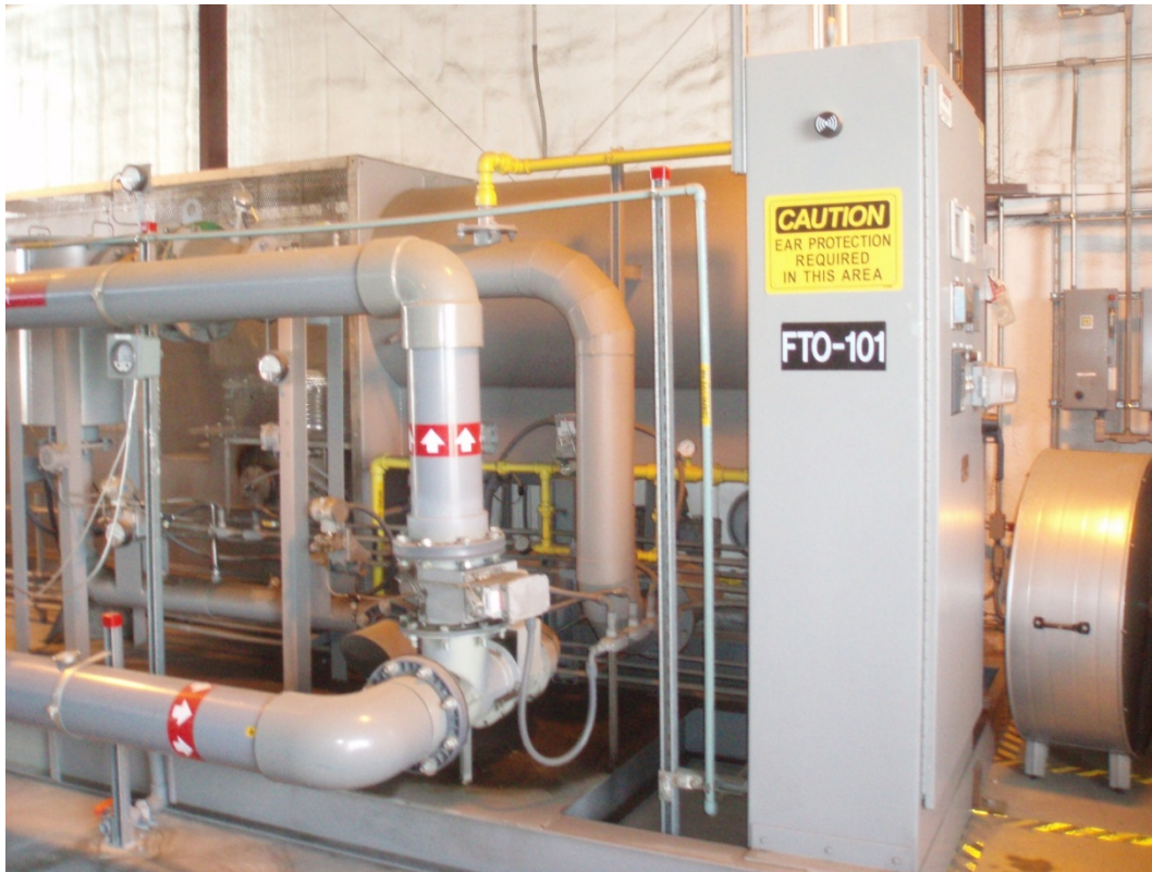
Photo 7: Flame Thermal Oxidizer at East end of plant. May 27, 2010.
