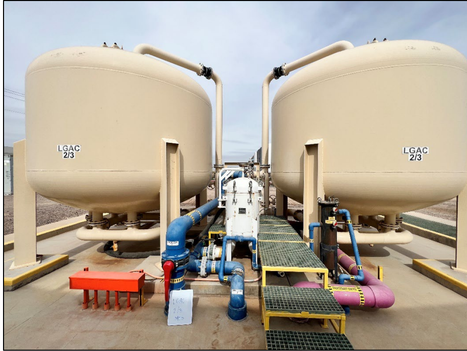
Photograph 11. February 13, 2025, 12:48 PM PGA North main treatment system LGAC vessels (LGAC 2/3). Facing north.
