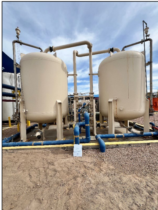
Photograph 10. February 13, 2025, 12:42 PM PGA North main treatment system ion exchange vessels. Facing east.
