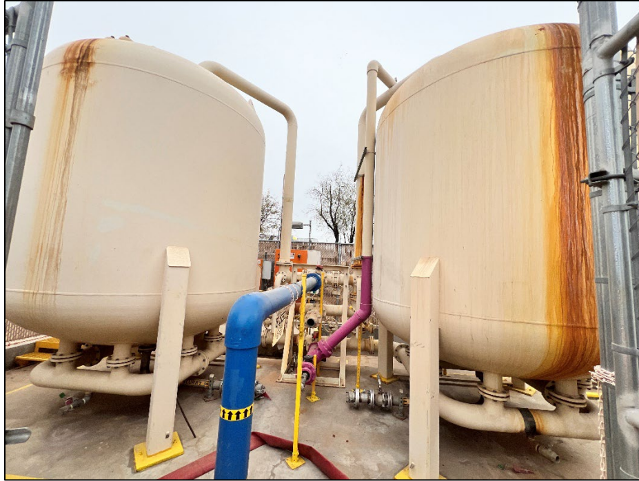
Photograph 17. February 13, 2025, 01:48 PM PGA North groundwater treatment system EA-05 LGAC vessels. Facing north.
