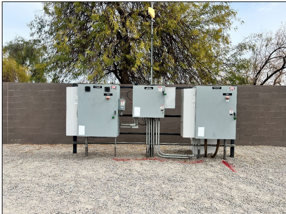
Photograph 14. February 13, 2025, 01:29 PM PGA North extraction well EA-14 control panels. Facing east.
