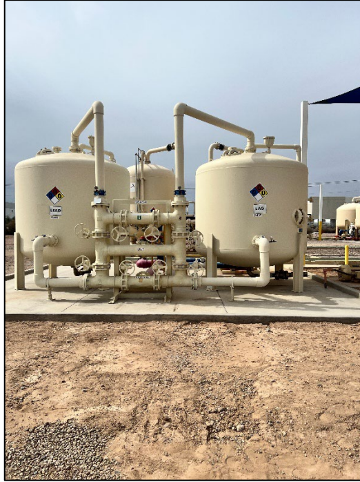
Photograph 13. February 13, 2025, 01:22 PM PGA North main treatment system LGAC vessels (LGAC 4). Facing east.
