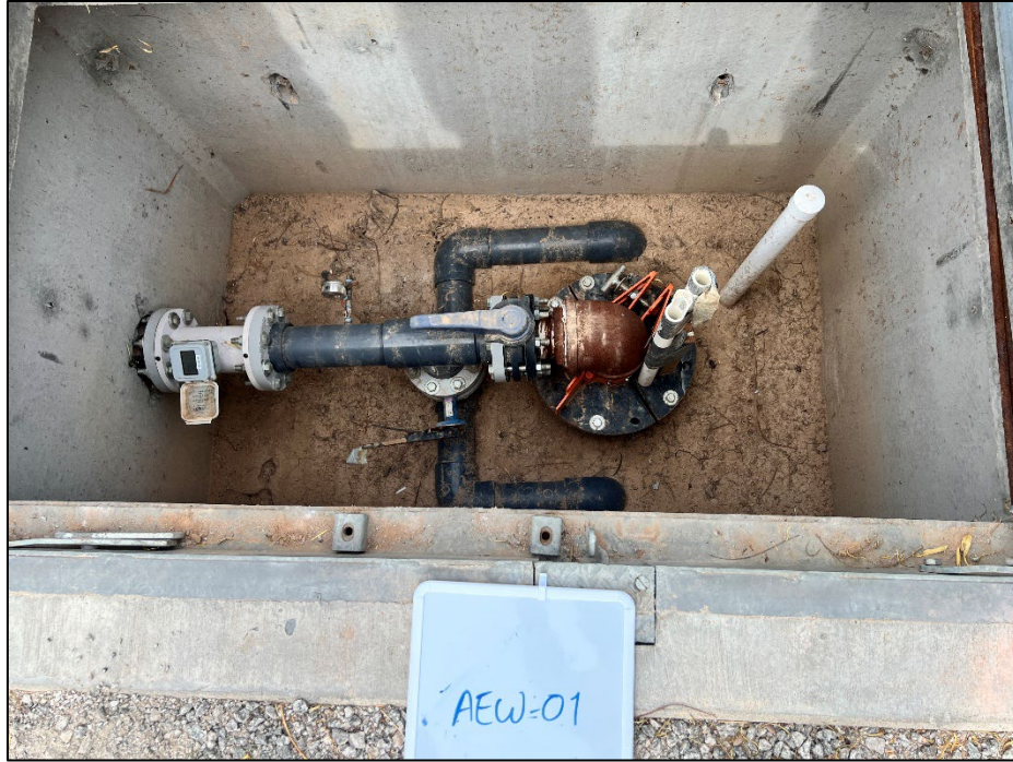
Photograph 15. February 13, 2025, 01:31 PM PGA North injection well AEW-01 (potential use for additive emplacement). Top view.
