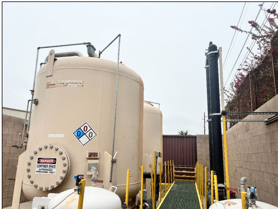
Photograph 20. February 13, 2025, 02:27 PGA North groundwater treatment system EA-08 LGAC vessels. Facing northeast.
