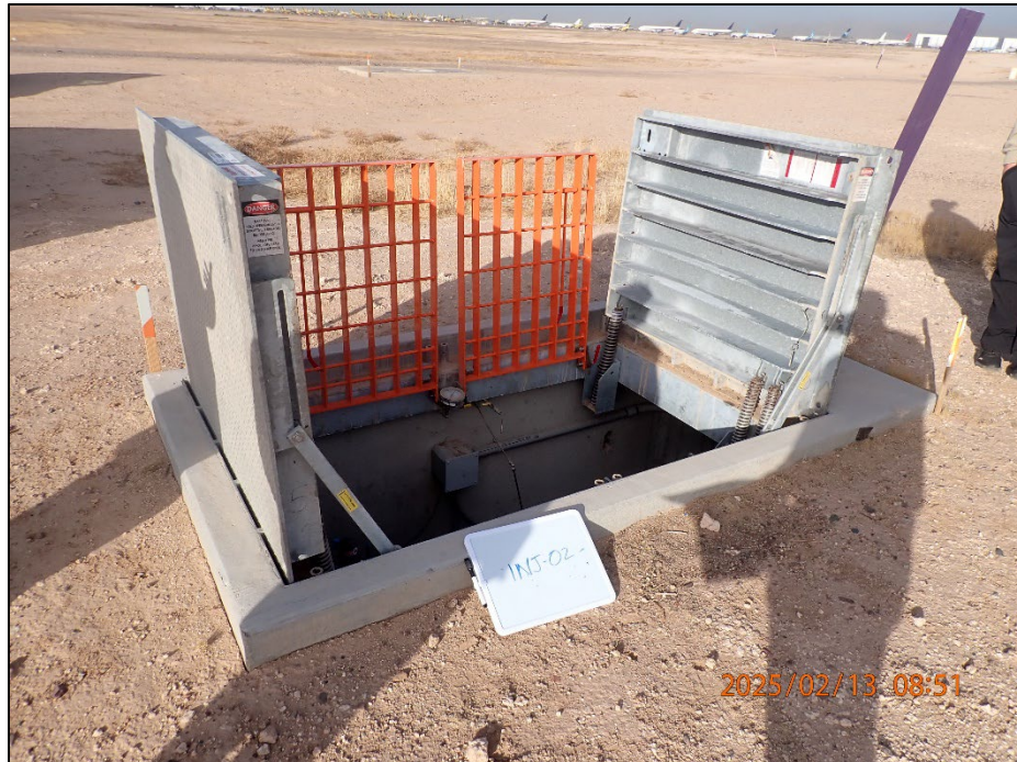
Photograph 2. February 13, 2025, 08:51 AM PGA South injection well INJ-02 vault. Facing northwest.
