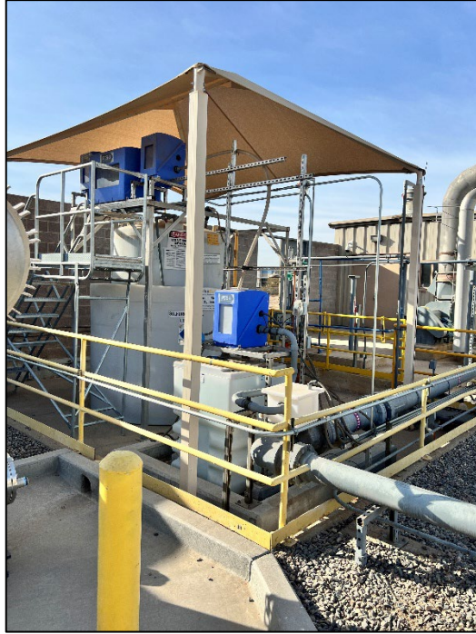
Photograph 3. February 13, 2025, 09:23 AM PGA South Subunit A acid storage tank within secondary containment. Facing south.
