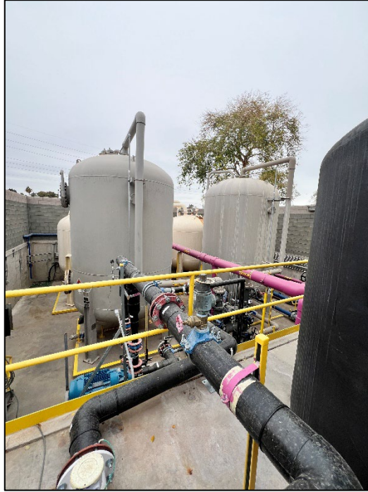
Photograph 19. February 13, 2025, 02:11 PM PGA North groundwater treatment system EA-06 LGAC vessels. Facing north.
