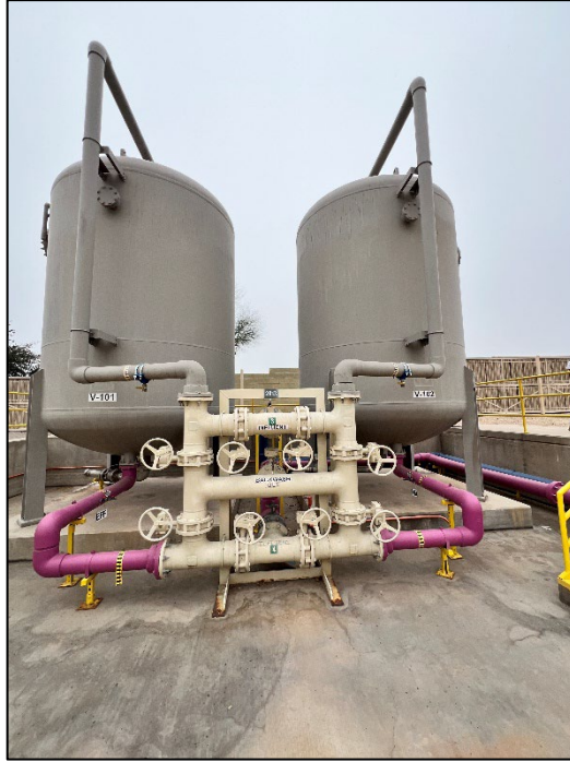
Photograph 21. February 13, 2025, 02:43 PGA North groundwater treatment system 33A LGAC vessels. Facing west.
