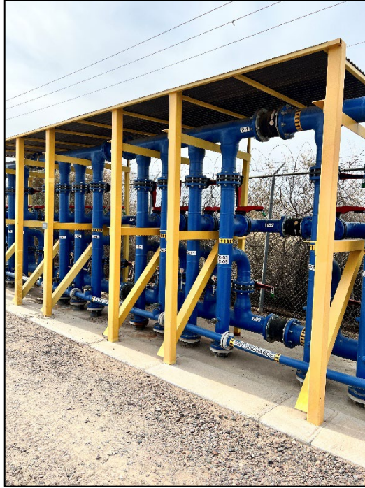
Photograph 9. February 13, 2025, 12:34 PM PGA North main treatment system process lines. Facing southwest.
