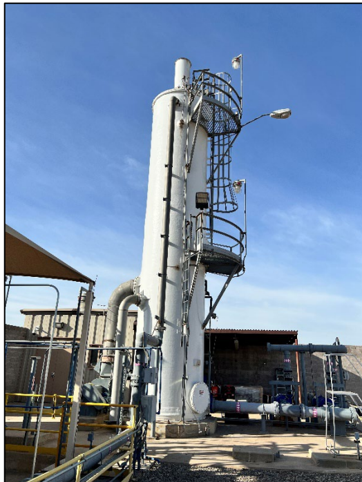
Photograph 4. February 13, 2025, 09:23 AM PGA South Subunit A air stripper. Facing southwest.
