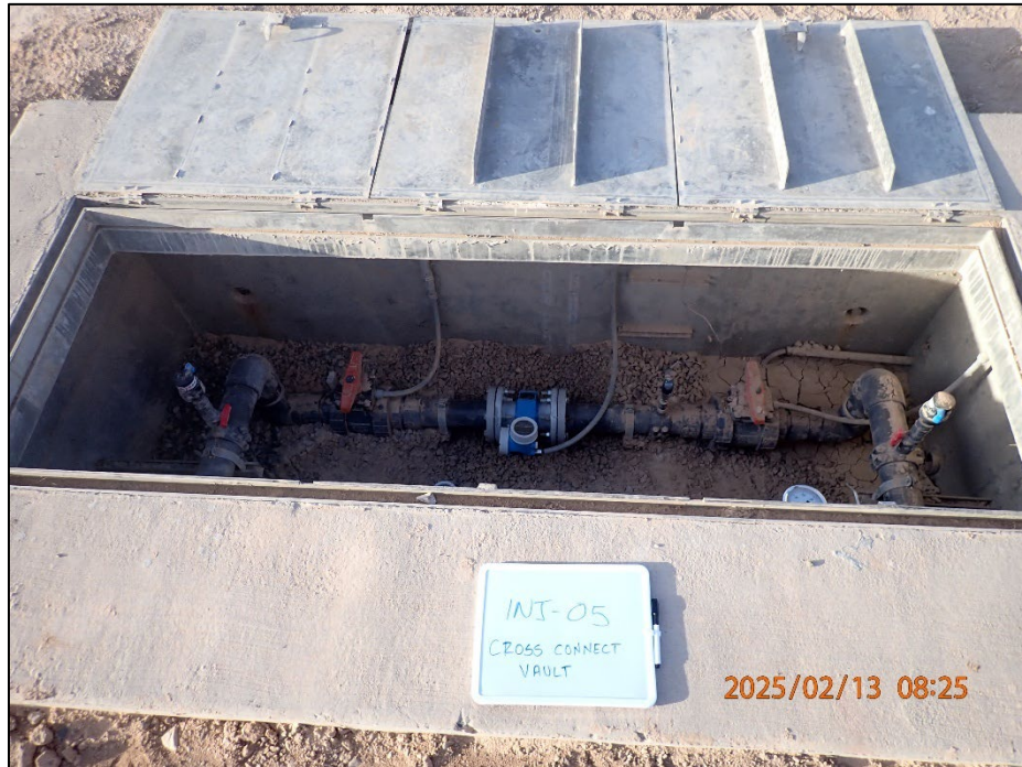
Photograph 1. February 13, 2025, 08:25 AM PGA South injection well INJ-05 cross connect vault. Facing west.
