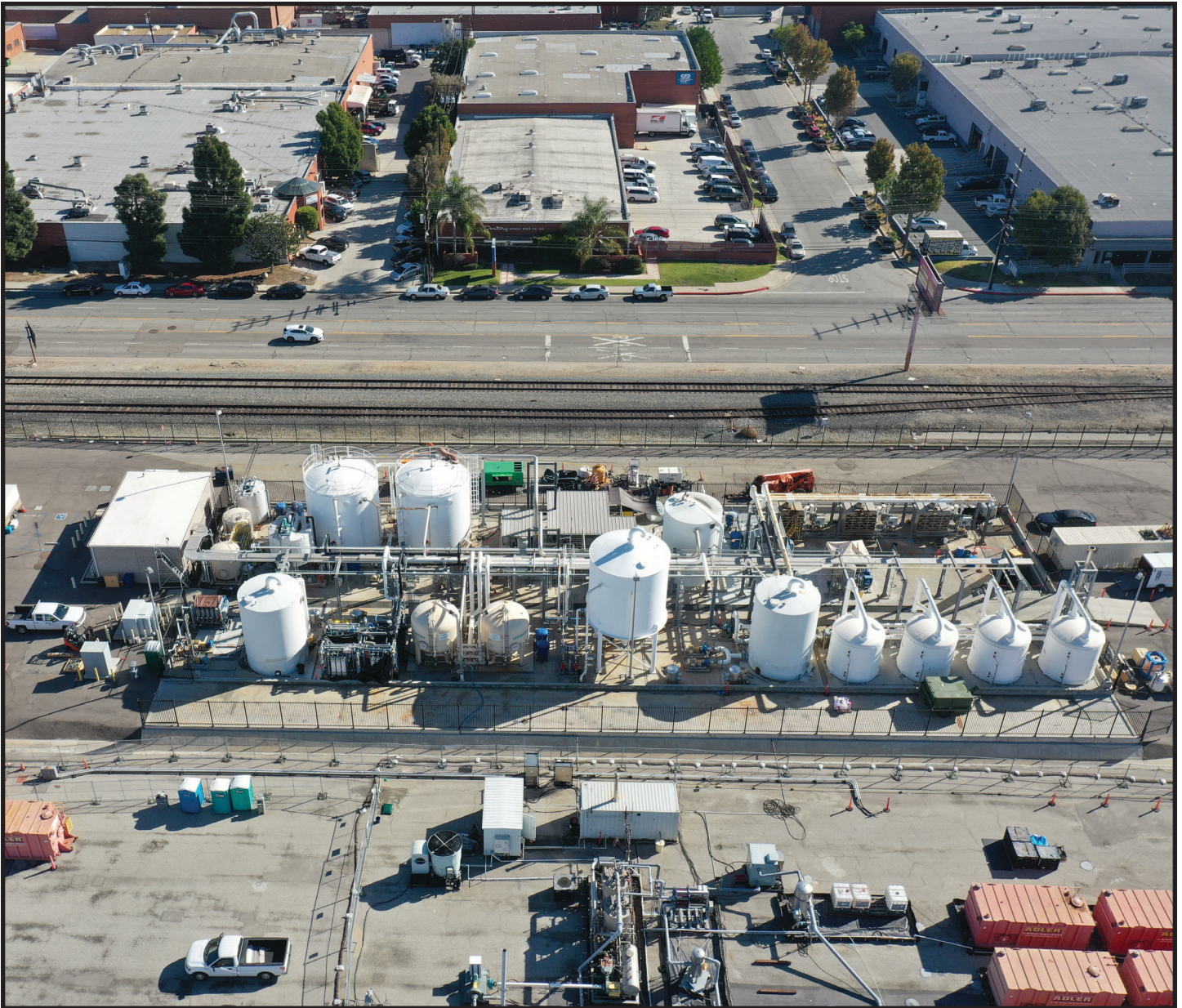
Aerial view of the pump and treat system at OU3G: Dual Site Groundwater.
