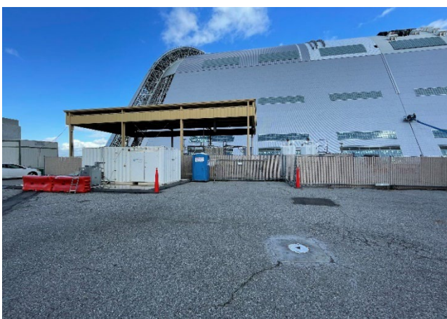
Site 28 West-side Aquifers Treatment System (WATS) – exterior (locked and secured). Temporary pre-treatment also pictured.
