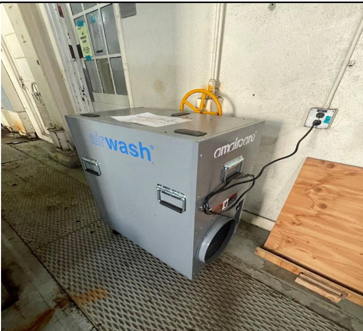
Air treatment unit in Moffett Building 10
