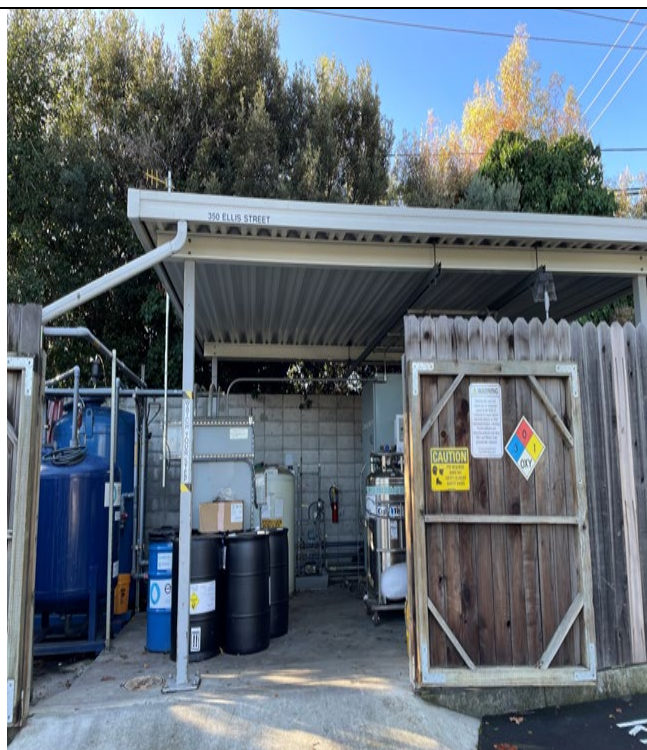
501 Ellis Street groundwater treatment system
