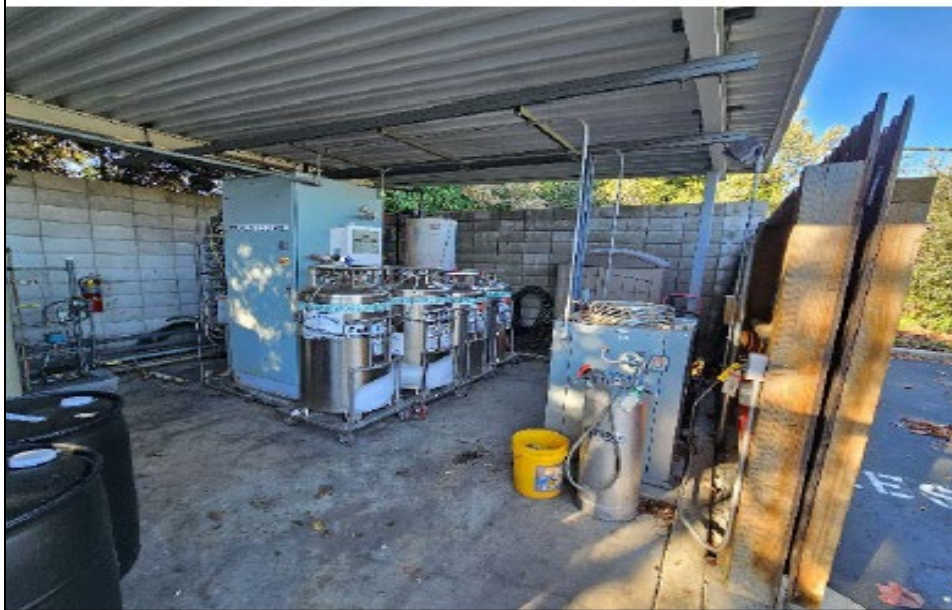
350 Ellis Street Groundwater Treatment System
