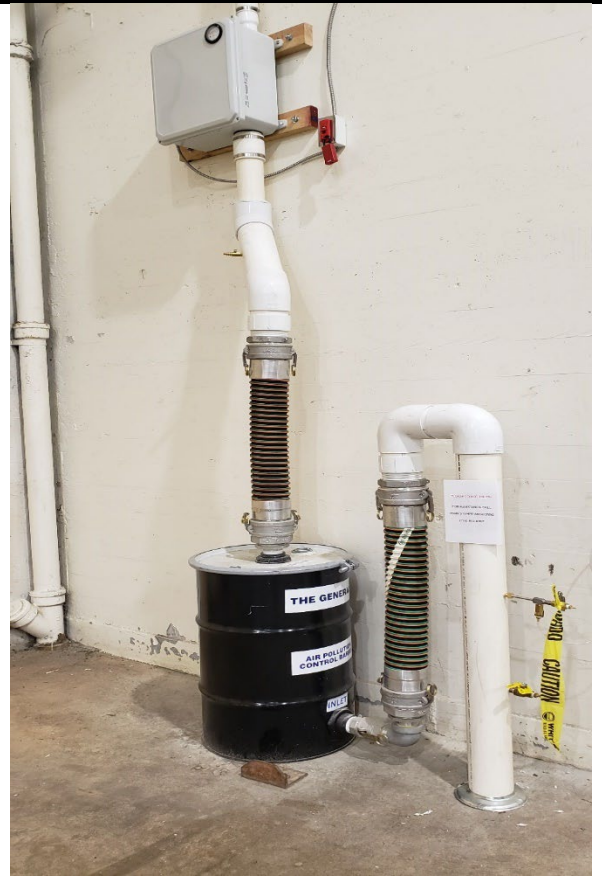
Vapor intrusion control system in Moffett Building 145
