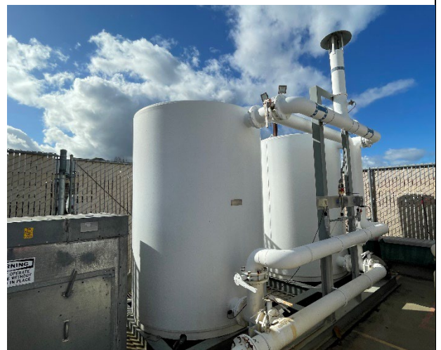
MEW Regional North of 101 Treatment System
