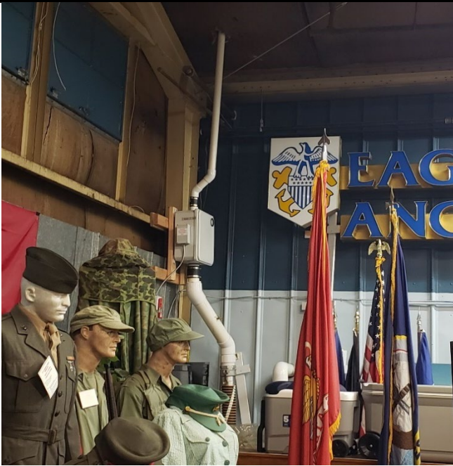
Vapor intrusion control system in Moffett Building 126
