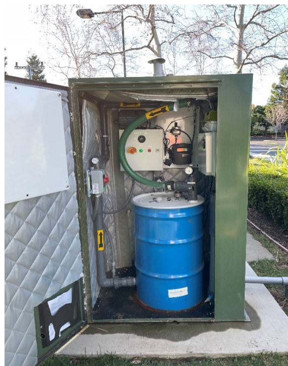
Vapor Intrusion treatment system – 350 Ellis St
