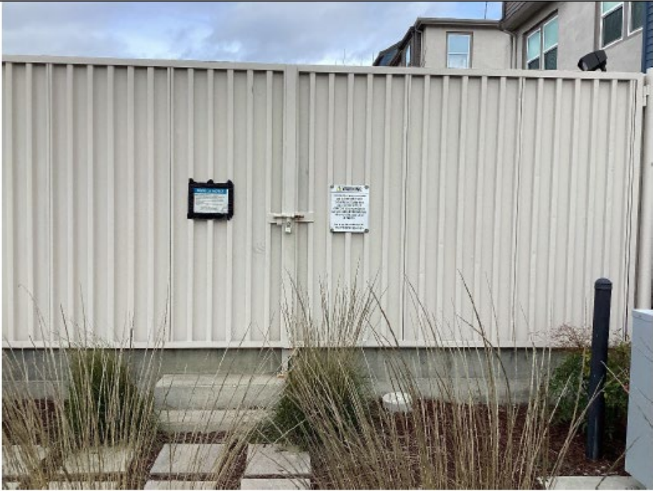
Gate for the AMD 915 LGAC treatment plant.
