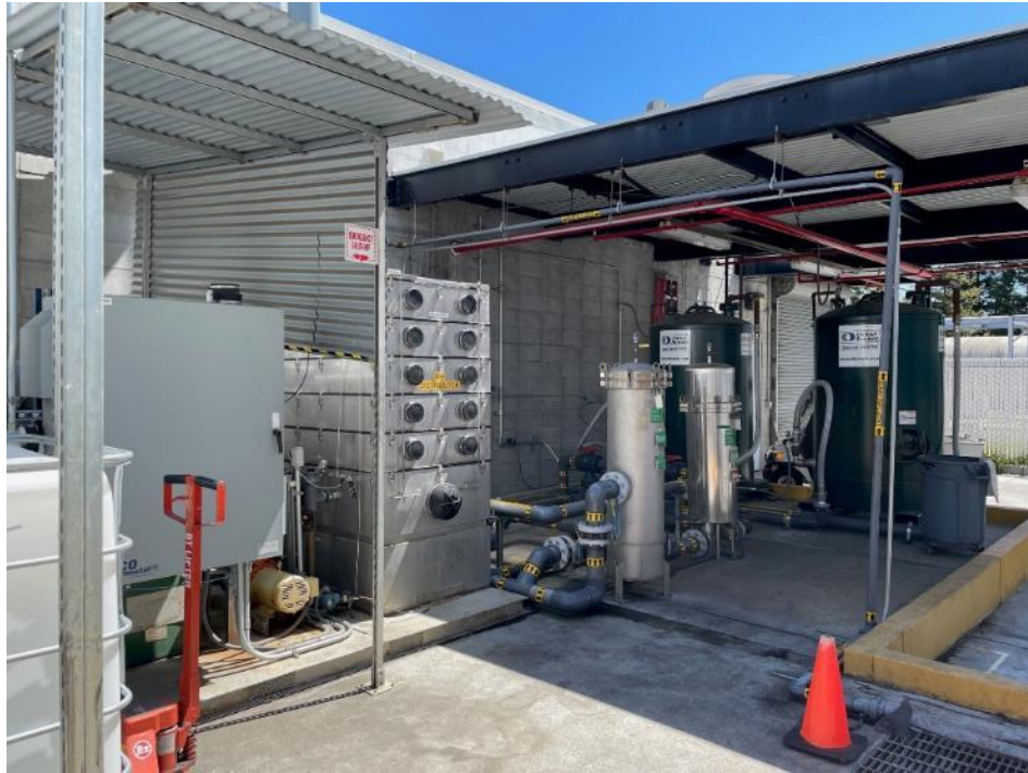
OU1 Subunit 1: control panel, air stripper, two cartridge filters, and GAC units.
