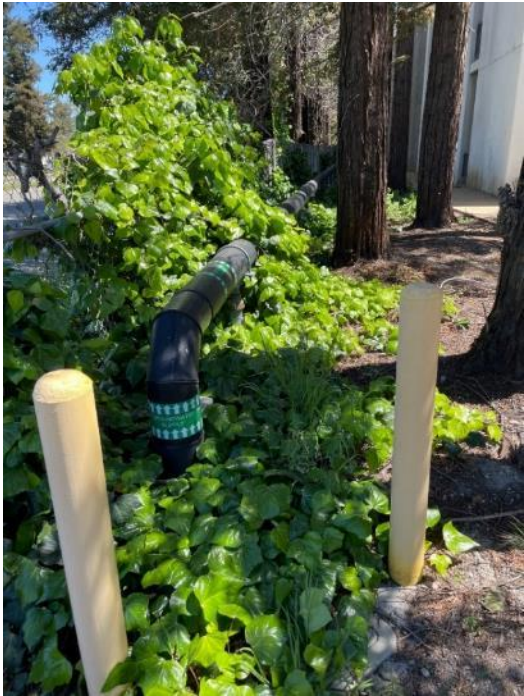
Water supply to the OU1 Subunit 1 GWETS. Photo taken approximately 100 feet North of the NW corner of Building E, facing east.
