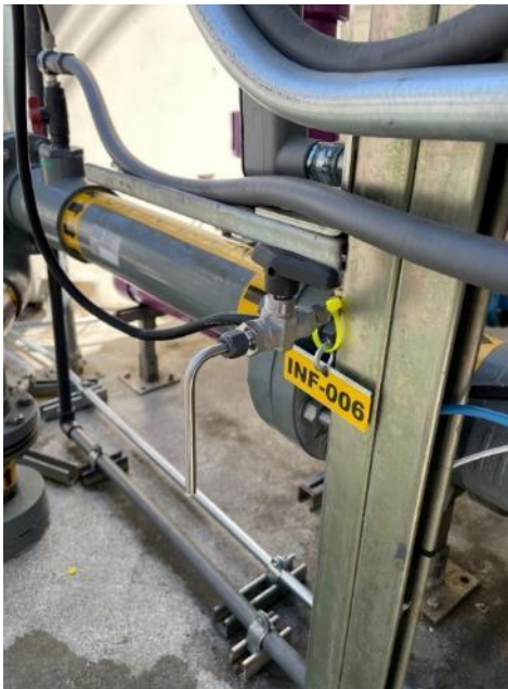
Influent sampling tap (INF-006), taps into influent line post antiscalant injection.
