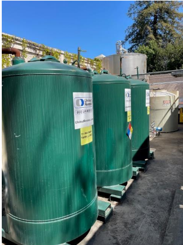
Lakeside GWETS. Temporarily shutdown as NFA has been submitted.
