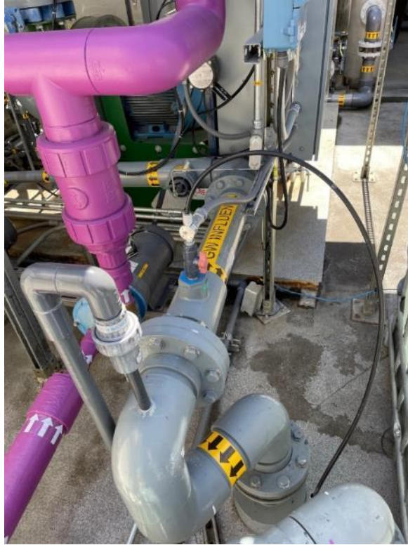
Influent line (grey), antiscalant injection point, and influent sampling tap (stainless steel in back).
