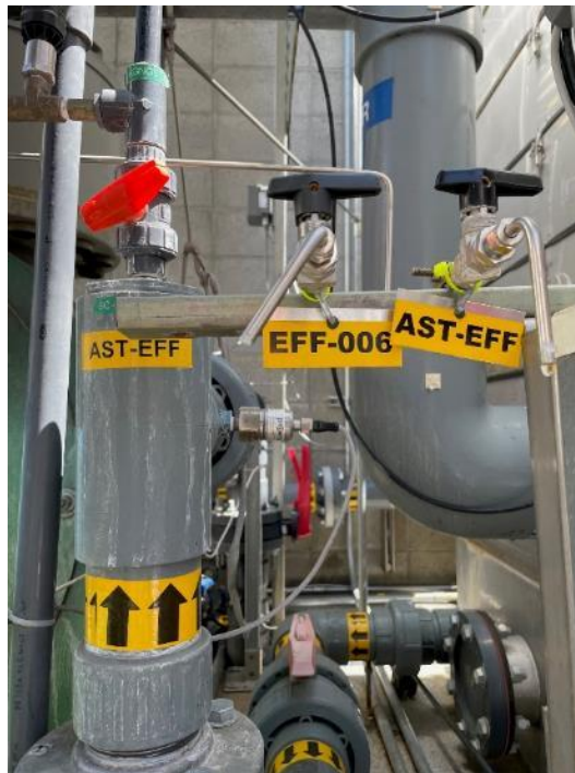
Air stripper effluent (AST-EFF) and Effluent (EFF-006) sample taps were tapped in the appropriate locations.
