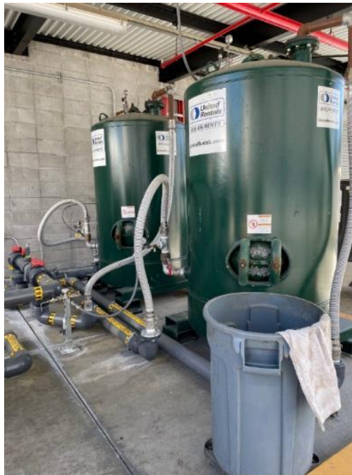
GAC vessels in series. According to signs on the rear of the vessels, the left vessel was the lag and the right was the lead at the time of the inspection.
