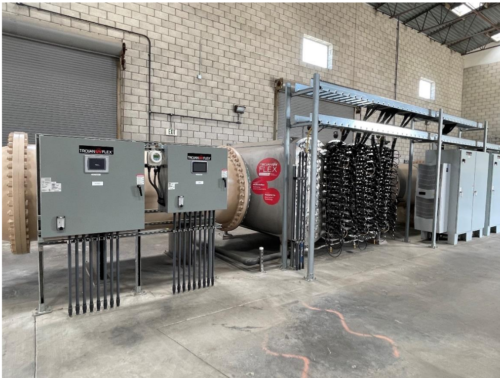
Figure 29 – Newly installed UV flex system (not in operation)
