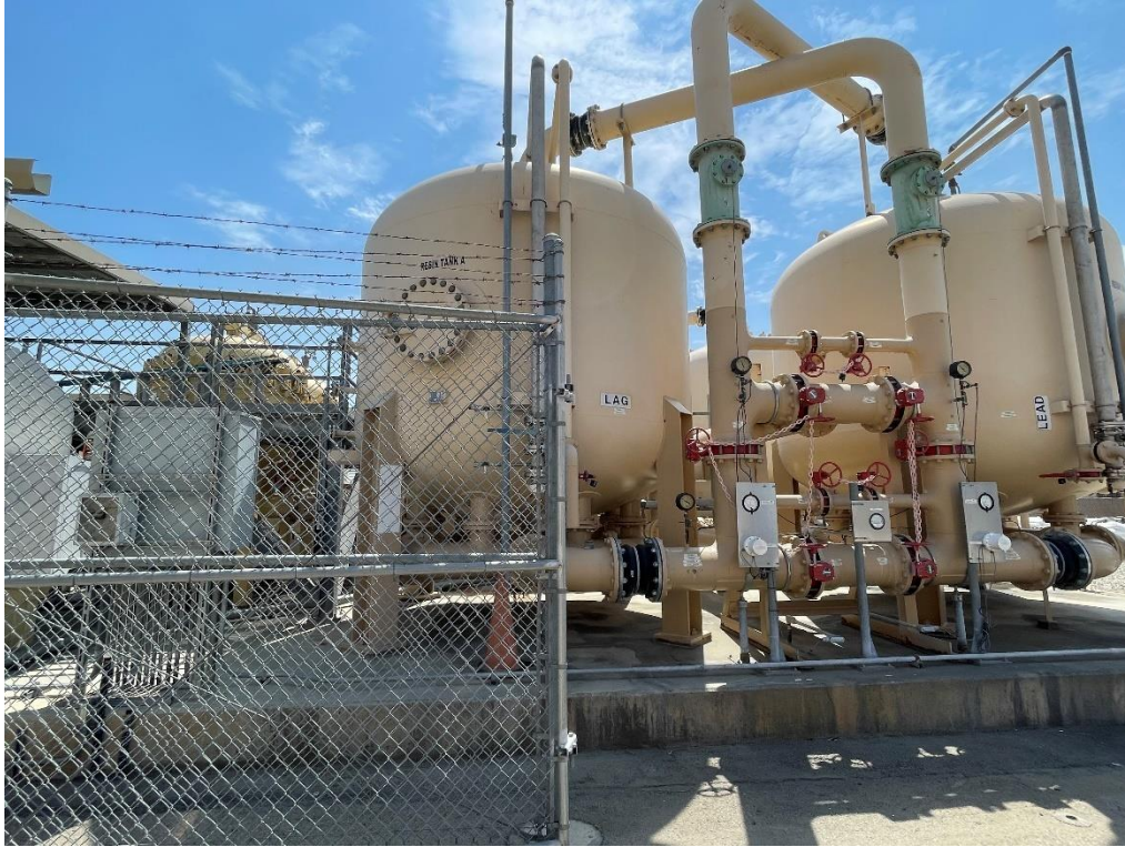
Figure 34 – Single pass IX resin vessels in lead and lag configuration
