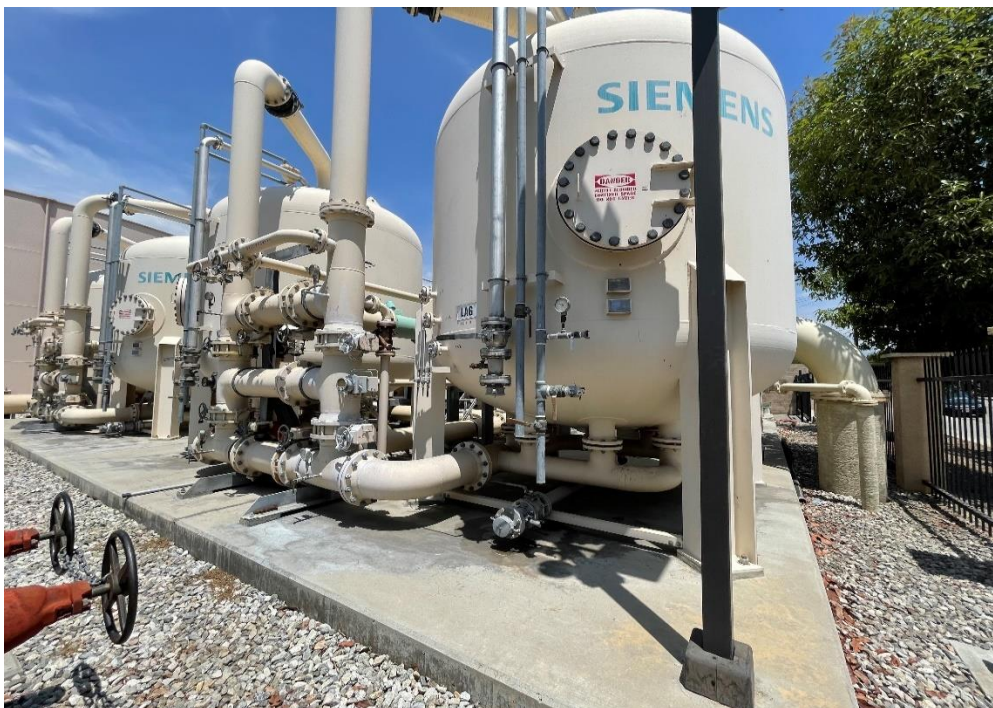
Figure 27 – 6 pairs of vessels in lead and lag configuration for IX treatment
