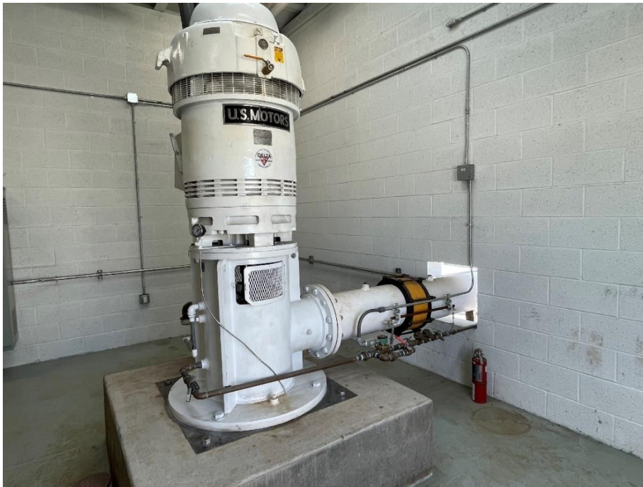
Figure 44 – Inside the housing unit for Well 1-4
