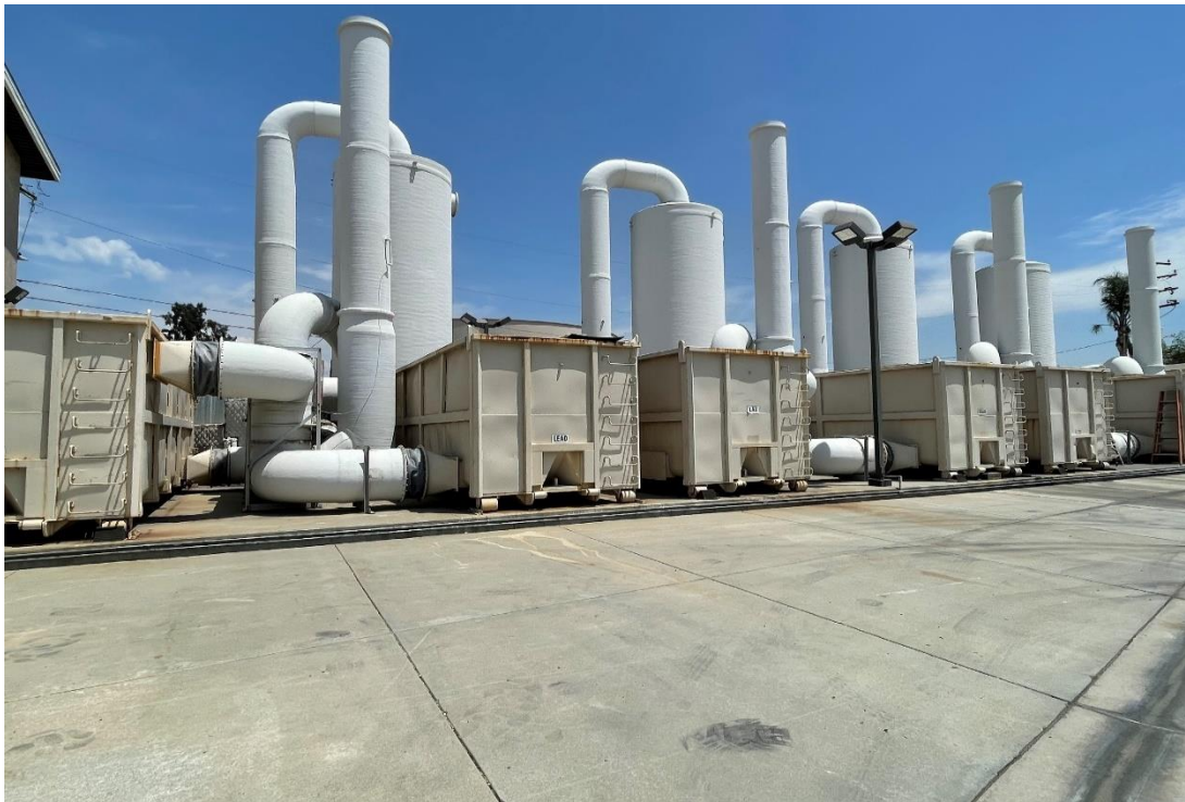
Figure 25 – Facing northwest, rear view of the four air stripping towers and associated carbon units
