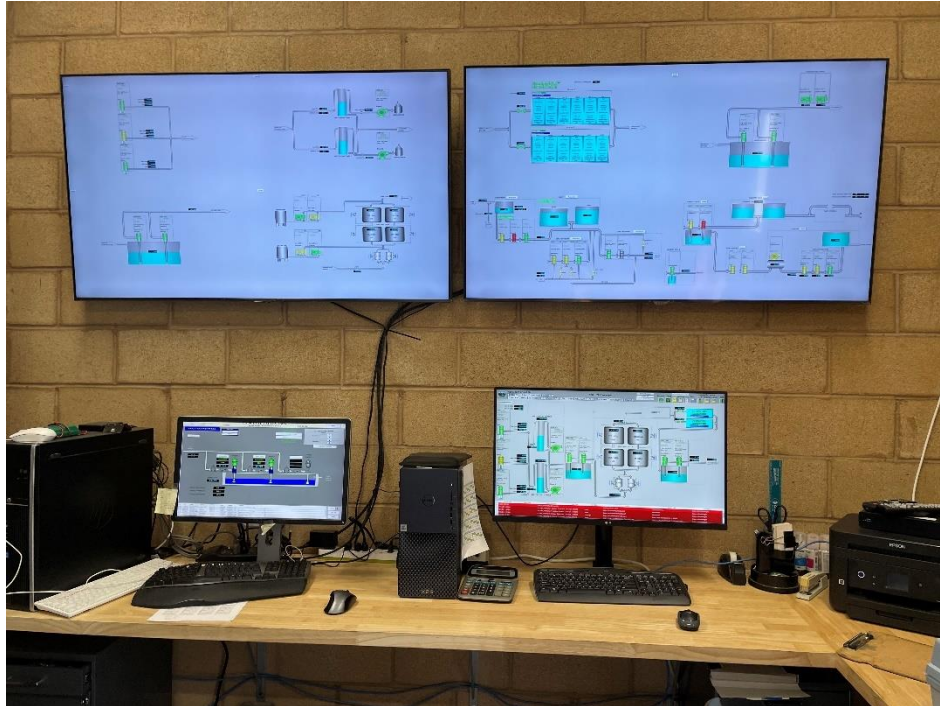
Figure 30 – SCADA system in the control room
