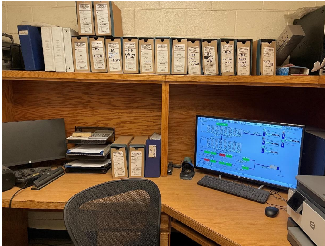
Figure 16 – Control room and SCADA controls with maintenance logs and O&M manuals
