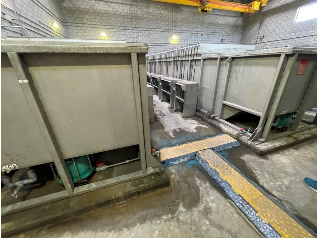
Figure 46 – Observation of leaking material associated with the UV treatment
