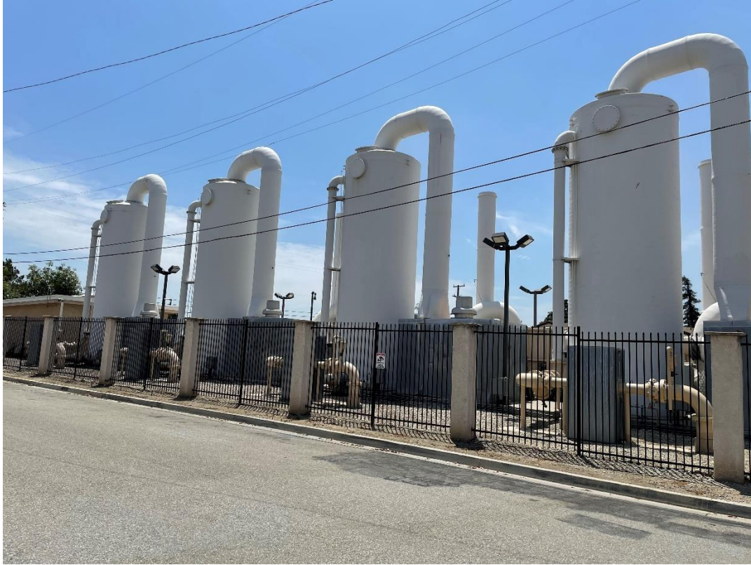
Figure 26 - Facing south, street view of air stripping towers
