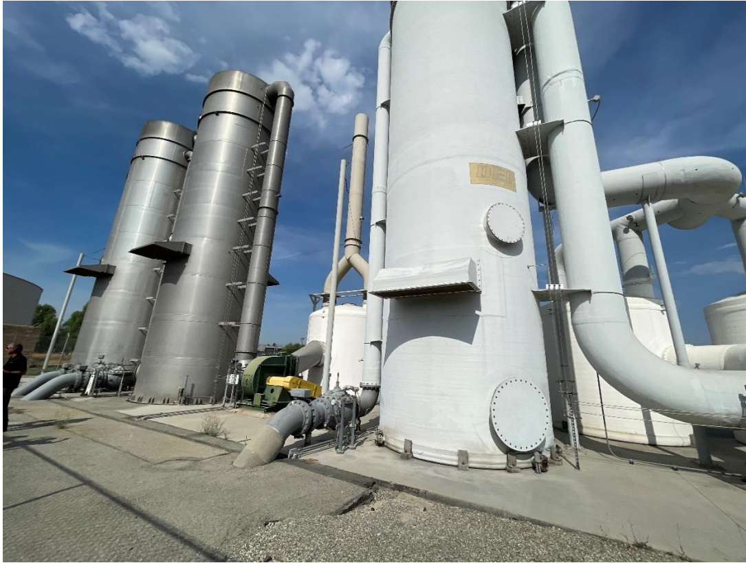
Figure 10 – Facing northwest within the secondary fence, three air stripping towers with carbon vessels alongside
