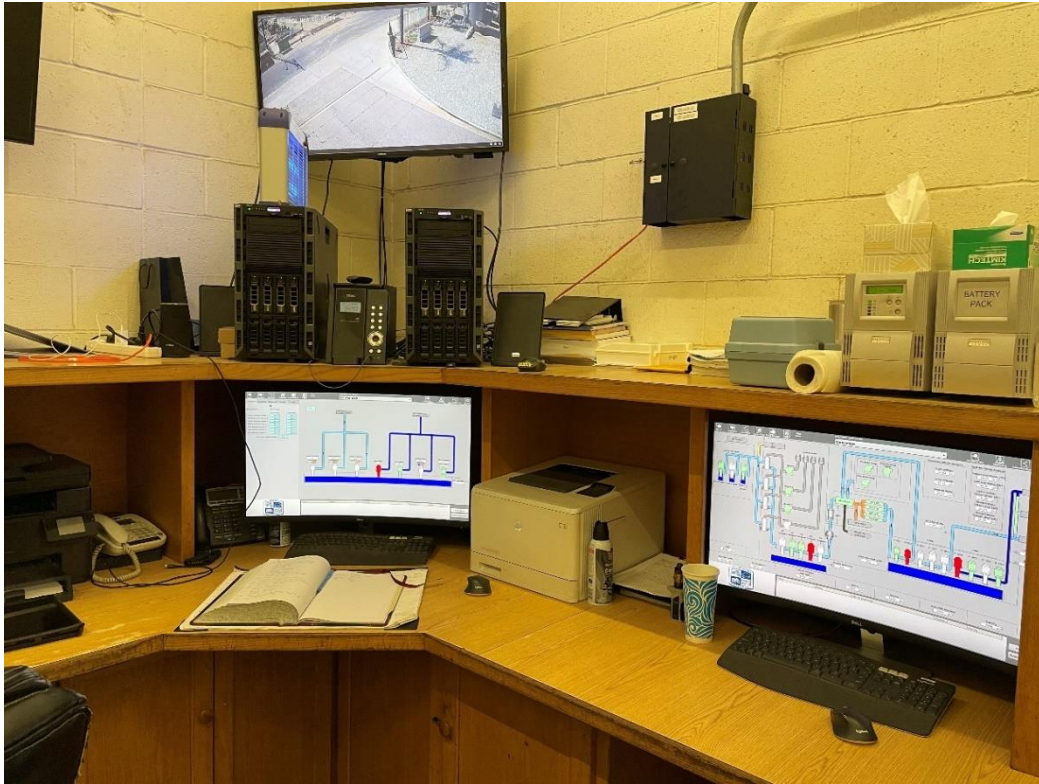
Figure 40 – SCADA system in control room
