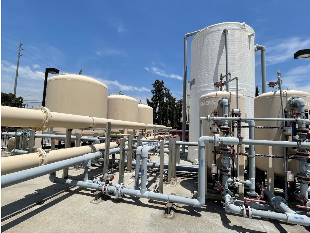
Figure 28 – Split Stream to 3 IX regenerative resin vessels in parallel
