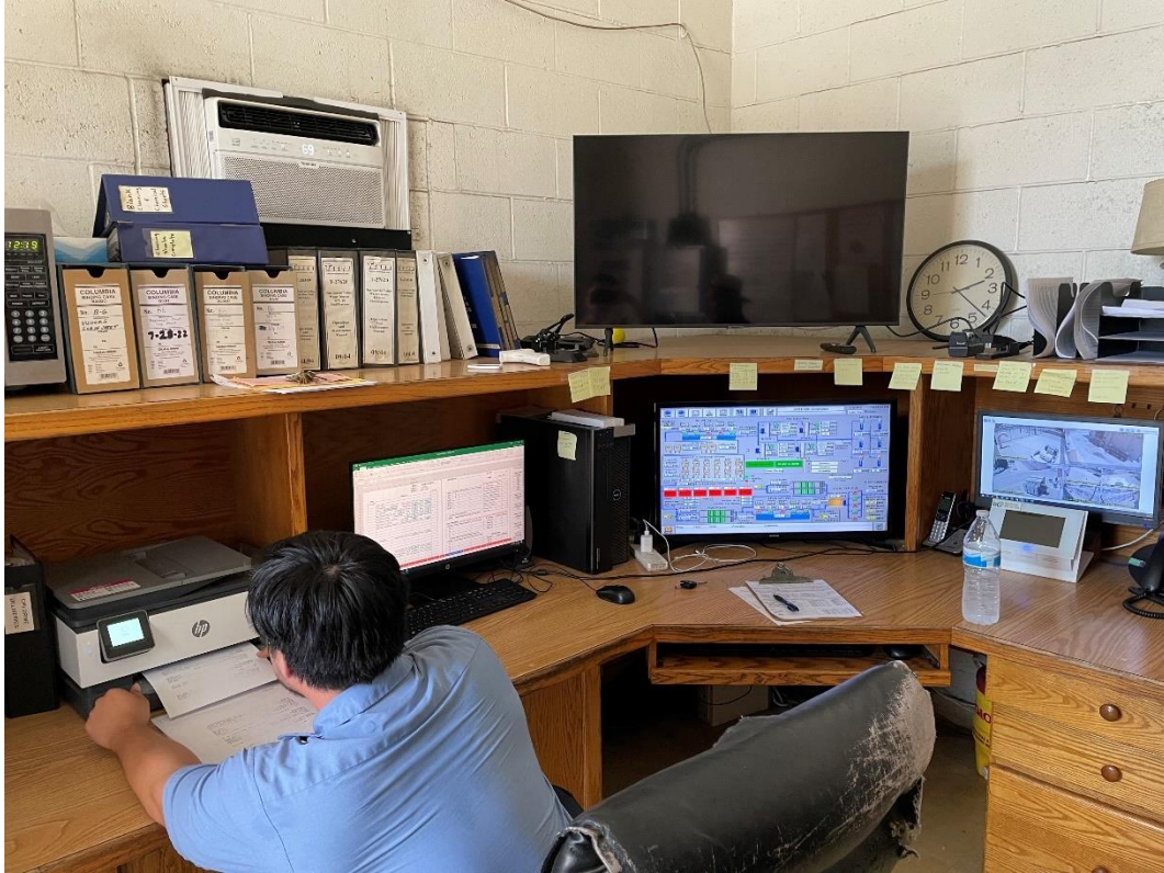
Figure 24 – Operator control room for LP
