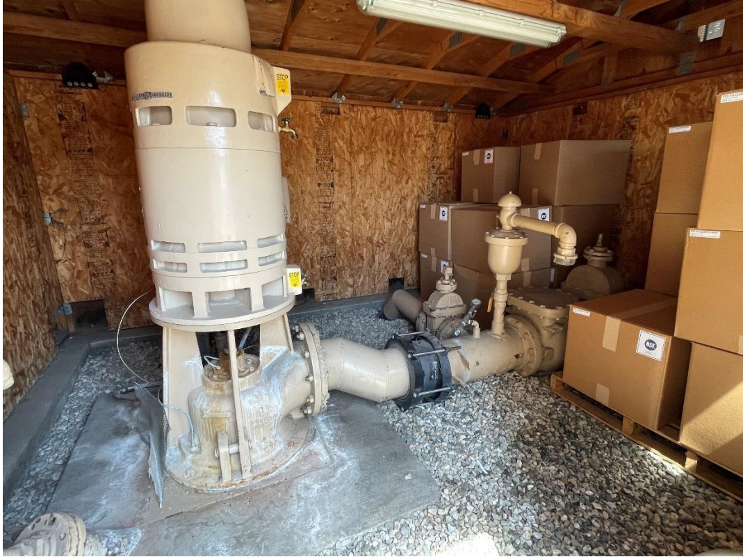
Figure 32 – Well 3, not in operation and on stand-by
