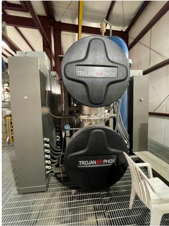
Figure 14 – Trojan UV PHOX treatment system (post IX)
