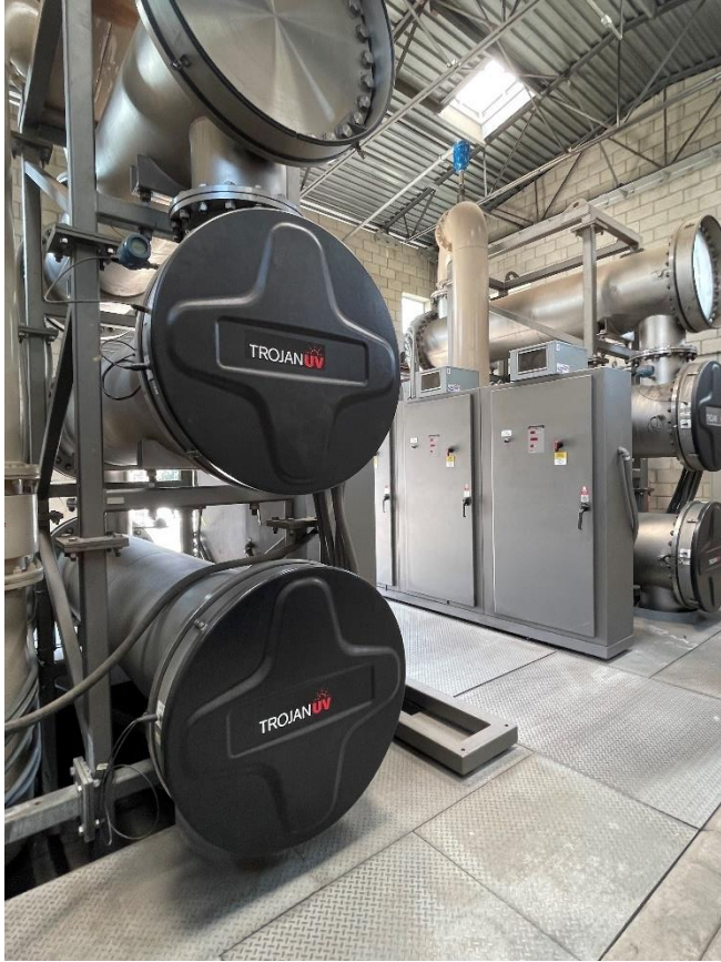
Figure 22 – Trojan UV treatment system for 1,4 dioxane
