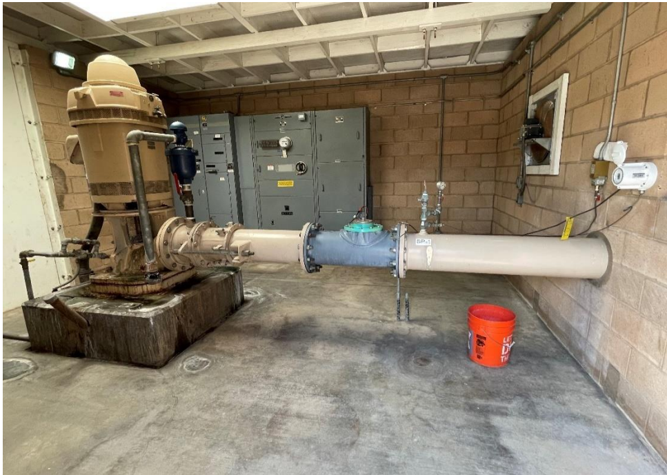
Figure 39 – Inside the housing unit of Well #2
