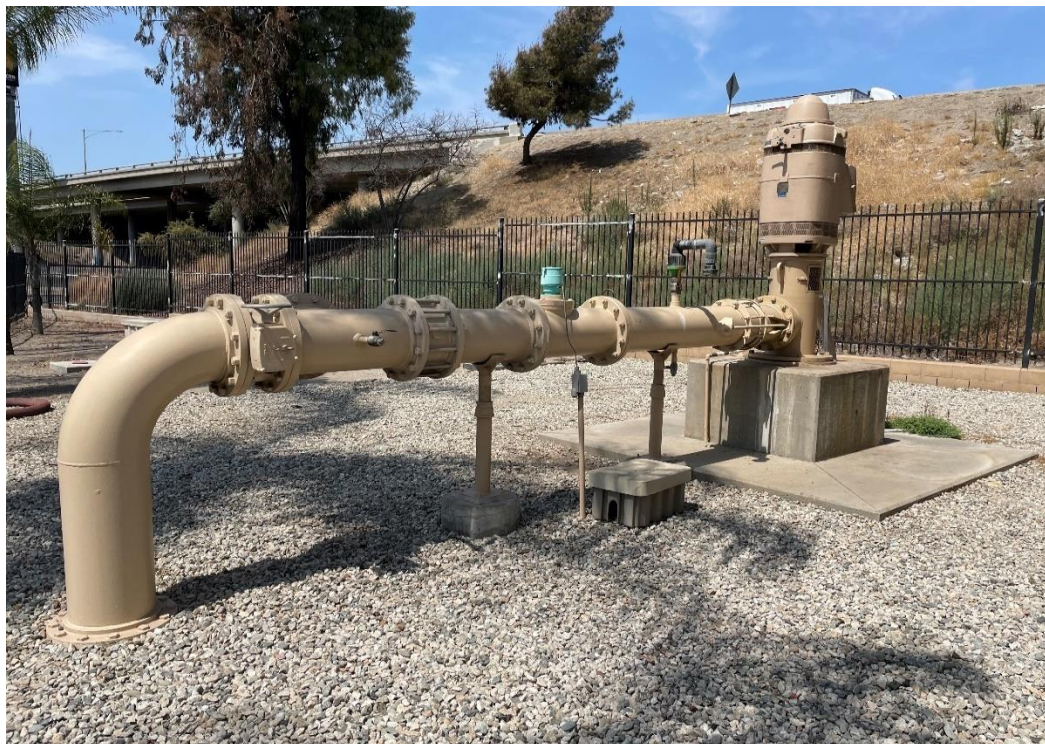
Figure 18 – B5E well on-site south of the control room building
