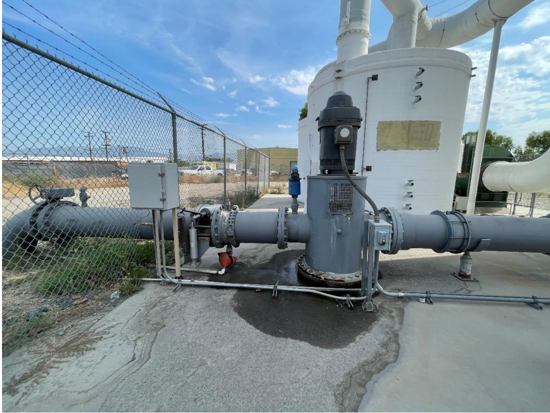
Figure 11 – Facing north, effluent piping from Air Stripper #3 and two carbon vessels in the back
