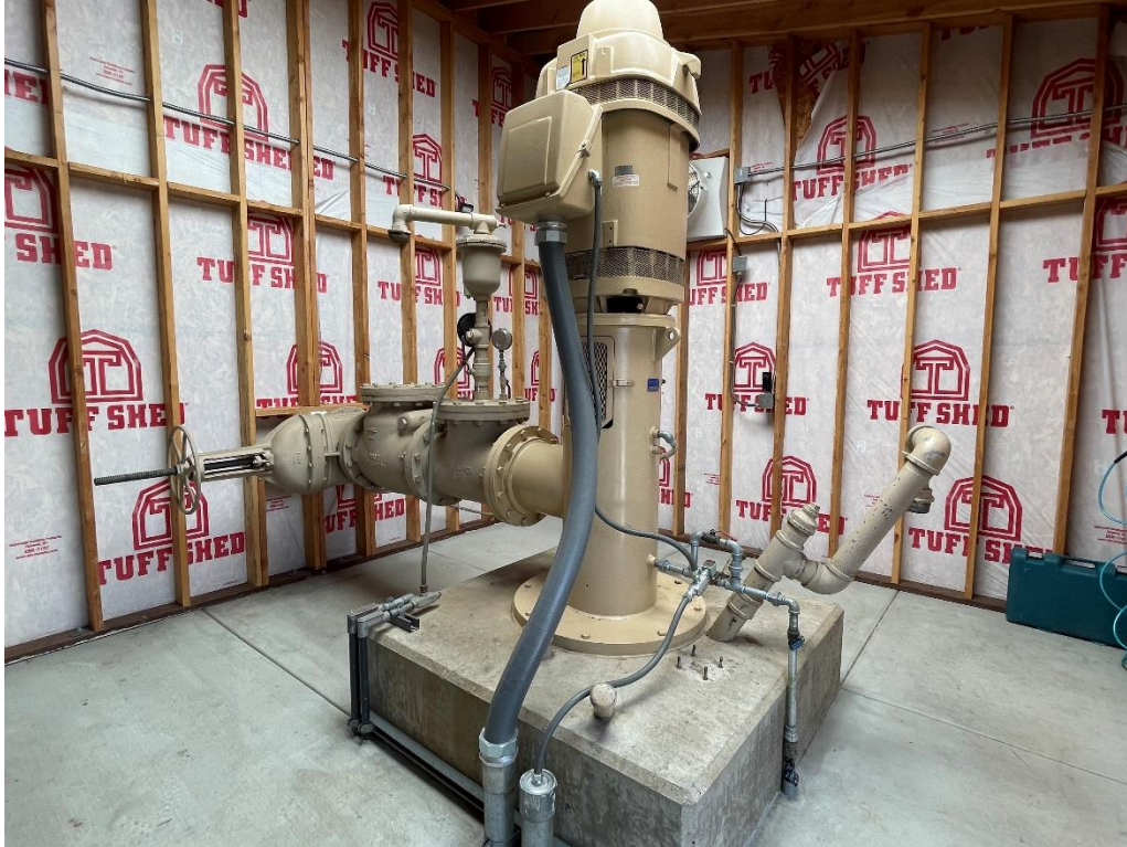
Figure 36 – Well #5, formerly submersible and now above ground
