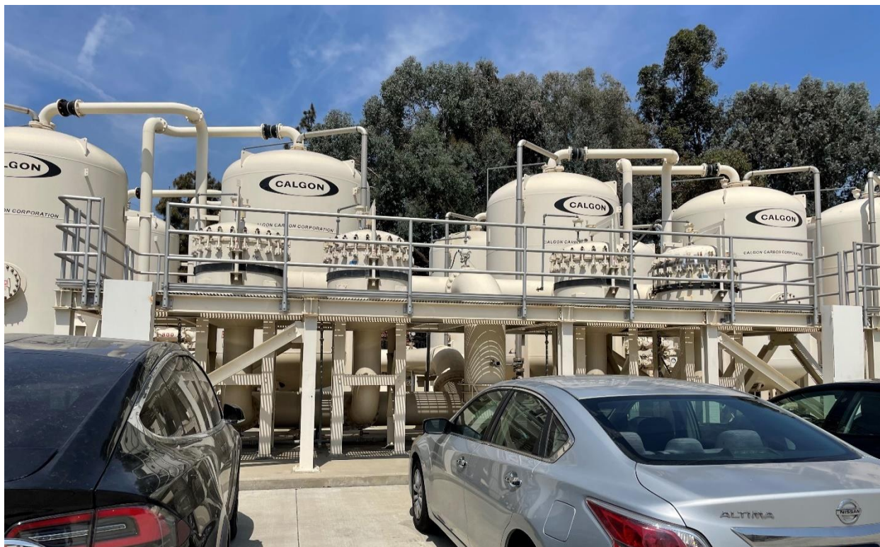
Figure 21 – Facing west, 10-micron filters in front of 8 pairs of IX vessels
