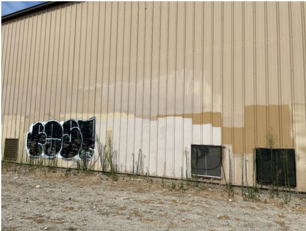
Figure 13 – Graffiti observed on the east side of the UV treatment building.
