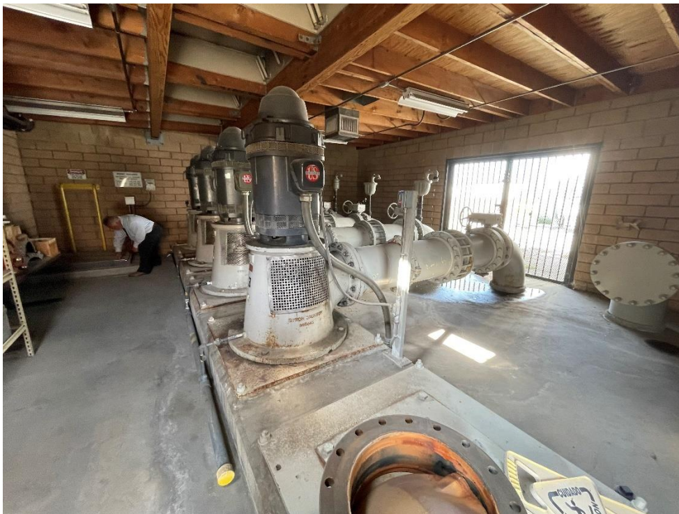
Figure 9 – Four pumps in the pump station, three in operation, and one in rest.
