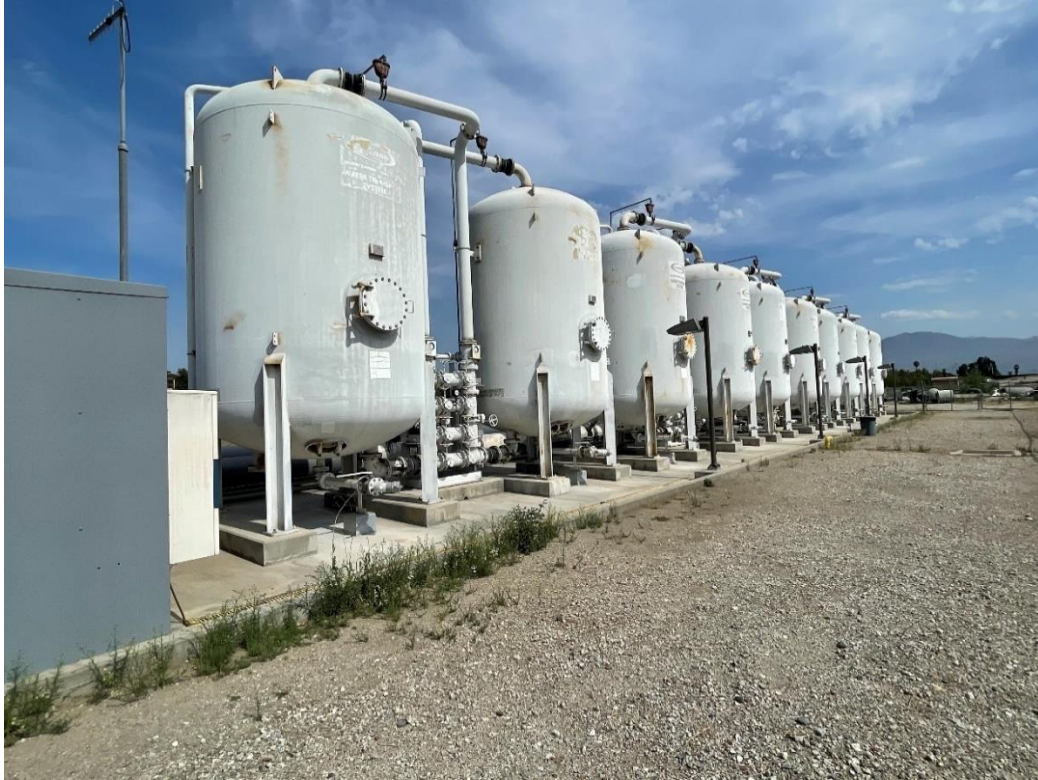
Figure 12 – Facing northwest, IX treatment vessels
