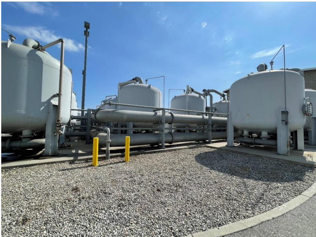
Figure 43 - Six pairs of IX vessels for perchlorate treatment
