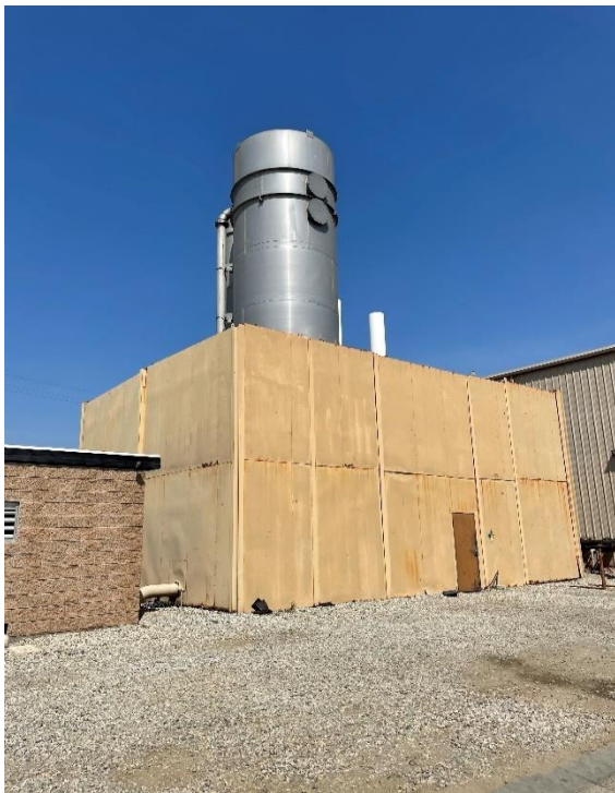
Figure 33 – Sound wall surrounding Air Stripping Tower #2
