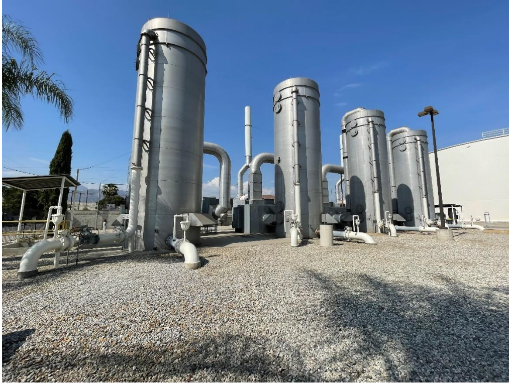
Figure 42 – Four air stripper towers
