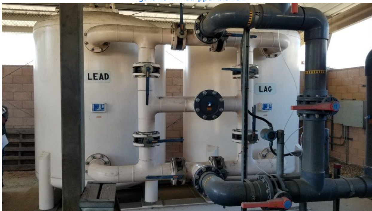
Figure 17. GWTP VGAC vessels.
