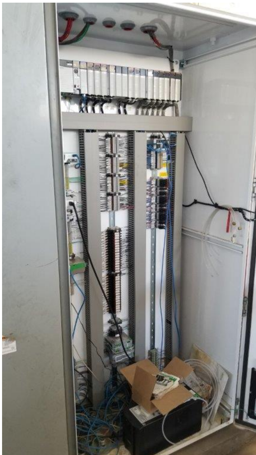
Figure 19. Interior of the GWTP control system cabinet.
