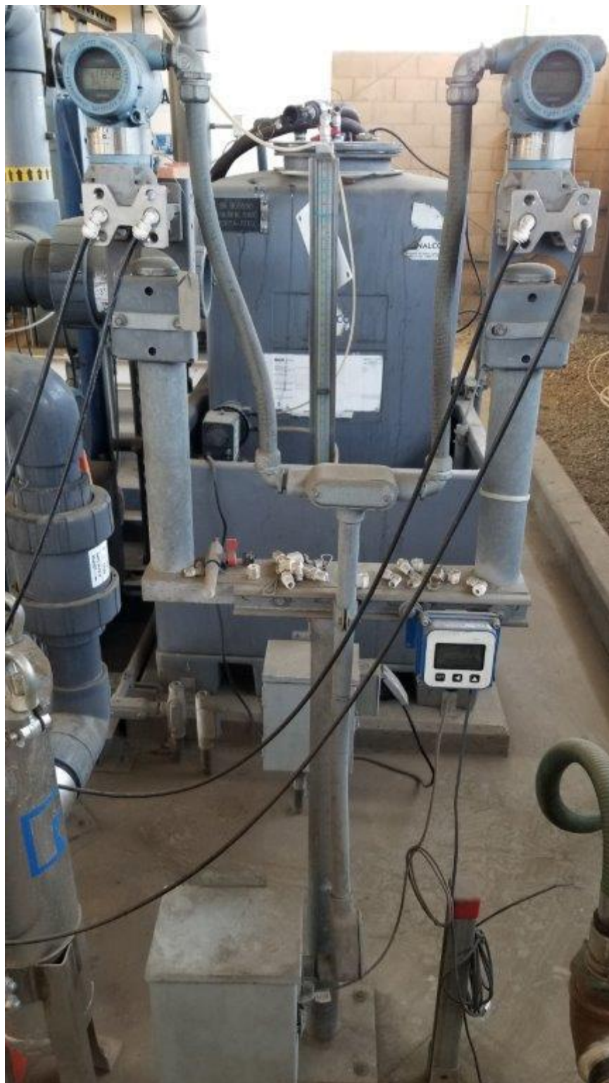
Figure 13. Pressure gages for influent.
