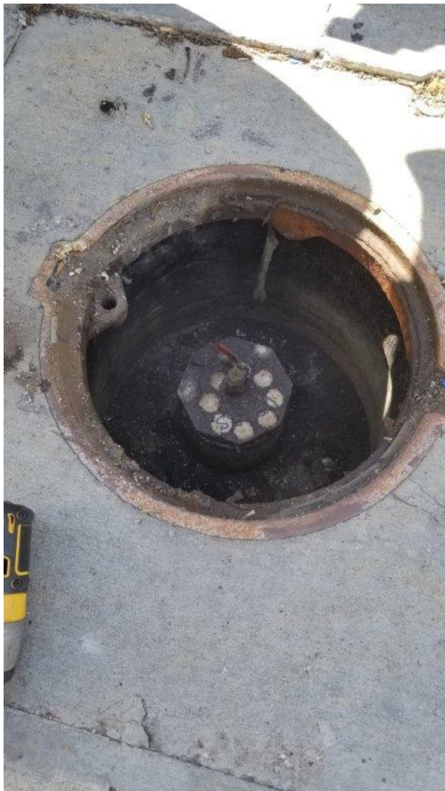
Figure 23. Close-up of VE-15S.
