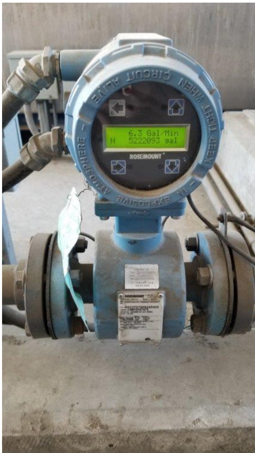
Figure 14. Influent flow meter.
