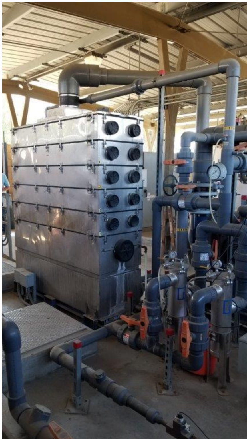
Figure 15. Air Stripper trays.
