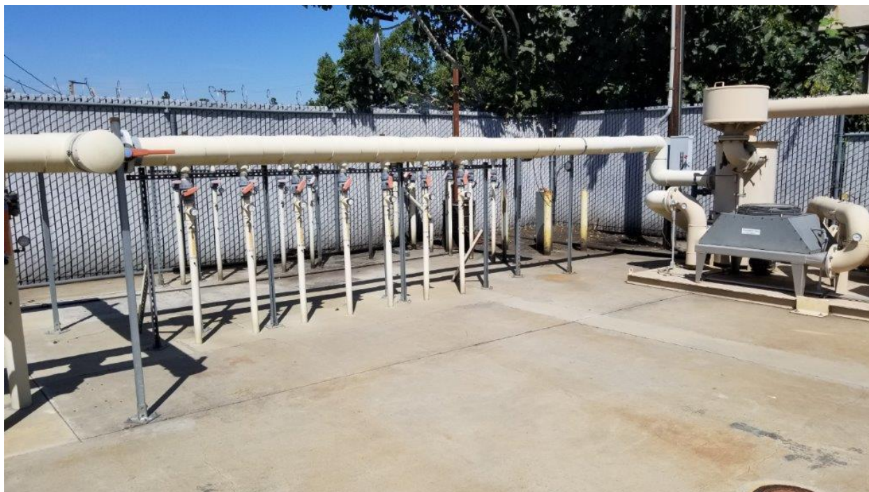
Figure 26. SVE sampling ports facing N.
