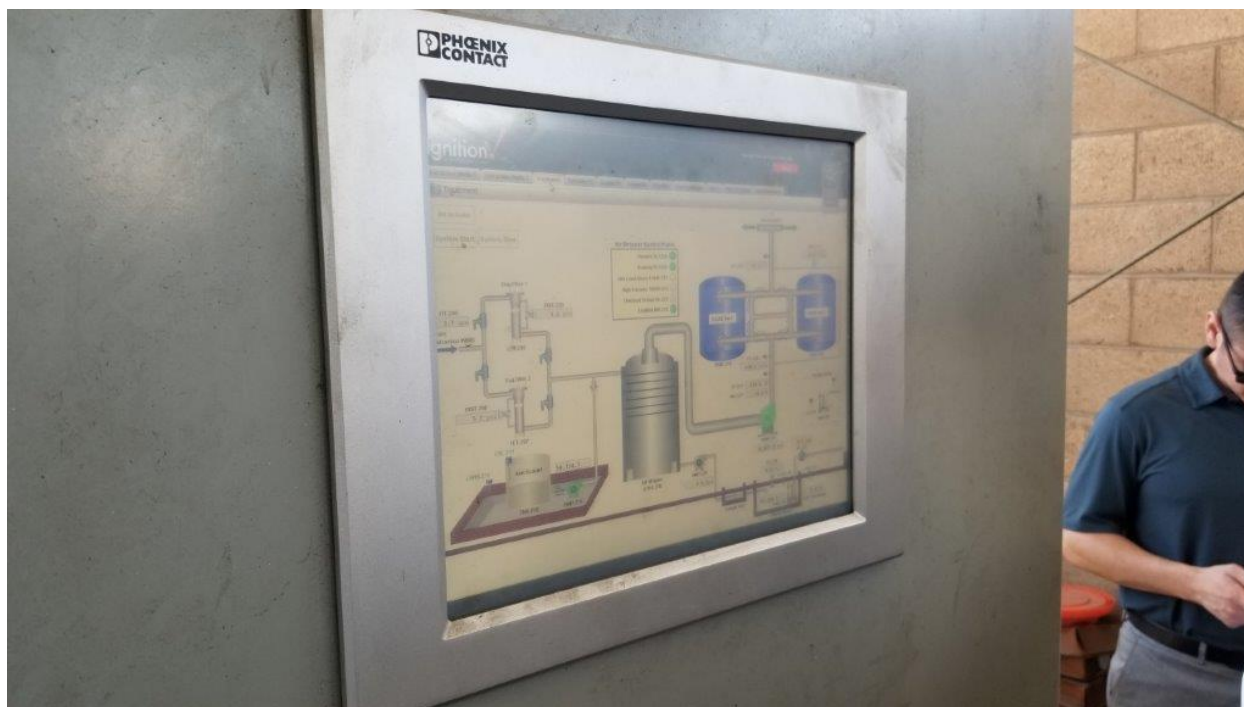
Figure 18. GWTP control panel.
