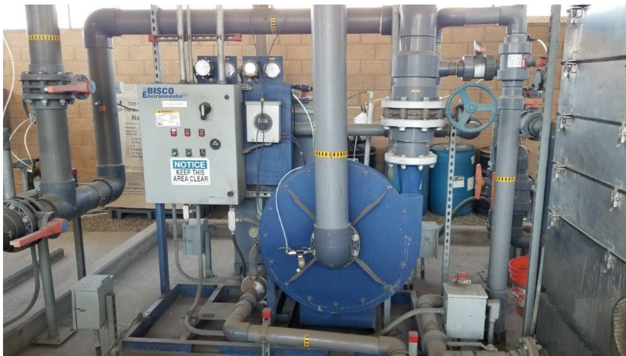
Figure 16. Air Stripper blower.
