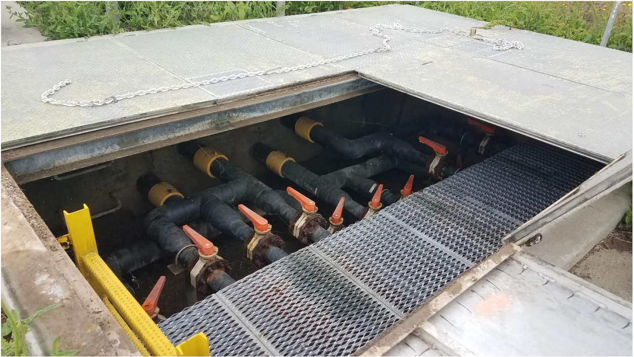
Valves and piping for the Ramparts Vault appeared to be in good condition
