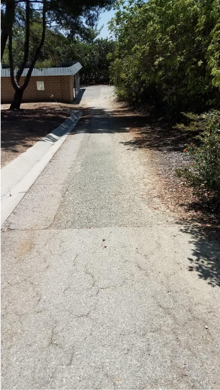
Access roadway with some brush growth toward end of road
