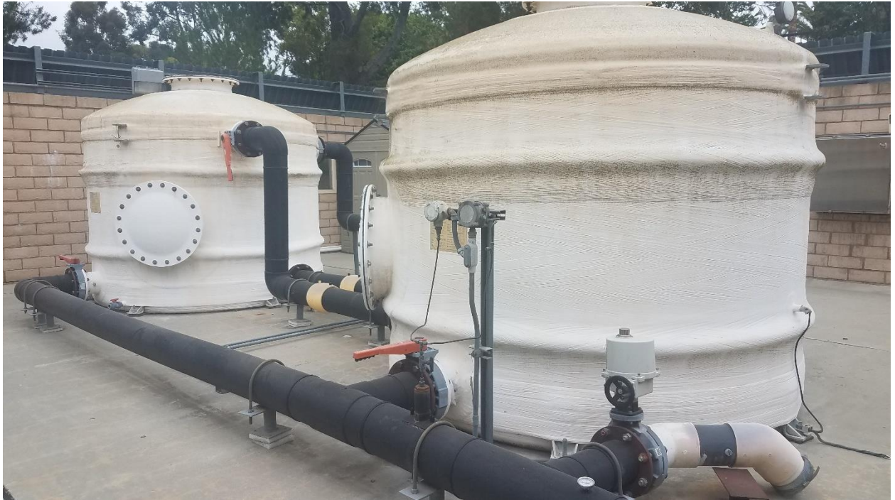
Remediation enclosure of the Gas Collection and Treatment System (GCTS)
