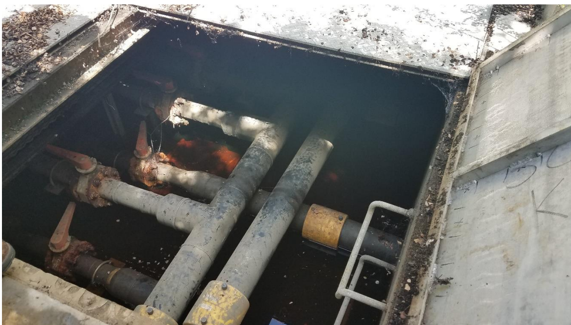
Valves and piping for the Ramparts Vault
