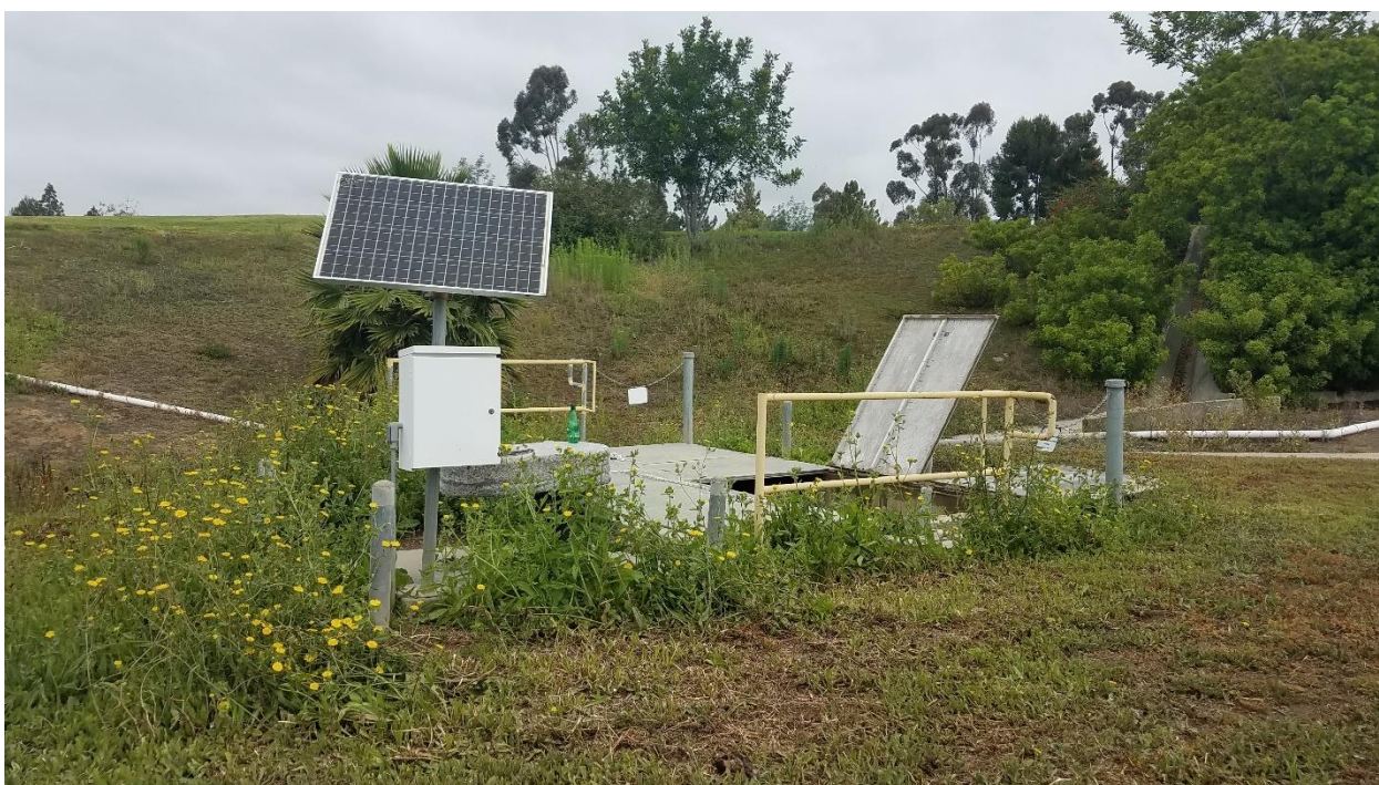
Ramparts Vault for the Gas Collection Treatment System (GCTS)
