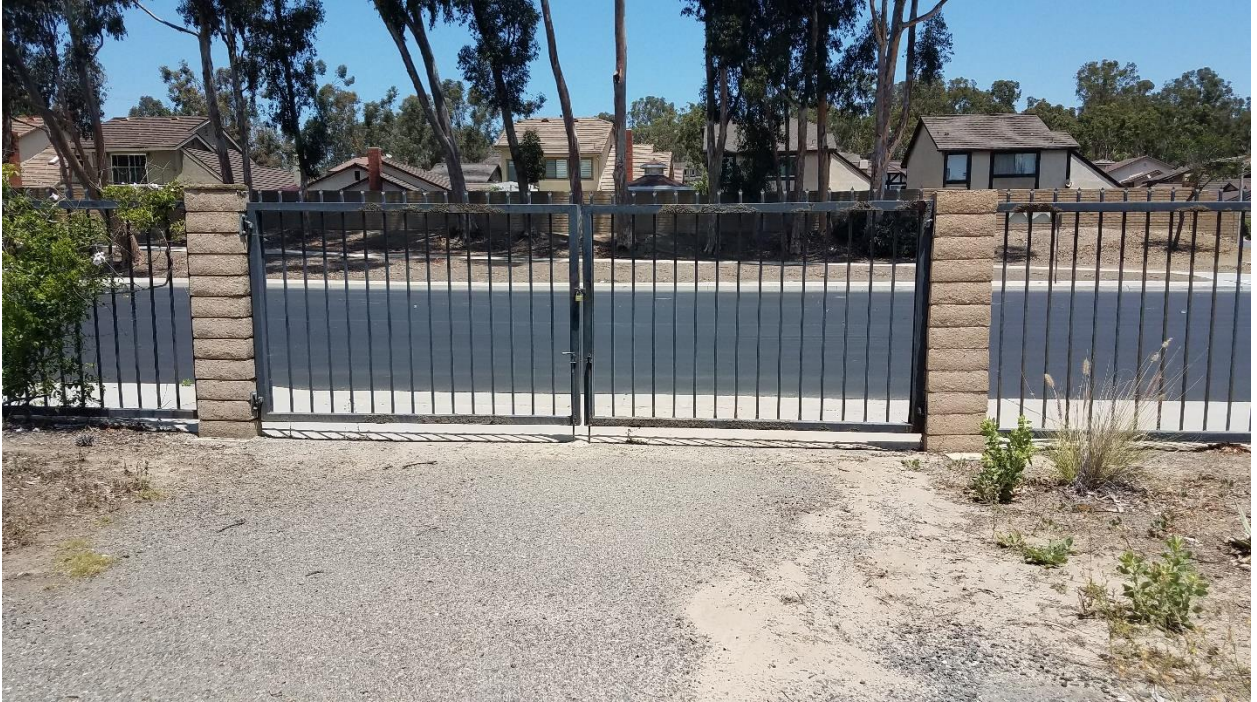
Access gate was also seen to be undamaged and secure for the site
