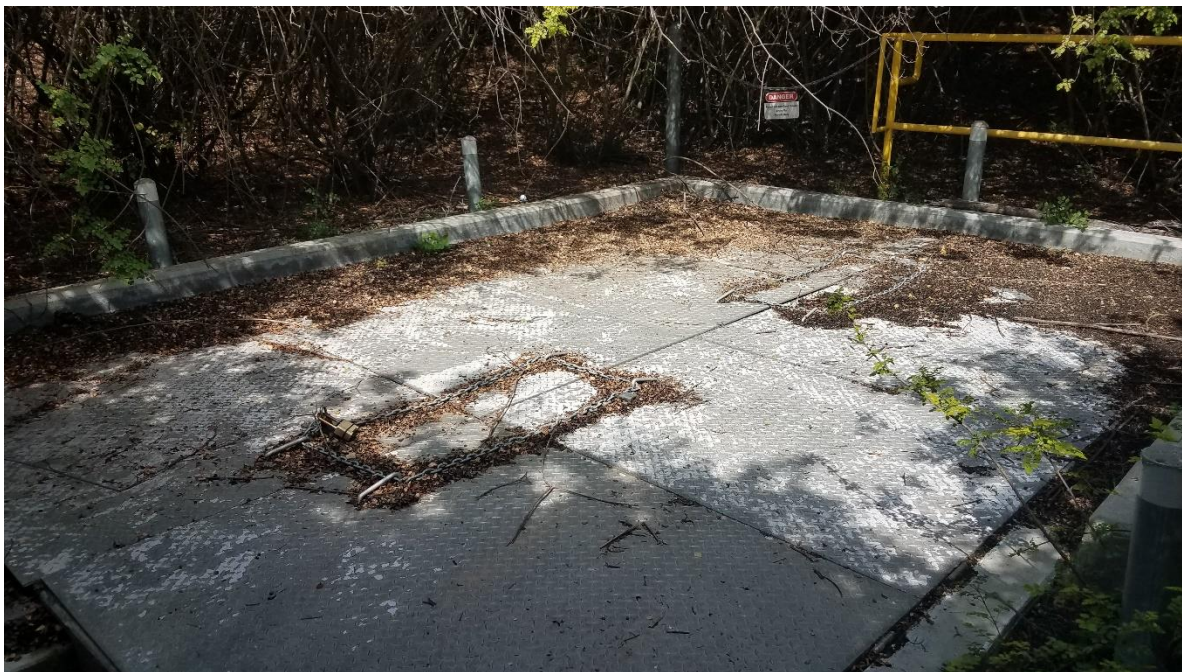
Los Coyotes Vault for the gas Collection Treatment System (GCTS)
