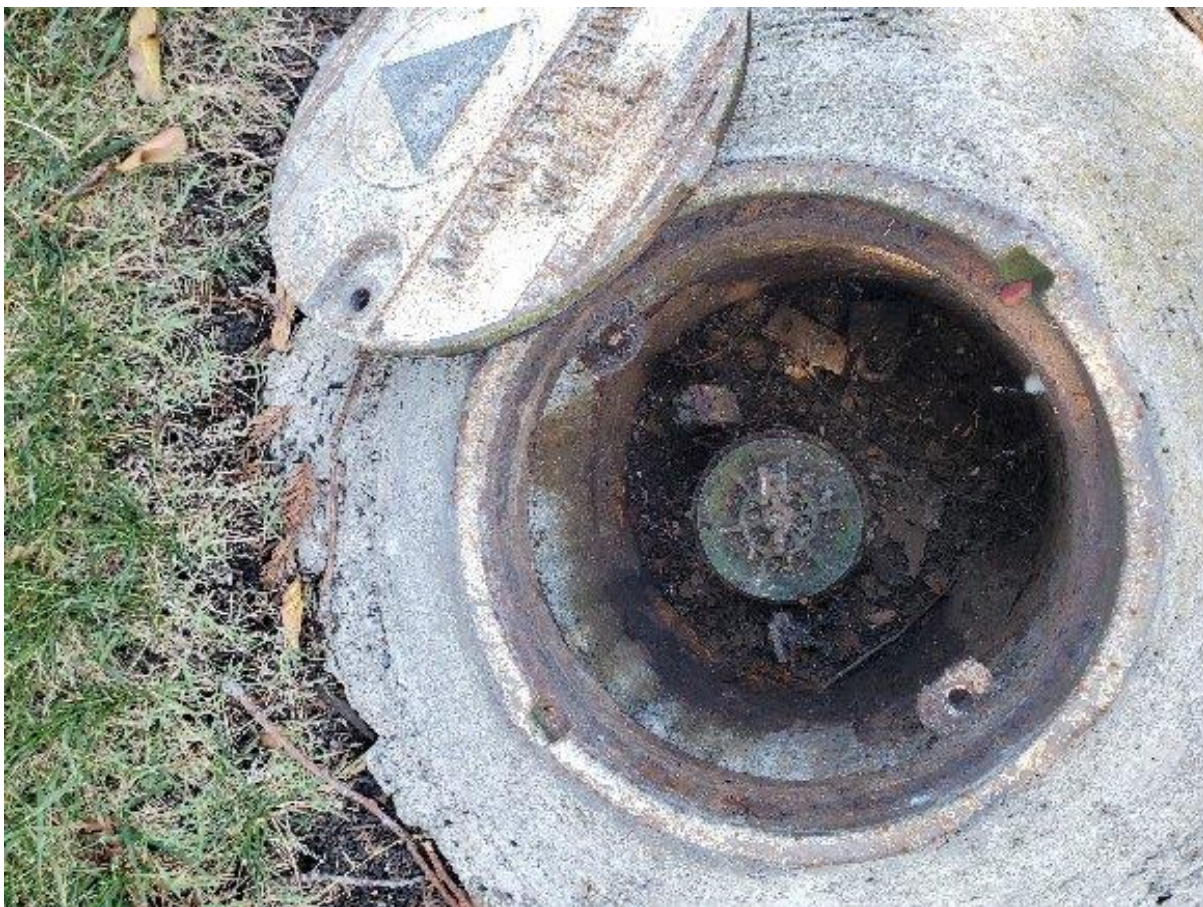
Photo 12 – Closeup of MW-17A with watertight cap
