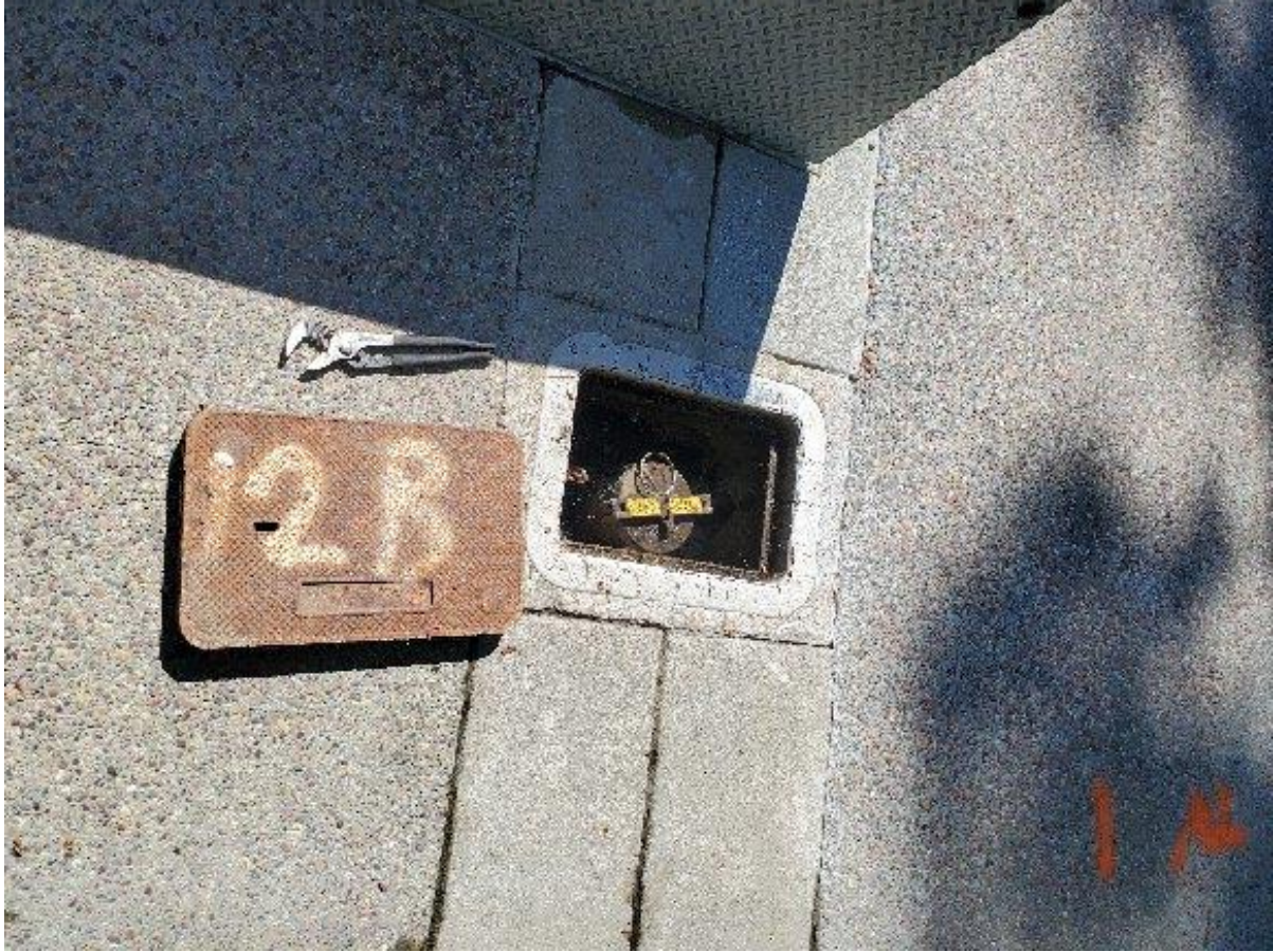
Photo 8 – MW-12B; 4-inch well with watertight cap.
