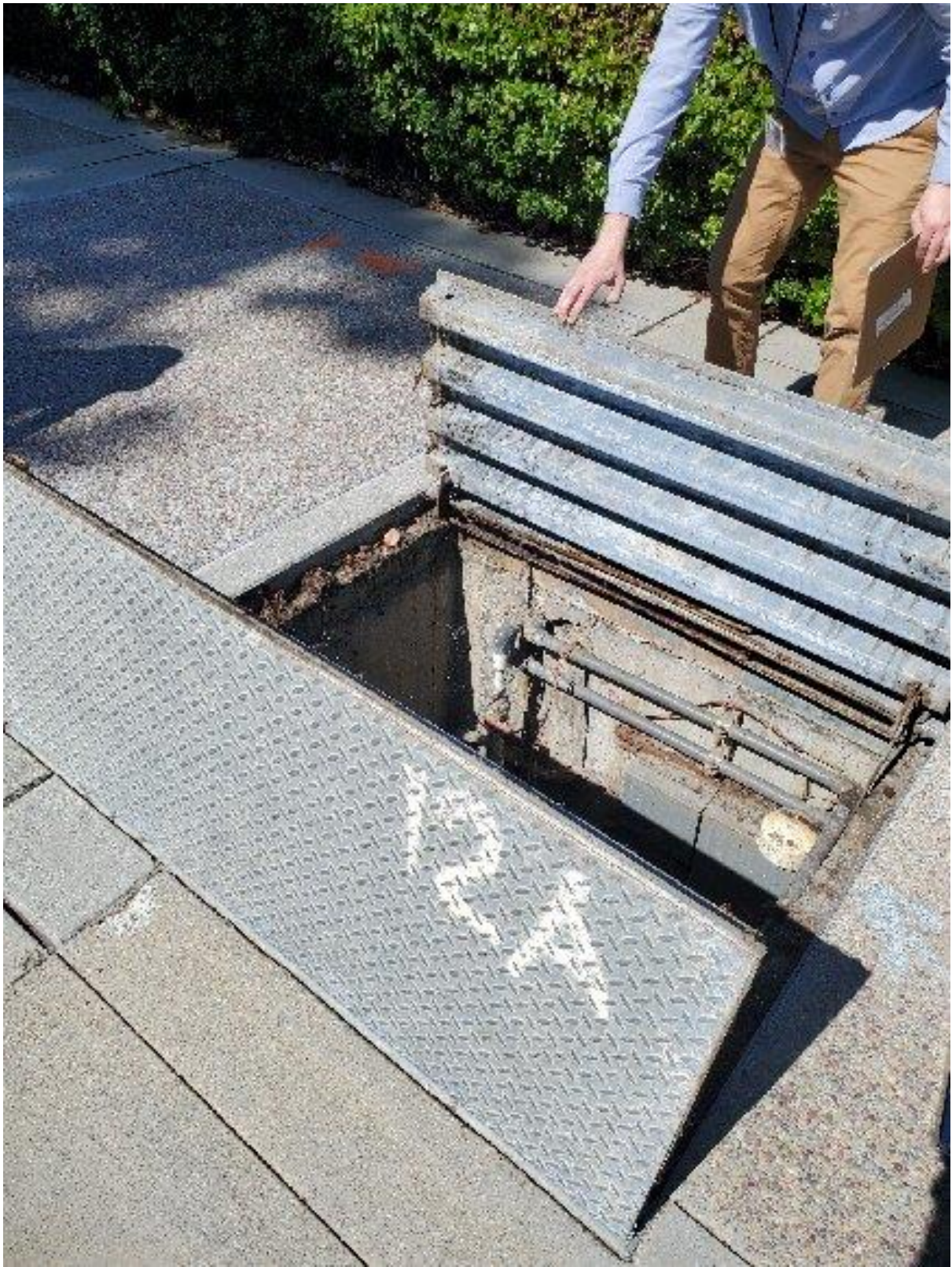
Photo 6 – Vault for MW-12A; facing SW.
