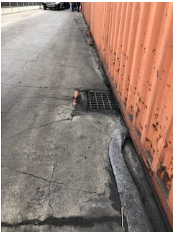
Photo 9. At SW-4 looking back, concrete has some cracks and repairs
