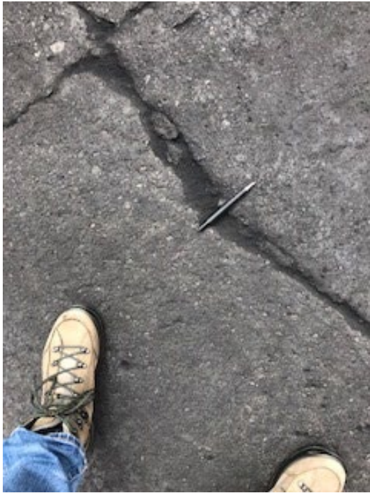
Photo 8. Largest crack observed
