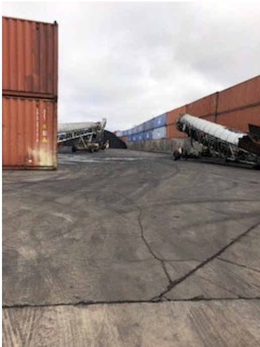
Photo 4. Example cracking (SW-3 looking north towards SW-4)
