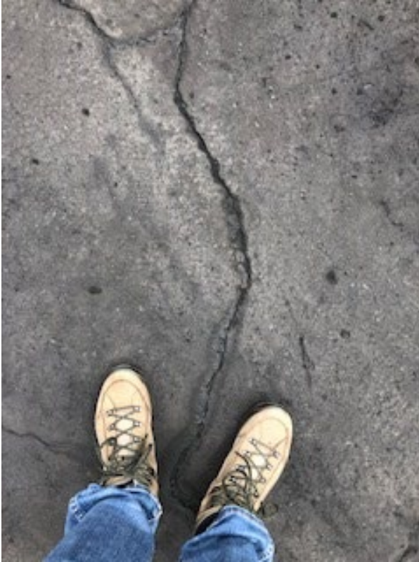
Photo 6. Cracking – no evidence of soil
