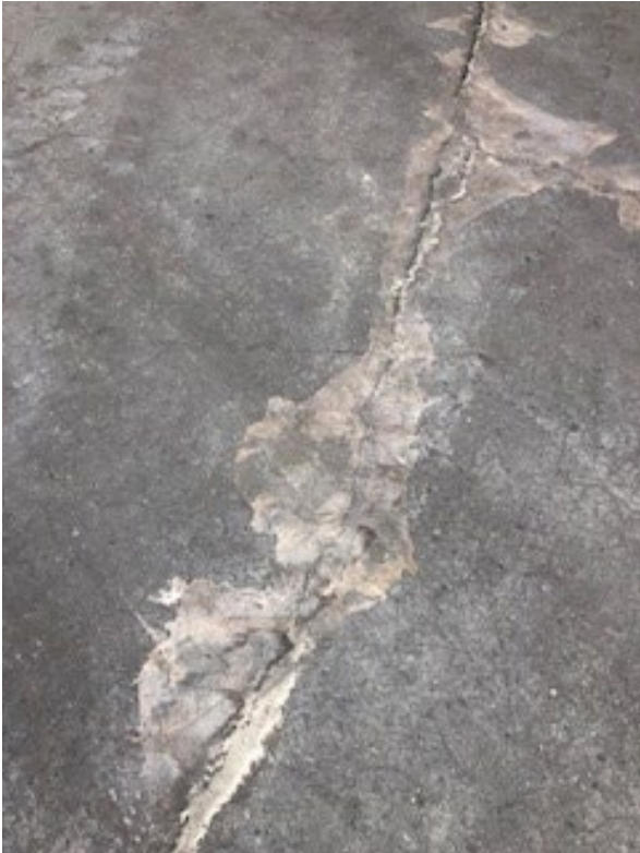
Photo 7. Cracking – previous repair
