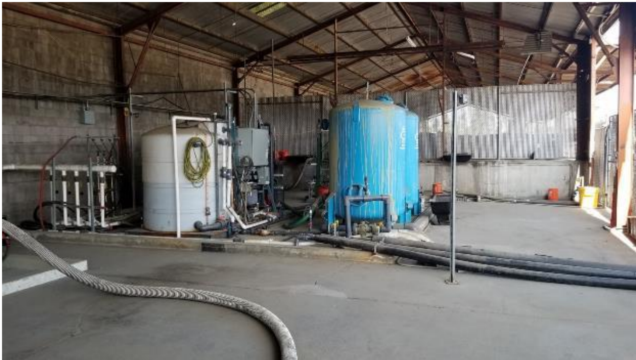
Figure 11. Overview of the groundwater extraction system. Facing west.
