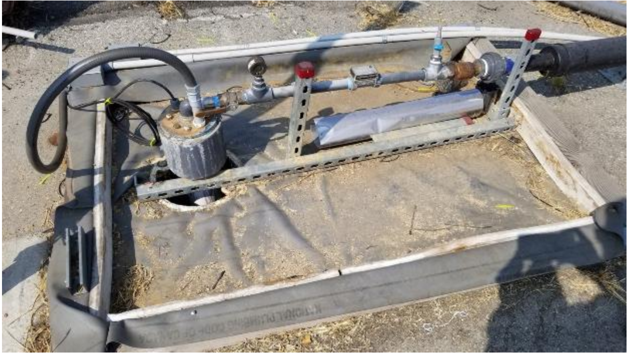
Figure 24. Groundwater extraction point installed for the ACB pilot test. Facing south.
