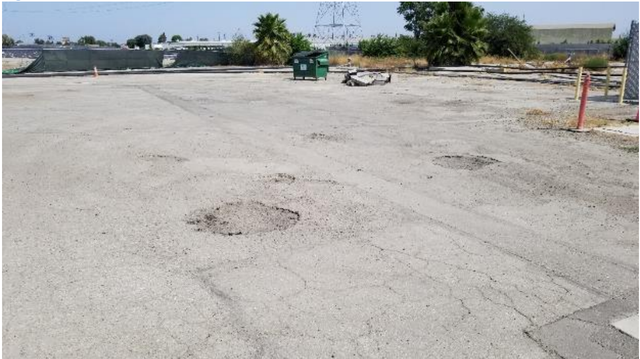
Figure 33. Potholes on the asphalt lot. Facing northwest.
