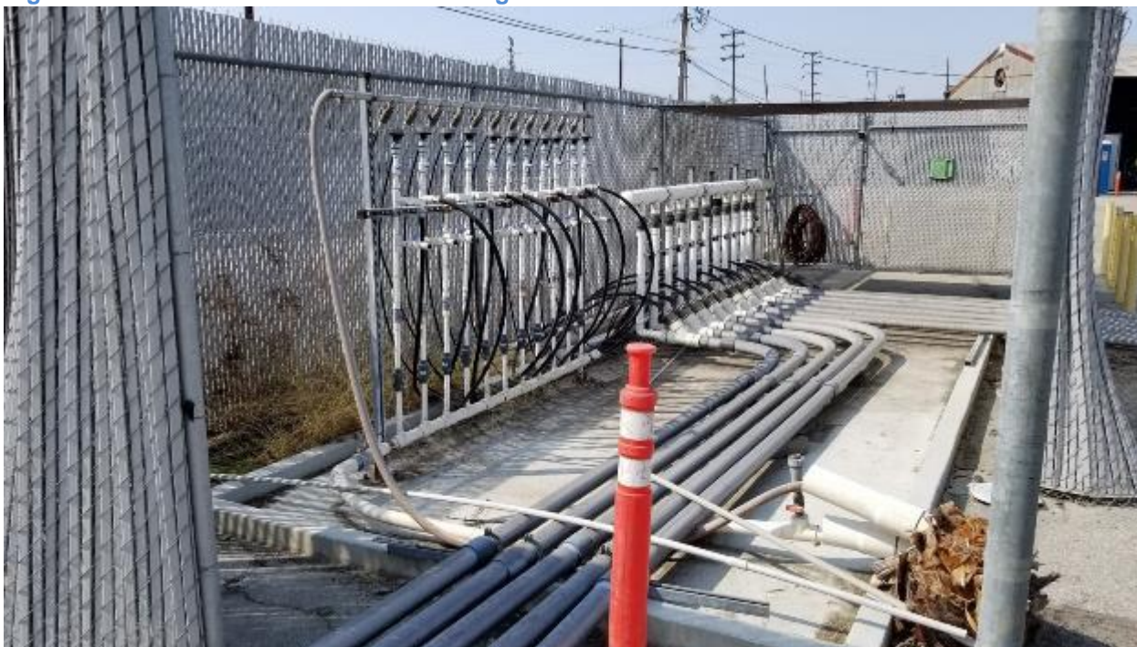
Figure 23. SVE pipe manifold. Facing southeast.
