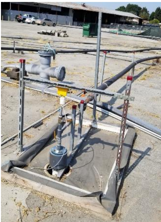
Figure 25. Groundwater injection point installed for the ACB pilot test. Facing southwest.
