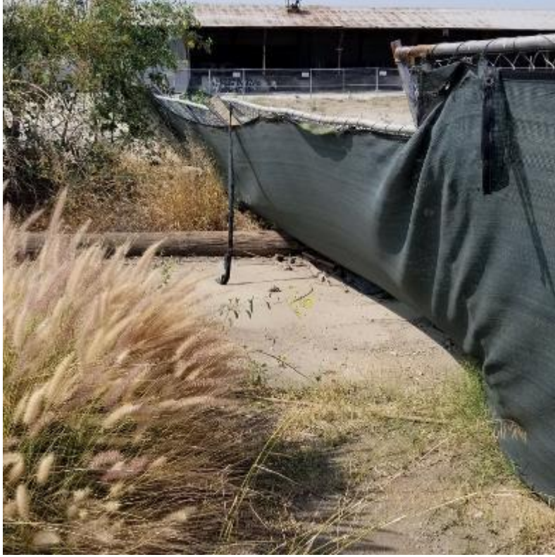
Figure 30. Length of fence partially toppled over along the west perimeter. Facing south.
