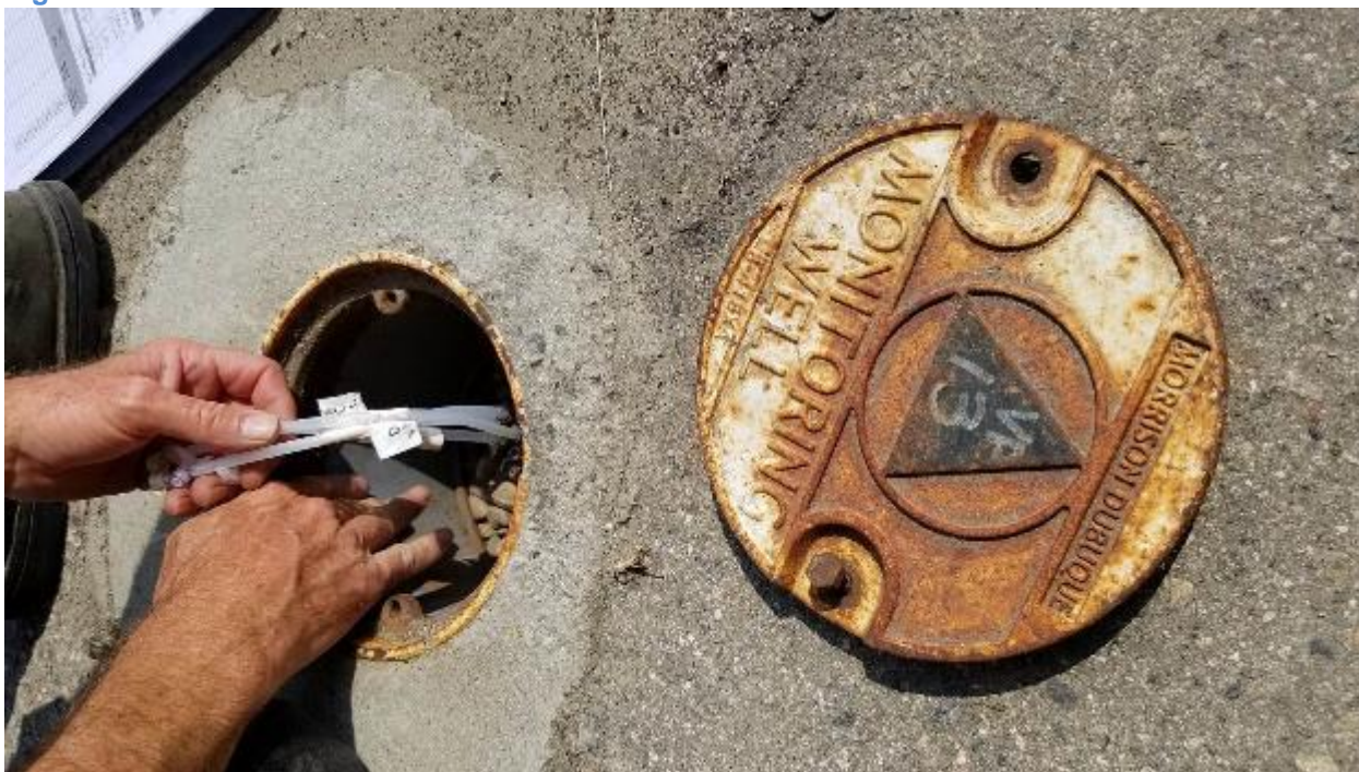
Figure 19. Vapor extraction point VP-13.
