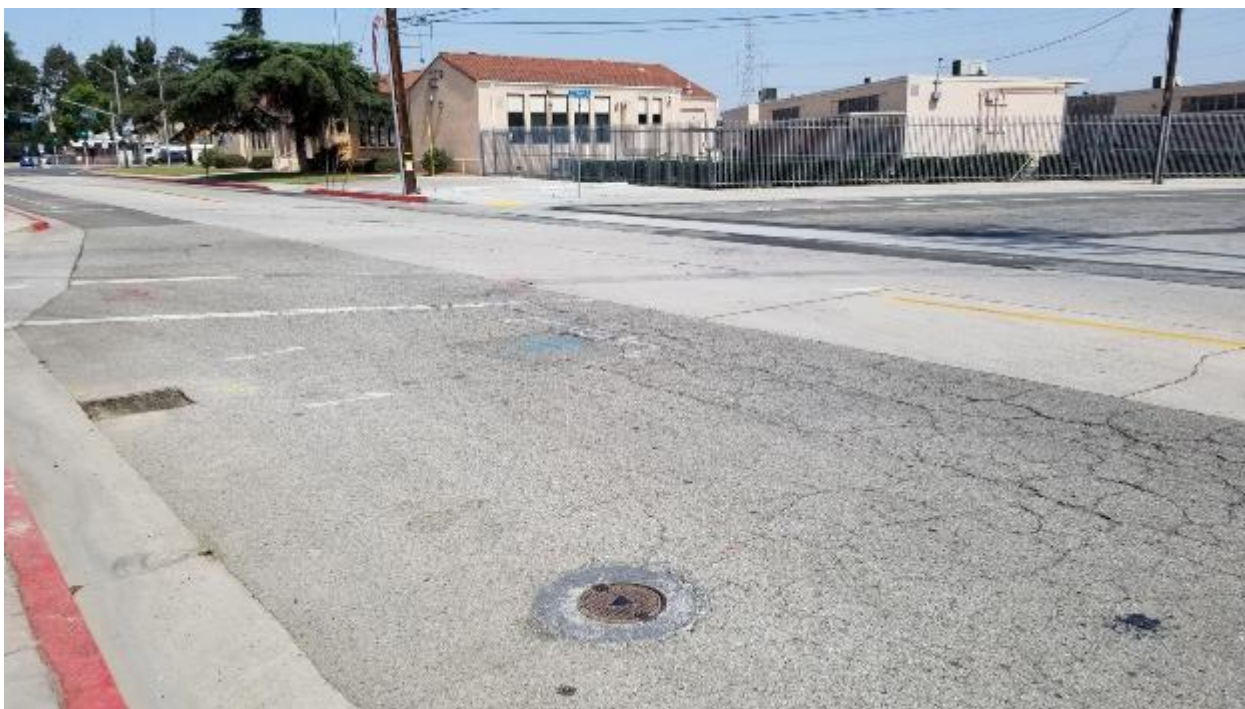
Figure 38. Vapor extraction point located on the southeast corner of Rayo Ave and Southern Ave. LAUSD property is in the background. Facing northwest.
