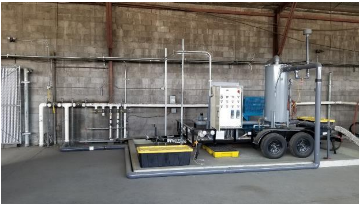
Figure 12. Overview of the SVE system. Facing south.
