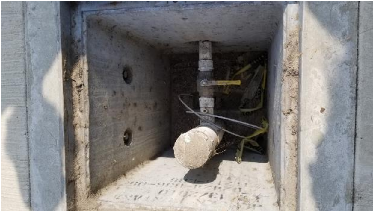
Figure 18. Vault interior SVE-9.
