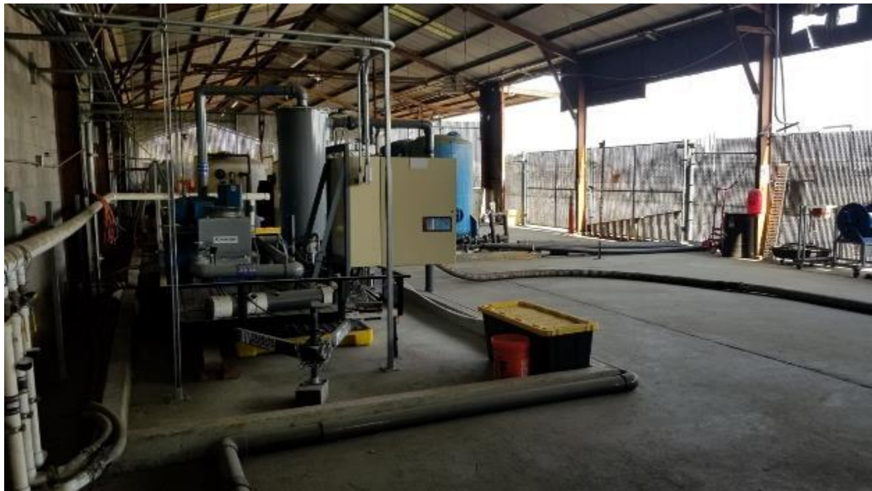
Figure 10. Overview of the treatment facility facing northwest.
