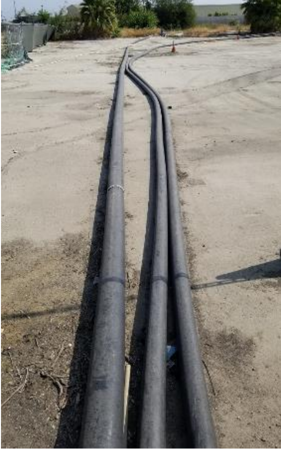
Figure 13. Groundwater extraction lines running to and from the treatment facility. Facing North.
