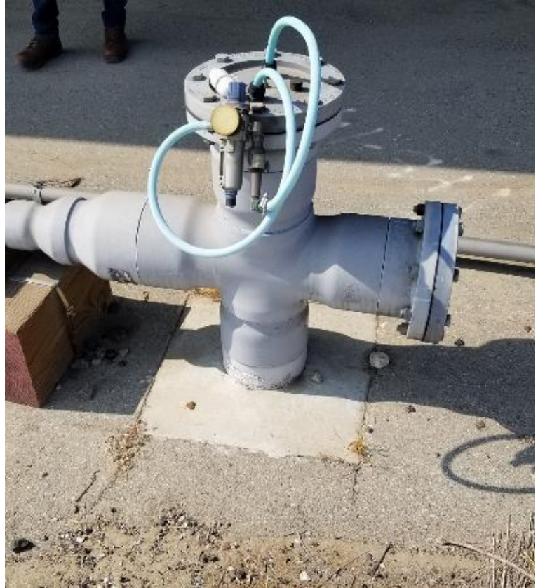
Figure 21. DPE-14 which is run as an SVE well now. Facing south.
