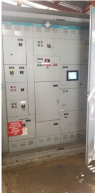
Siemens GWET System Control Panel
