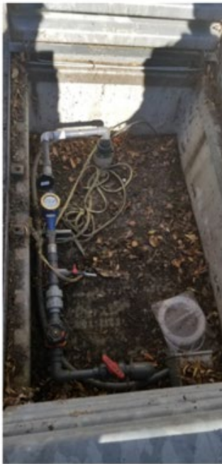
Siemens Extraction Well LF-12A Detail
