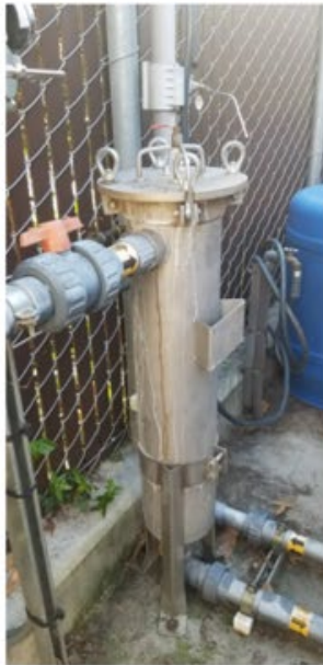
Intersil GWET Influent Bag Filtration Unit
