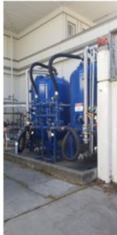
Siemens GWET GAC Vessels
