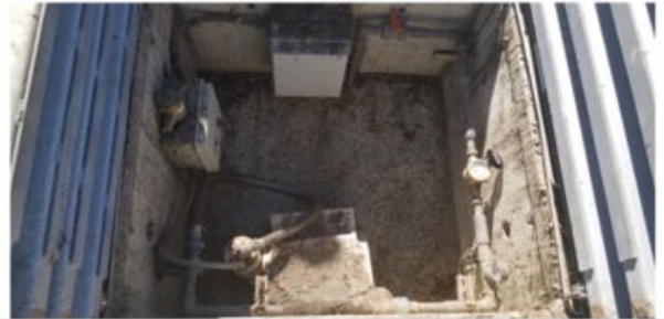
Intersil Extraction Well 12A Interior
