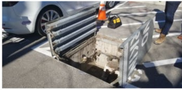
Intersil Extraction Well 12A
