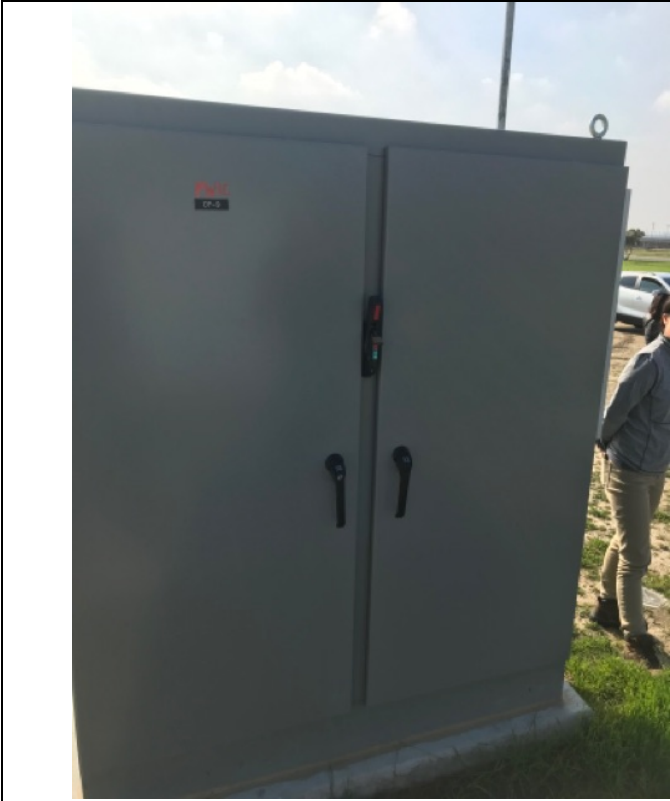
Extraction well electrical panel
