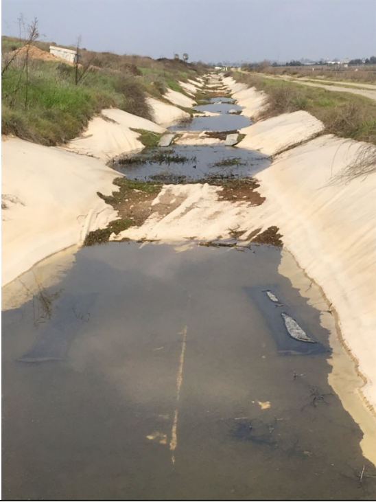
Subsidence in drainage ditch
