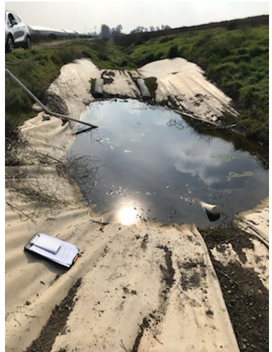
Subsidence since repair (~12 years and 1.5 ft depth)
