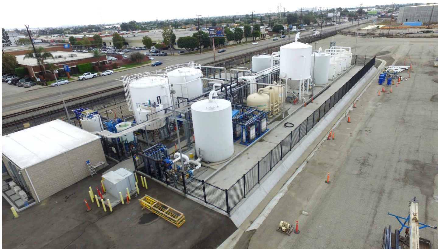
Figure 2. Dual-site groundwater treatment facility at the former Montrose property
