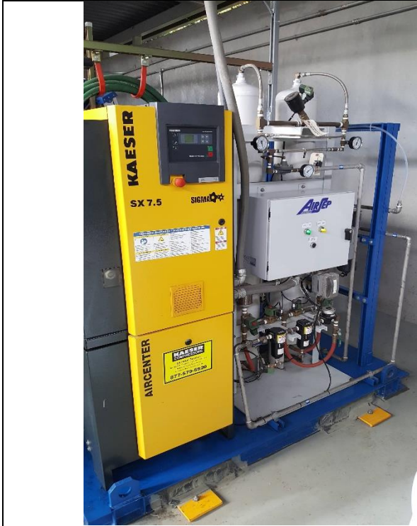
Vishay/SUMCO/Schlumberger – Groundwater Treatment System - Granular Activated Carbon Advanced Oxidation Process Oxygen Generator Unit
