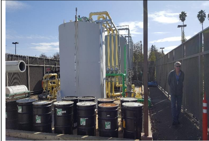
MEW Regional Groundwater Remediation Program - South of 101 Treatment System
