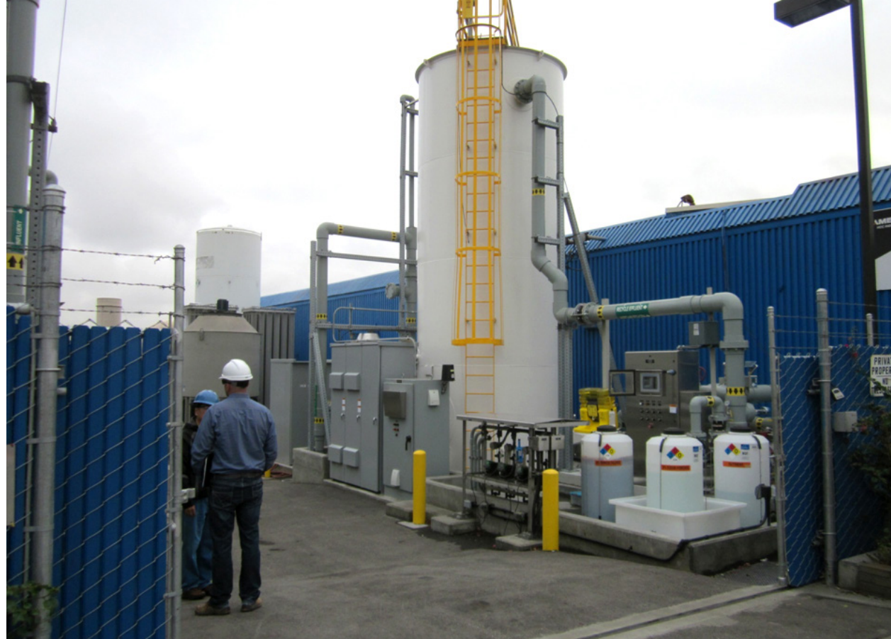
The El Monte Operable Unit Water Treatment System.
