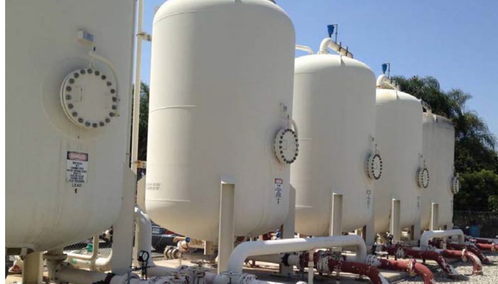
The South El Monte Operable Unit Water Treatment System run by the City of Monterey Park.
