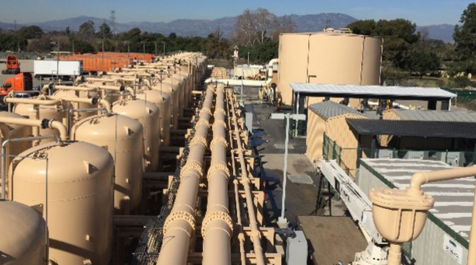
The Whittier Narrows Operable Unit Treatment Plant.
