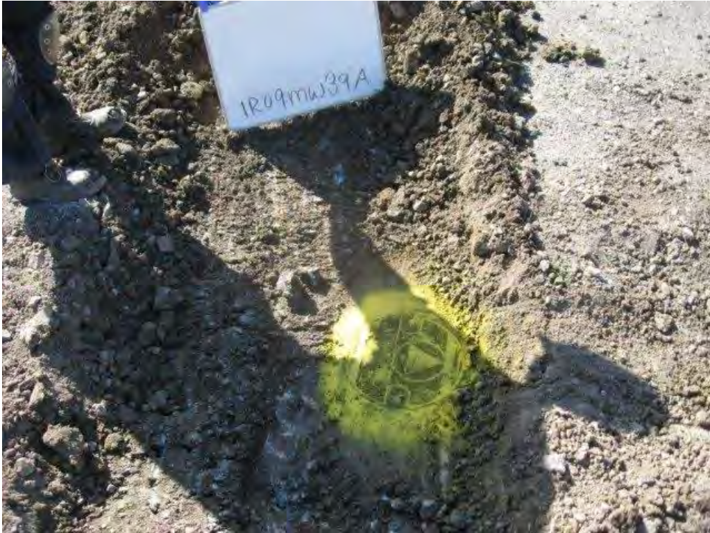
Photograph 53. Well IR09MW39A at Parcel G. Well box had been buried.
