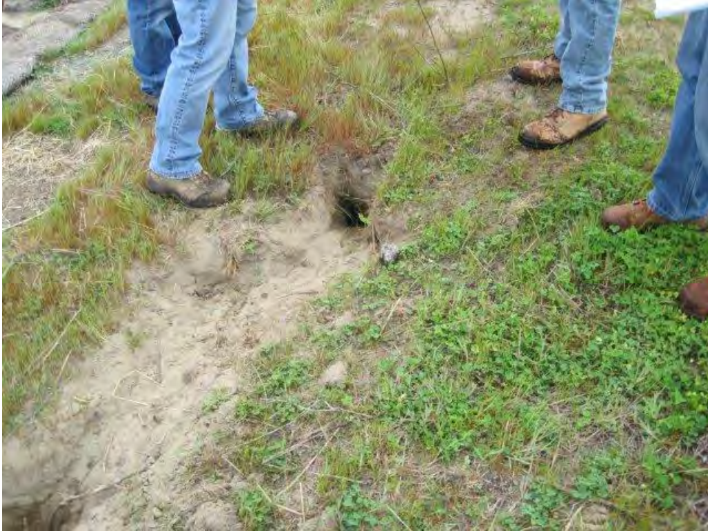
Photograph 15. Large, collapsed burrow near revetment crest in central portion. Second burrow entry at lower left corner of photograph. Burrow scheduled for repair.
