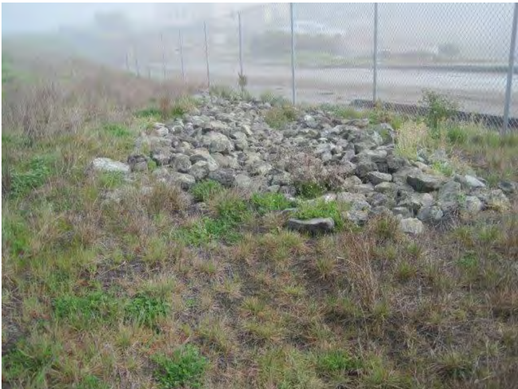
Photograph 24. Outfall protection at the end of the drainage swale. Perimeter fence and Donahue Street in the background.
