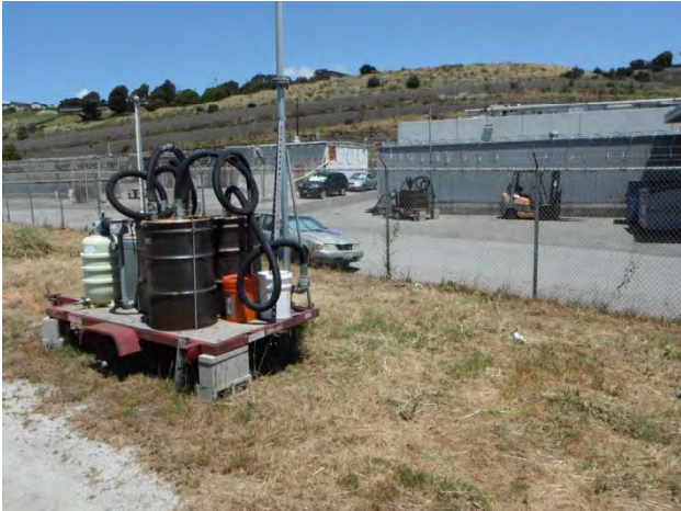
Active extraction at the perimeter of the landfill
