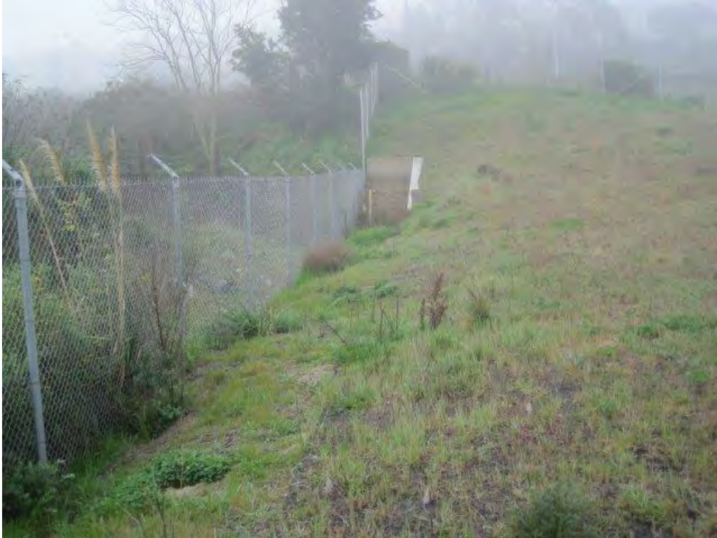
Photograph 19. Concrete retaining wall adjacent to the fence boundary with Parcel A in the southwestern portion of the cover.
