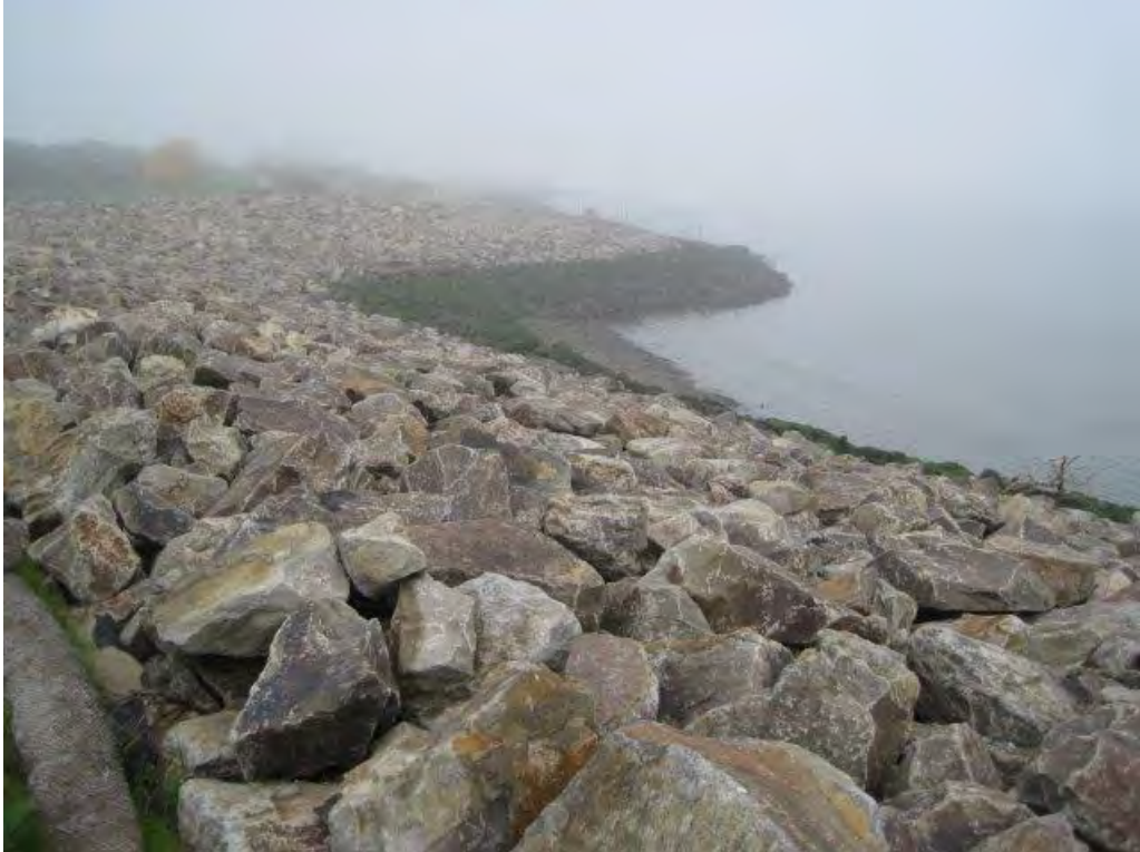
Photograph 10. Revetment looking northwest at the western end of the revetment from western portion.
