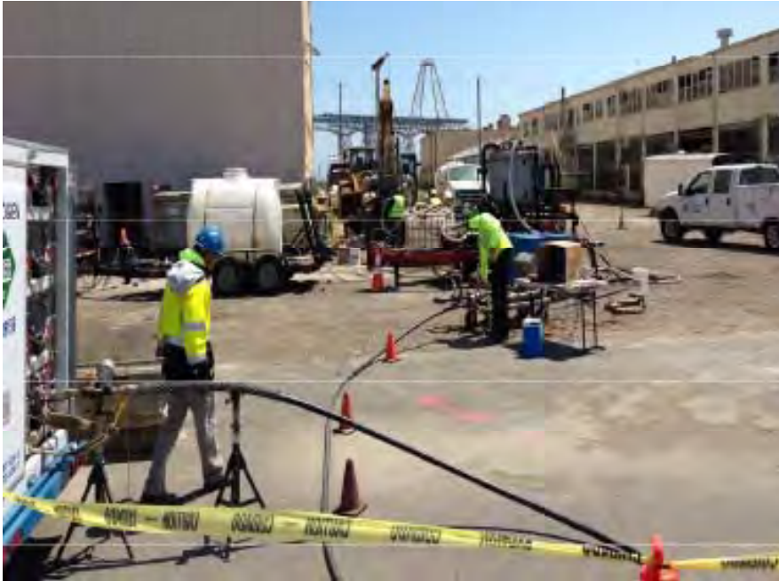
Injection of lactate solution in wells near Building 258 in the RU-C2 areas
