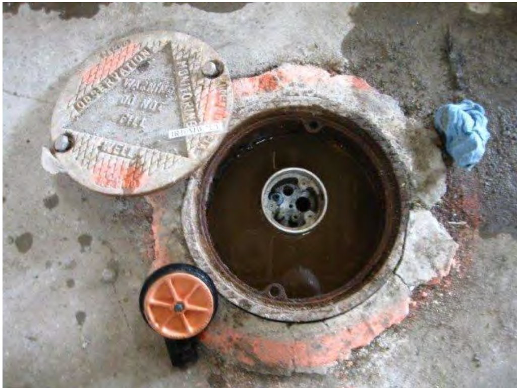
Photograph 58. Well IR10MW71A at Parcel B. Water inside well box.
