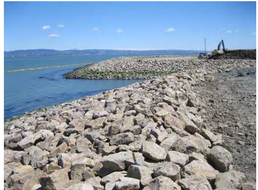
Completed shoreline revetment; all debris removed and shoreline stabilized with riprap rock
