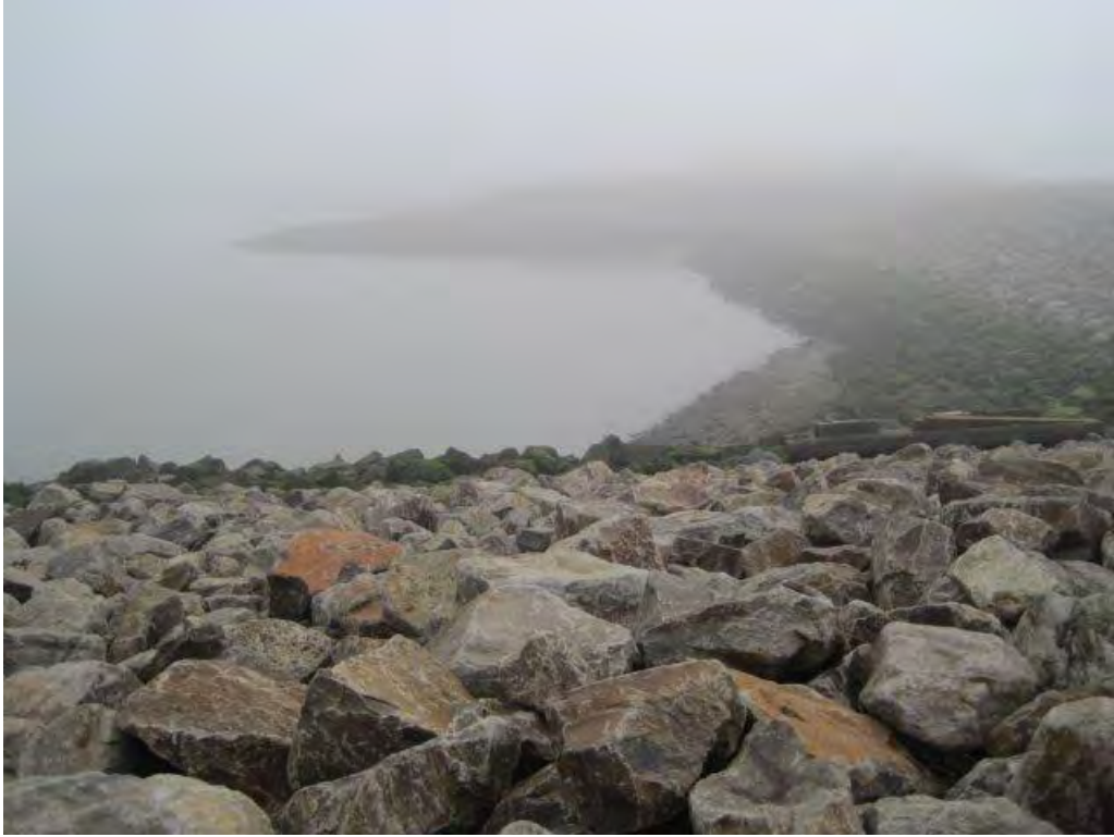
Photograph 9. Revetment looking east from near the western end. Accumulation of sand at revetment toe.
