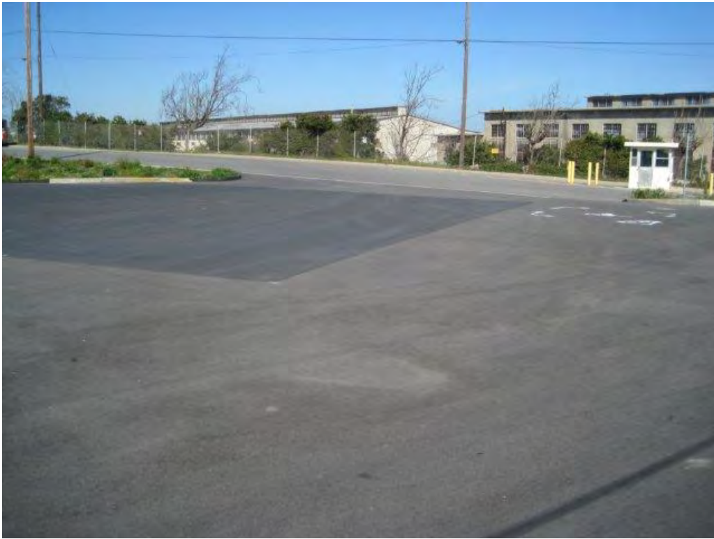
Photograph 41. Asphalt pavement and seal coat (darker gray) covers in parking lot at Building 101 at Parcel UC-2. Looking north.
