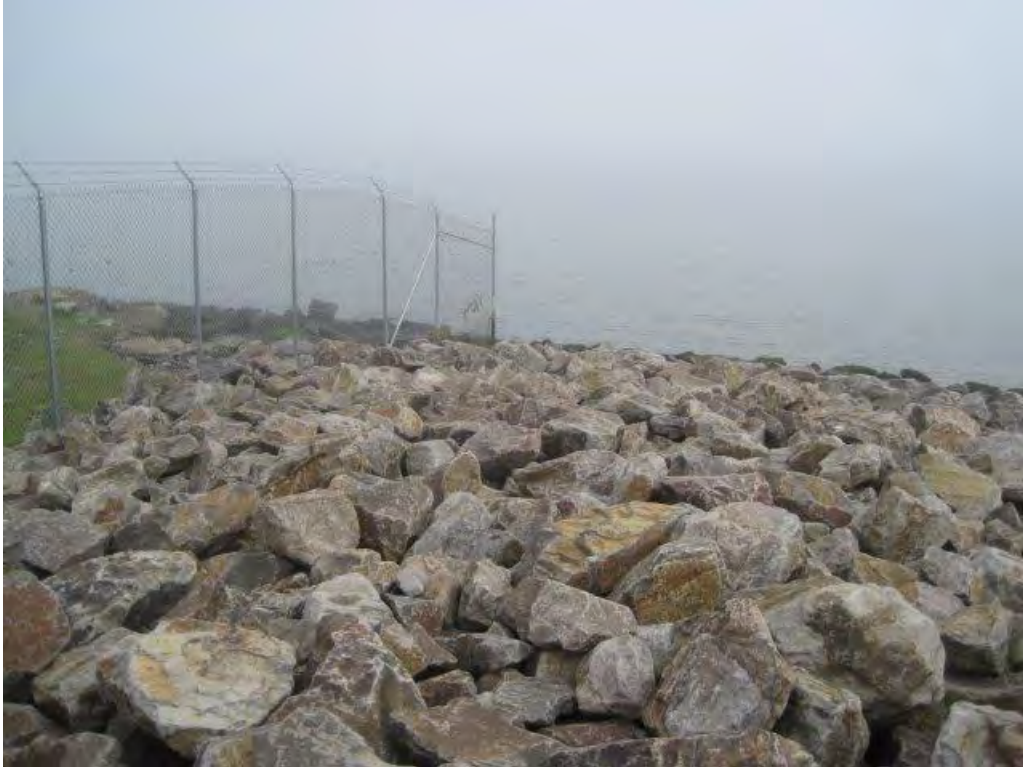
Photograph 13. End of the western boundary fence looking north down the revetment slope toward the bay.
