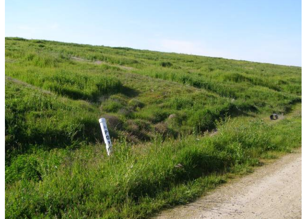
Subsidence on east slope and squirrel bait location
