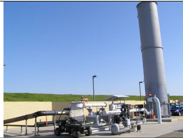
Gas flare influent piping
