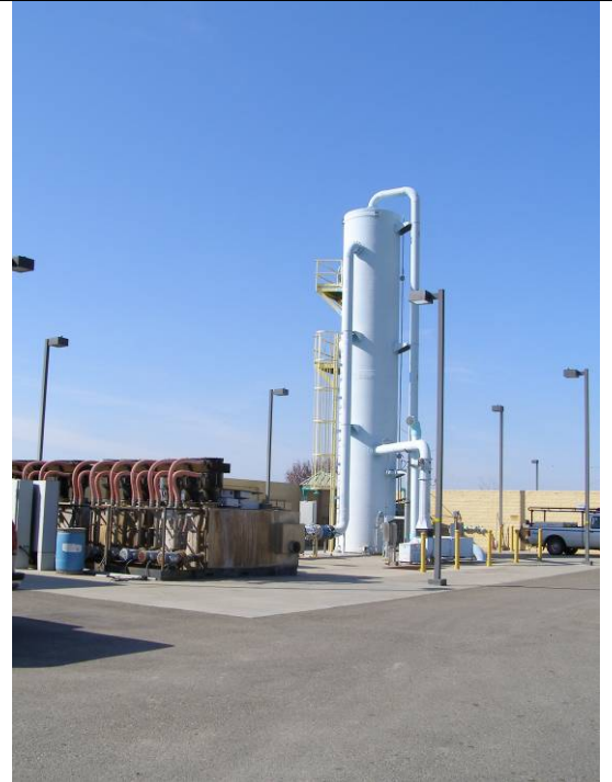
Packed Tower Aerator
