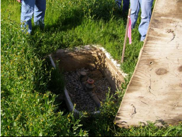
Gas extraction well
