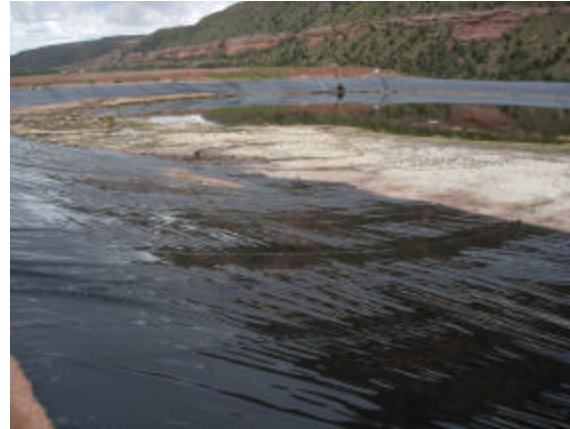
CRP #4 Interior Liner Trampoline Effect
