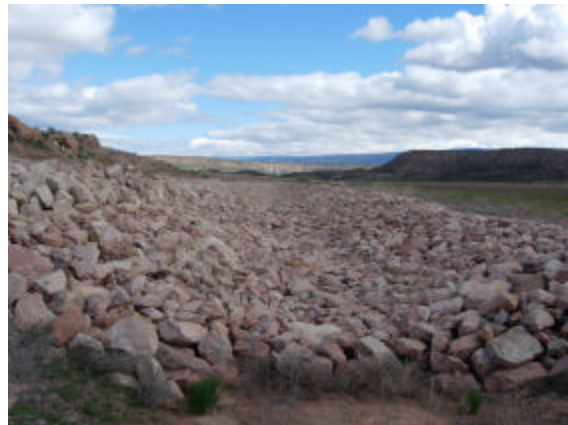
Club Mesa Tailings Piles 1& 2 Storm Water Run-Off control
