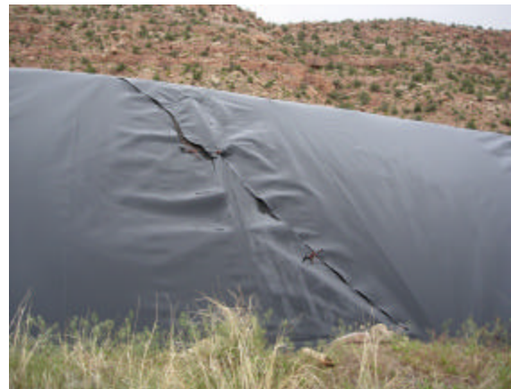
Club Ranch Pond CRP #4 Exterior Liner Failure
