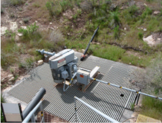
Club Mesa Tailings Pile 1 &2 Seep Collection Sump #1
