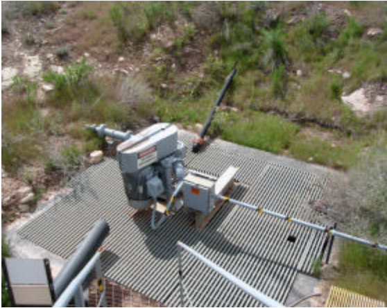
Club Mesa Toe Drain Collection Sump
