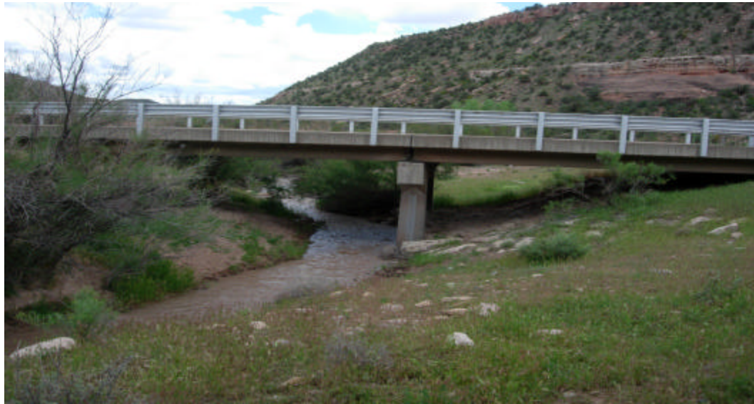
Looking west from Atkinson Creek Disposal Area at Atkinson Creek and Colorado Highway 141 overpass.
