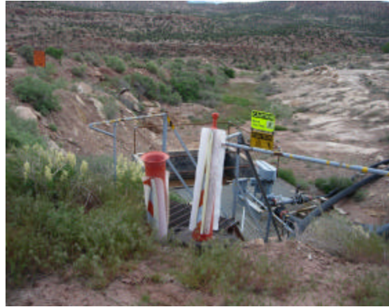
Club Mesa Toe Drain Collection Sump
