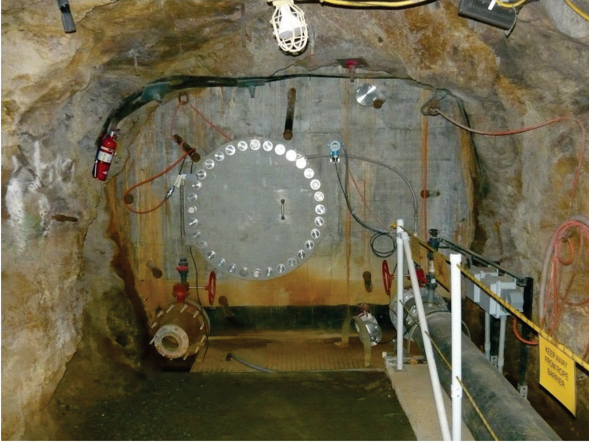
Argo Tunnel Flow Control Bulkhead (photo not taken at time of inspection)
