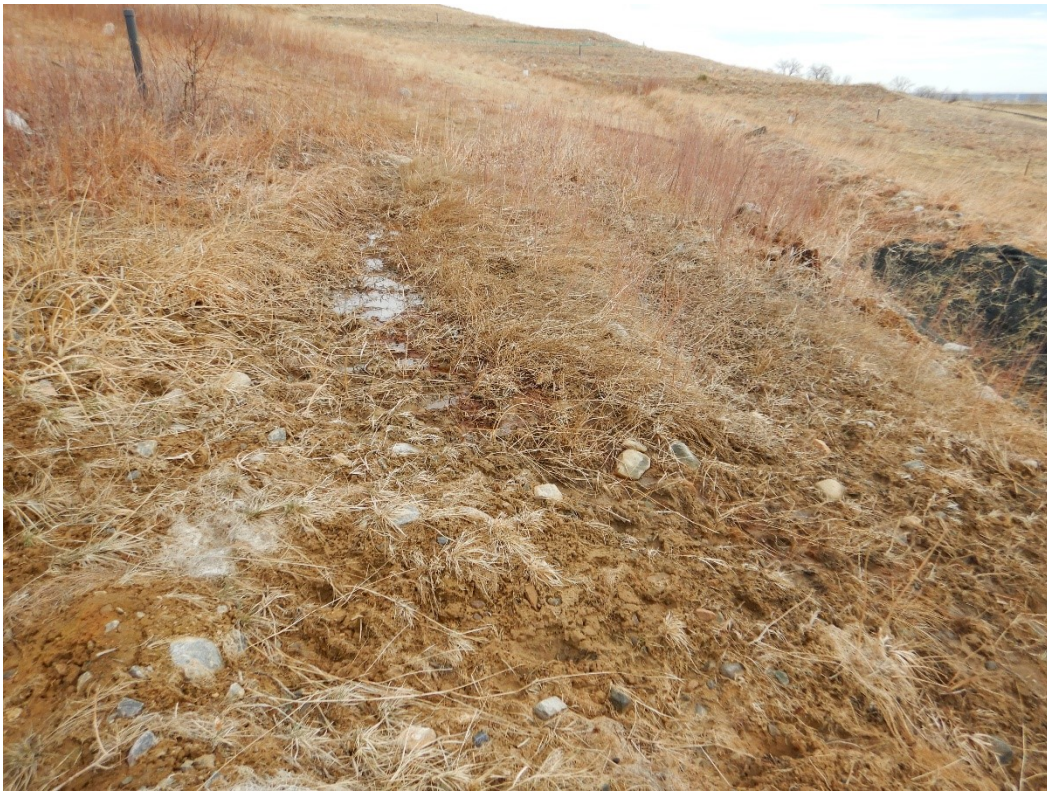
Figure 6. Looking East at Seep 4 and the Surrounding Area, Which Was in Good Condition
