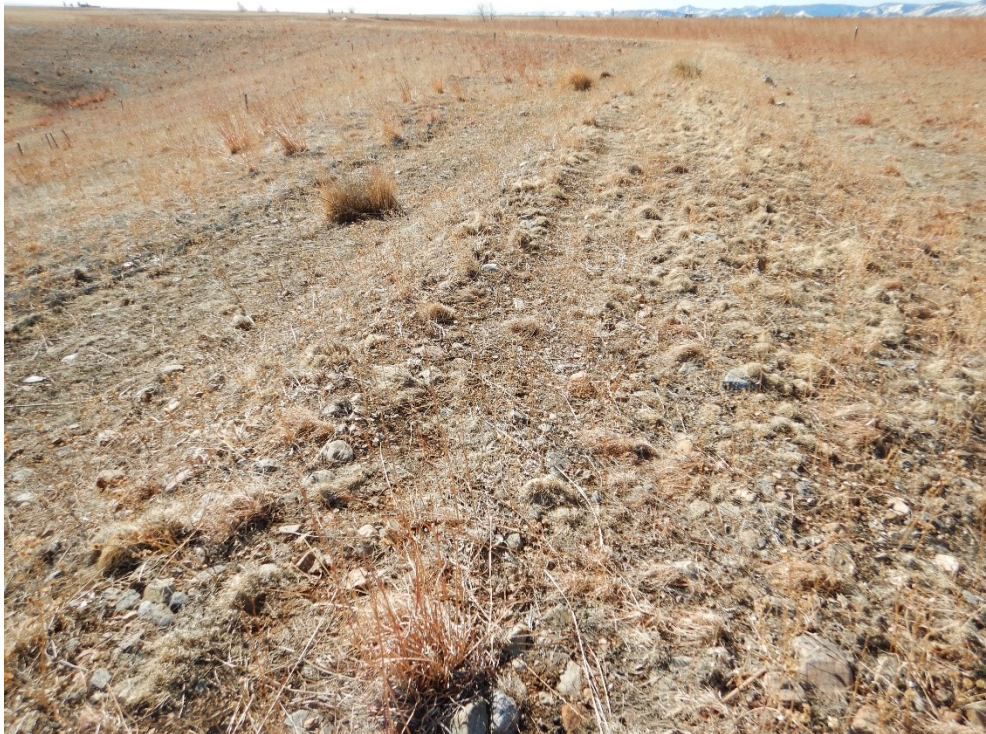
Figure 1. Looking Southwest at the Present Landfill Diversion Berm Located Between the East Face Slope and the Top of the Landfill Cover, Which Was in Good Condition
