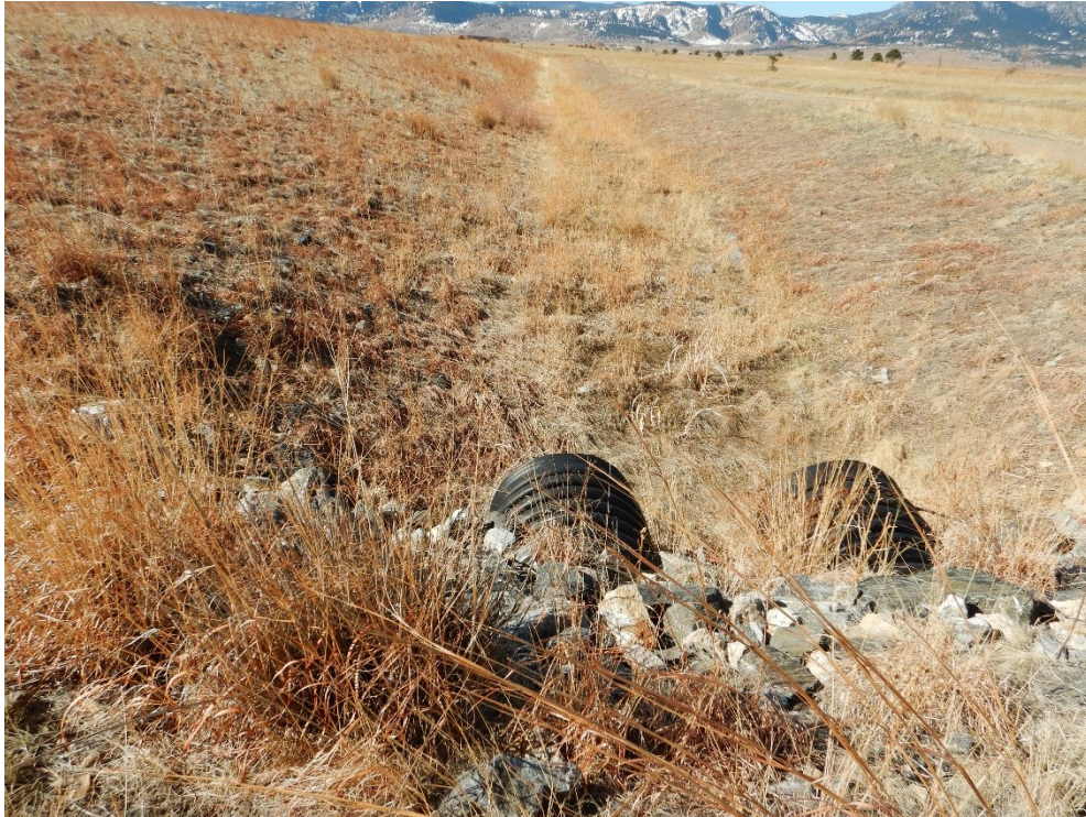
Figure 3. Looking West at the Northern Vegetation-lined Perimeter Channel and North Slope of the Present Landfill Cover, Which Were in Good Condition
