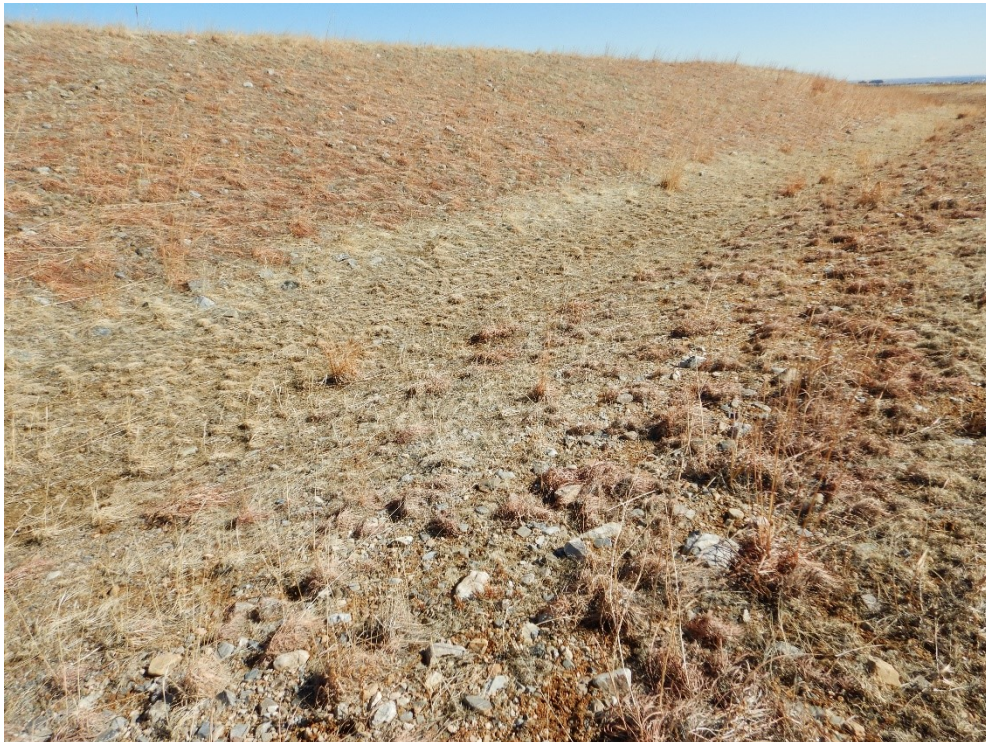
Figure 4. Looking Northeast at the Southern Vegetation-lined Perimeter Channel and South Slope of the Present Landfill Cover, Which Were in Good Condition
