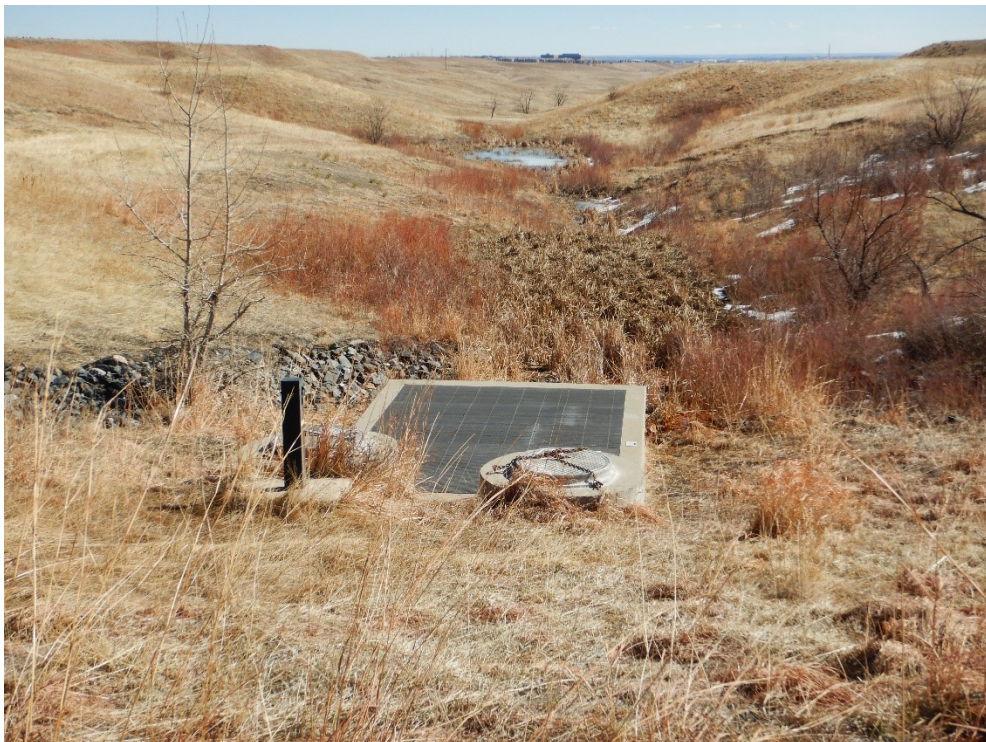
Figure 6. Looking East at the Present Landfill Treatment System. Small amounts of Bio-growth were removed from the North and South Manhole Outlet Pipes, treatment unit outlet pipe, and system outfall using a mechanical pipe cleaner as part of routine preventative maintenance.
