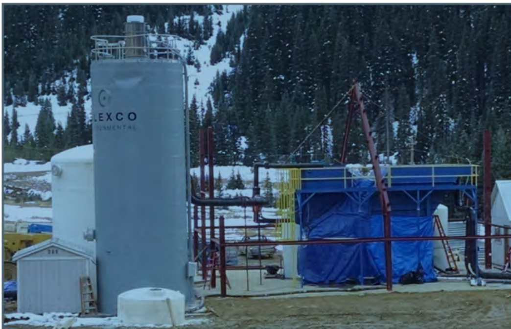
Figure 1 - Left to Right, Reactor Tank, Silo, and Clarifier as the building is being erected in Nov. 2015
