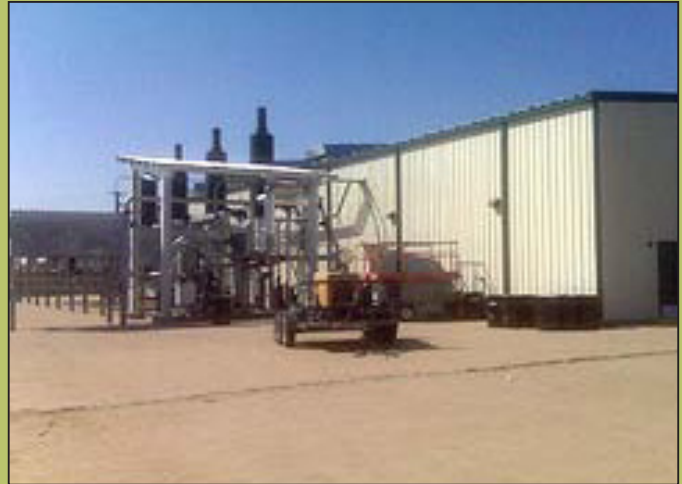
PICTURED: View of the outside of the landfill gas-to-energy plant. (Source: EPA)
