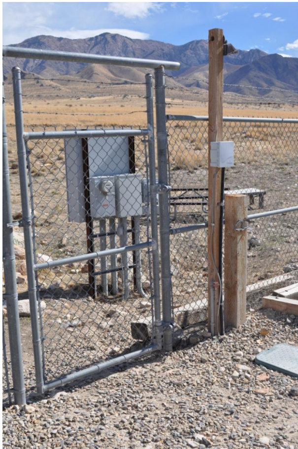
Enclosure gate and electrical panel.
