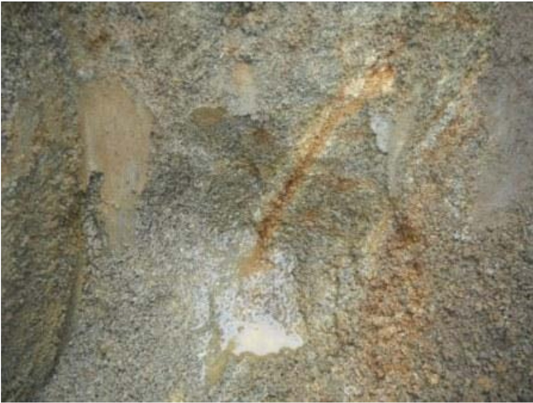
Photo 1 – Seepage from iron-stained fracture in weathered granitic rock.
