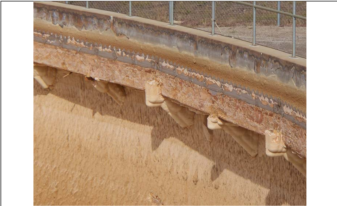
Photo 6. Scale build-up along lip of clarifier overflow.
