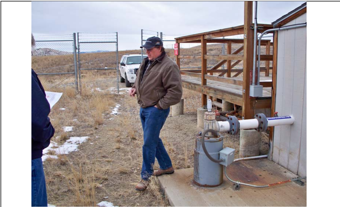
Photo 13. West Camp Pumping Well
