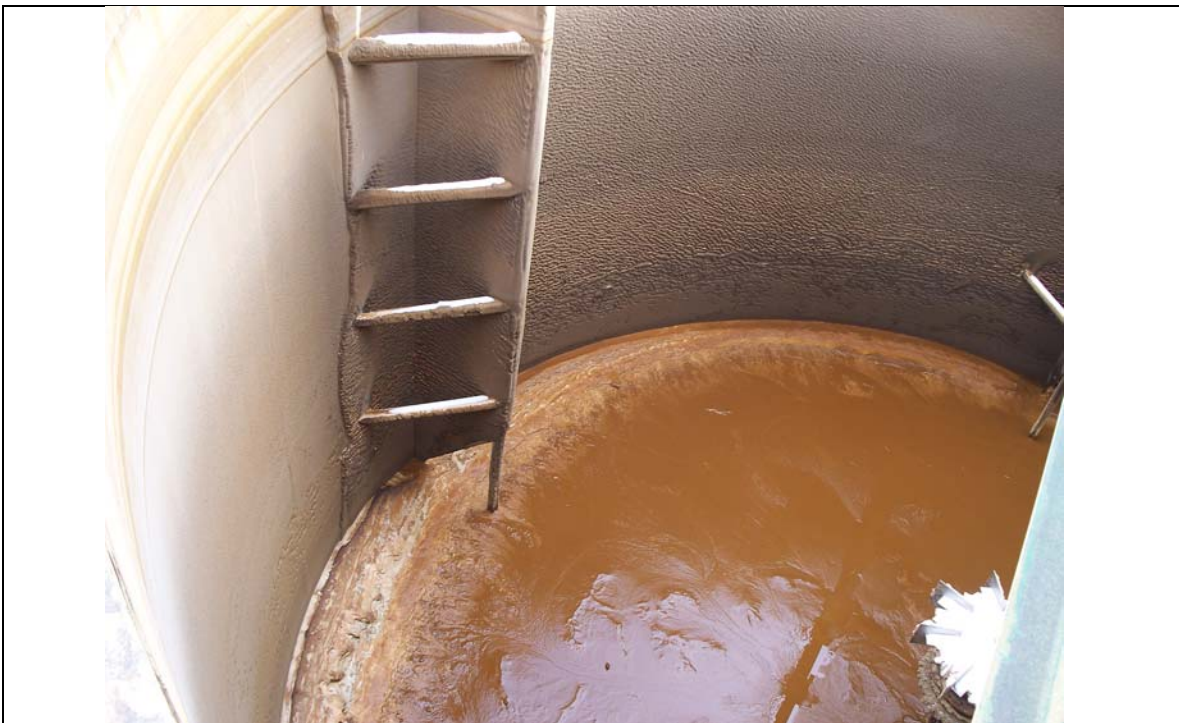
Photo 4. Drained reactor tank, baffle visible (drained for maintenance)
