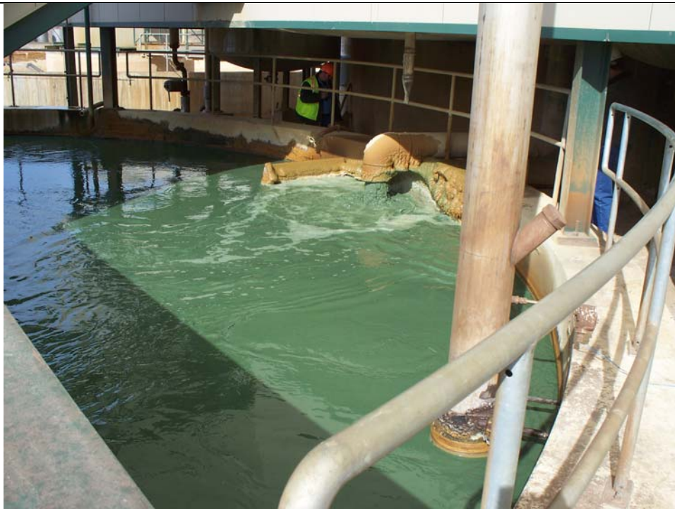
Photo 8. Flow into first stage reactor tank.
