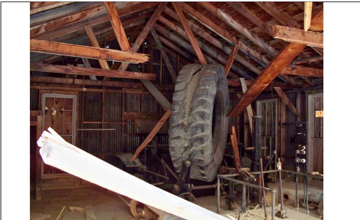
Photo 19. Pilot Butte building interior with vandalism.
