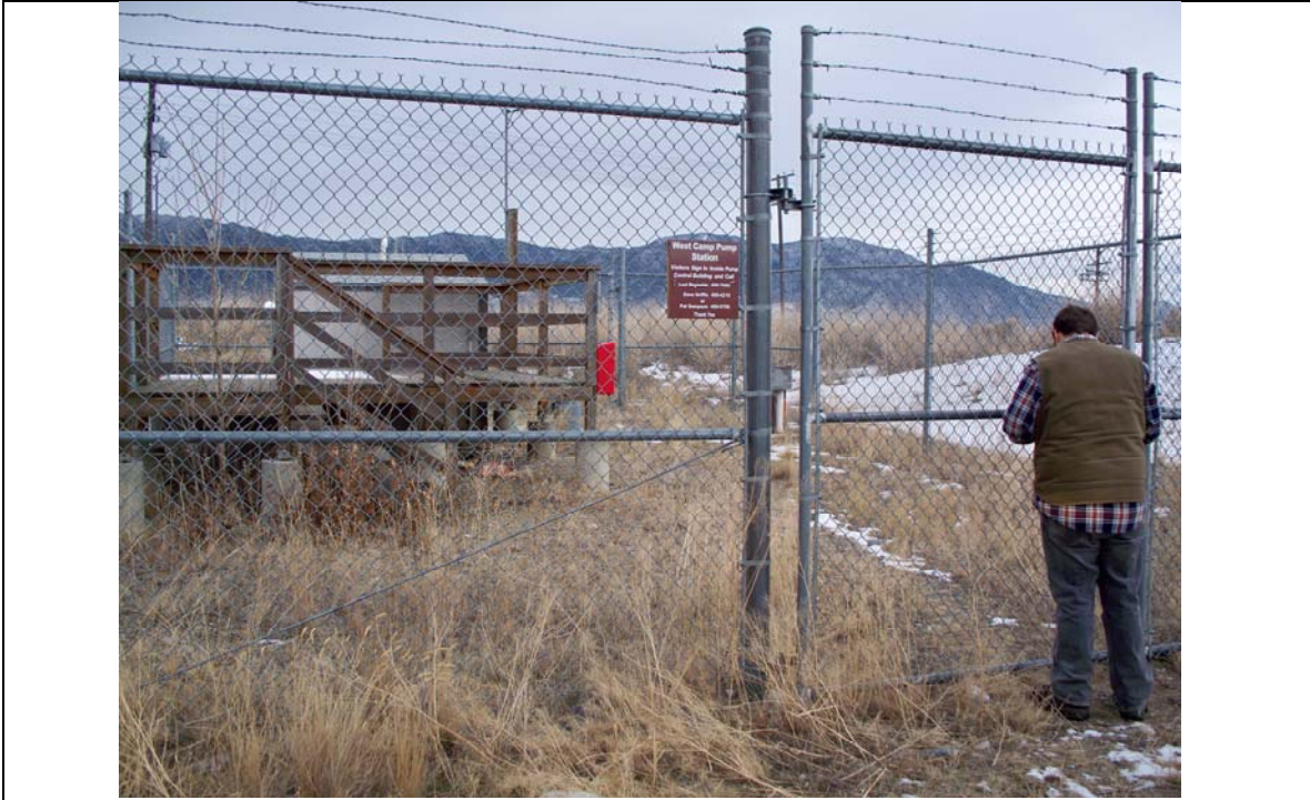
Photo 12. West Camp Pump Station
