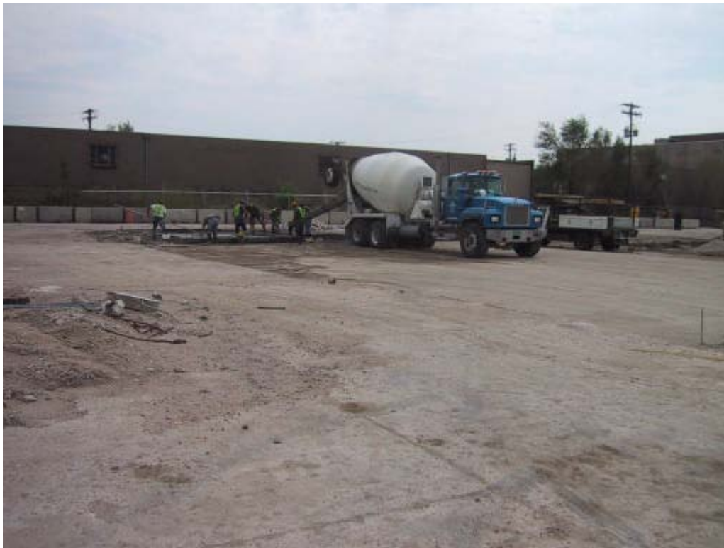
1100 Umatilla Street - formerly DuWald Steel now Atlas Metals. Workers doing site prep work for new pad at Atlas Metals.
