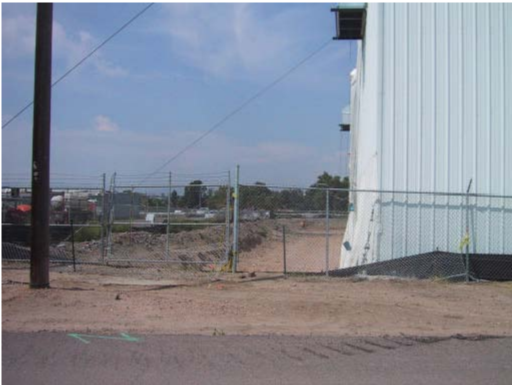
1805 South Bannock Street - Shattuck Chemical Site – Newly excavated monolith location along left edge of photo.
