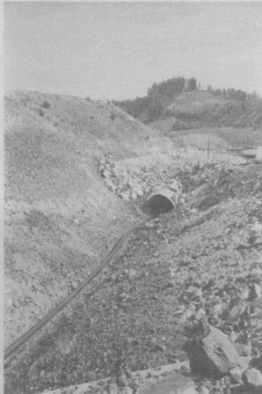
Photo No. 6 Pipeline Conveying ARD Seep Discharge above Pond C View to North
