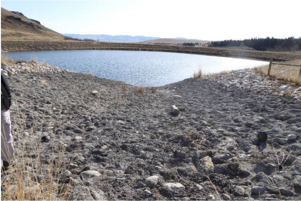
Supplemental Stormwater Control (OU04 RDU-3)
