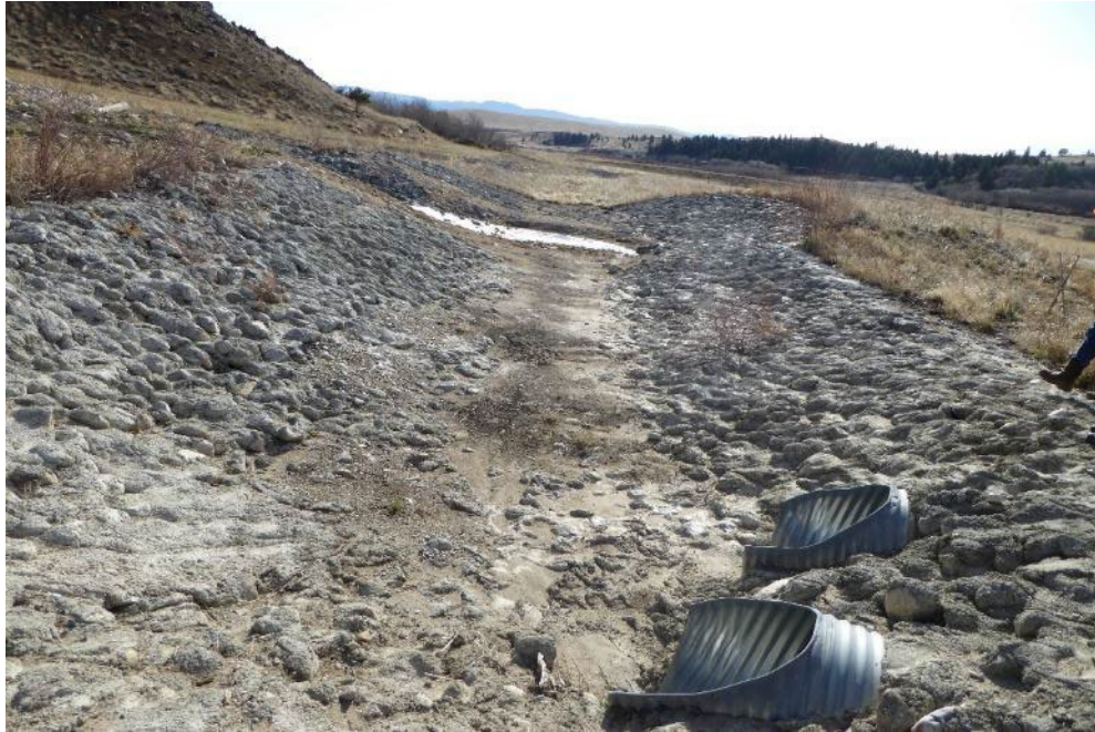
Surface water diversion structure pipes (OU4, RDU-3)
